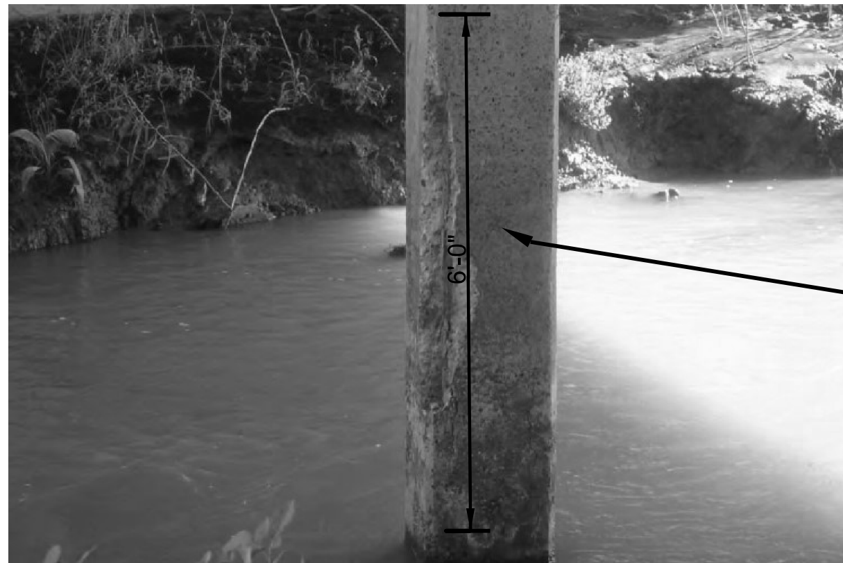
REPAIR 6 NBI: 21-109-0-1804-01-002 BENTS 2 & 3 FRACTURES IN PILES
