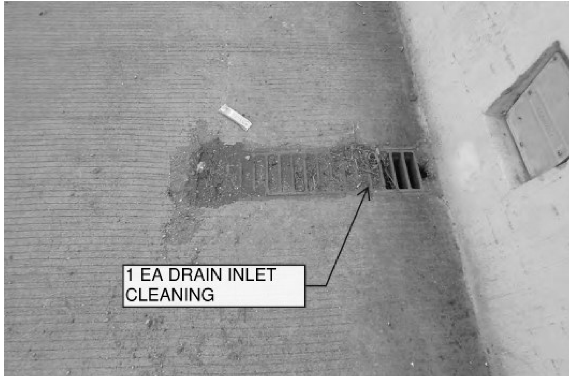
NBI: 21-031-0-0039-16-170 TYPICAL CLOGGED DECK DRAIN ALONG SHOULDERS
