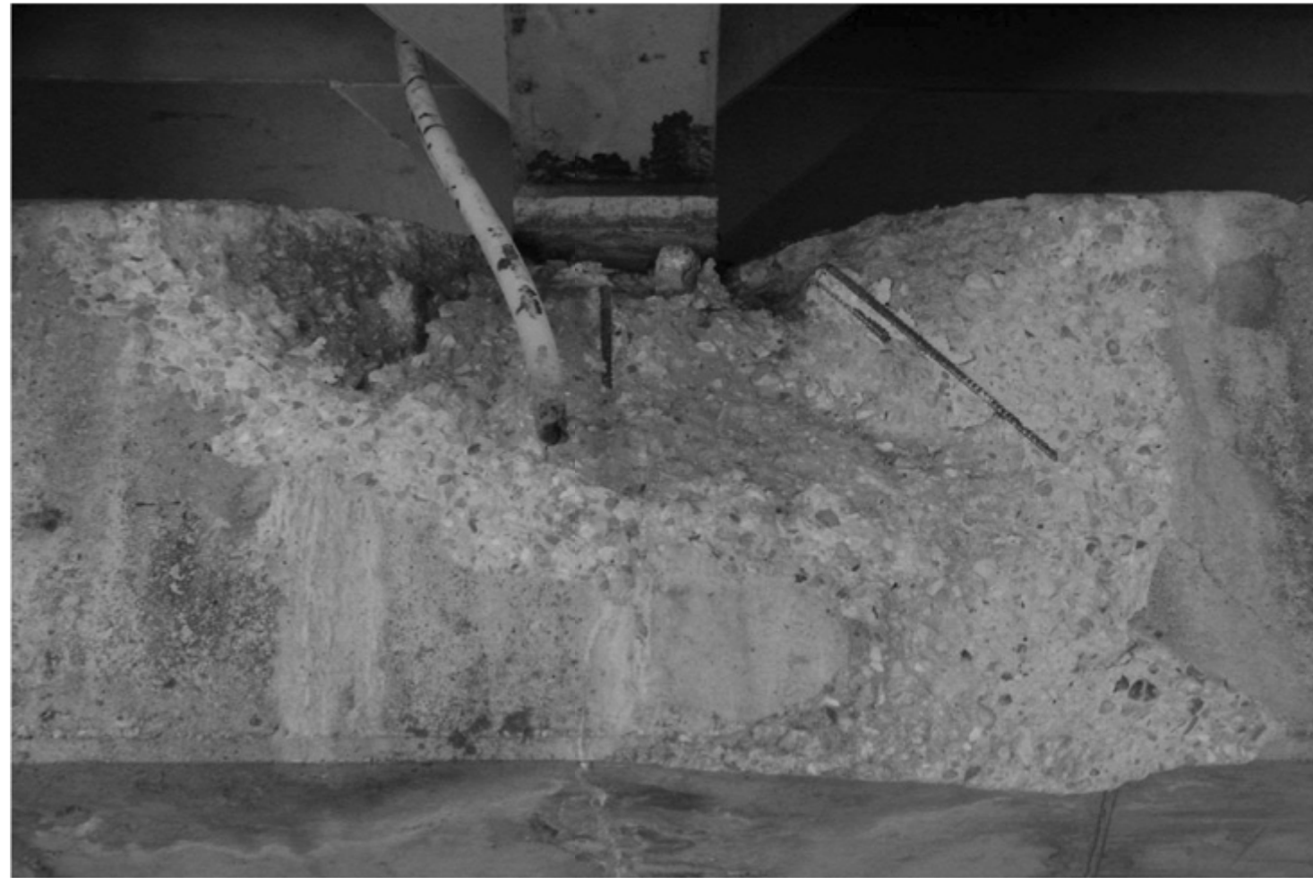
PHOTO 1. - SPALLING OF PIER CAP 3, LOOKING NORTH.
