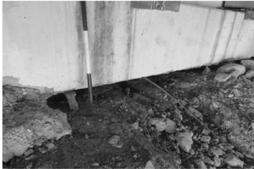
PHOTO 1. - UNDERMINED NORTHWEST ABUTMENT CAP, LOOKING NORTH.
