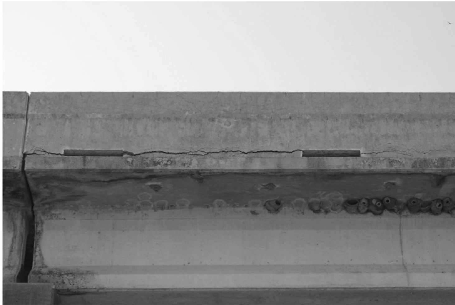
PHOTO 1. - CRACK IN NORTHWEST BRIDGE RAIL IN SPAN 10, LOOKING SOUTHEAST.
