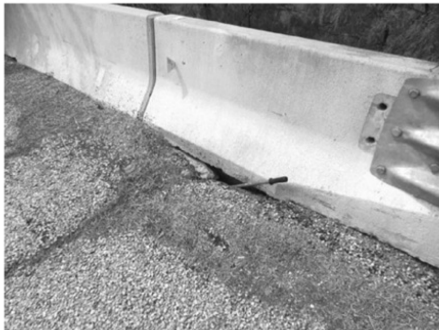
PHOTO 3. - EROSION VOID IN NORTHWEST APPROACH, LOOKING SOUTH.
