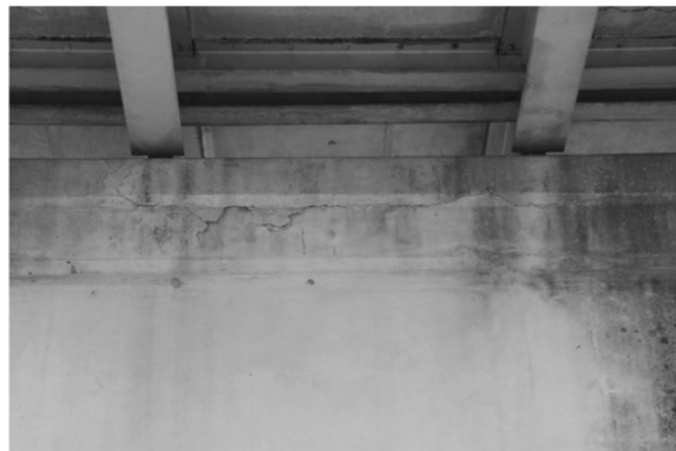
PHOTO 1. - DELAMINATION IN PIER CAP AT BENT 3, LOOKING WEST.
