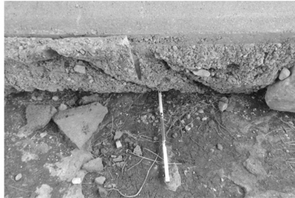
PHOTO 2. - EXPOSED AND UNDERMINED SOUTHWEST RIPRAP, LOOKING WEST.
