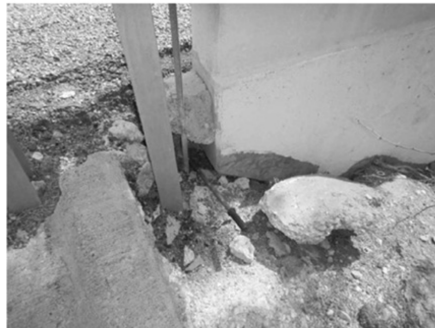
PHOTO 4. - EROSION VOID AT NORTH AND WEST CORNER WINGWALL. WEST CORNER SHOWN, LOOKING EAST.
