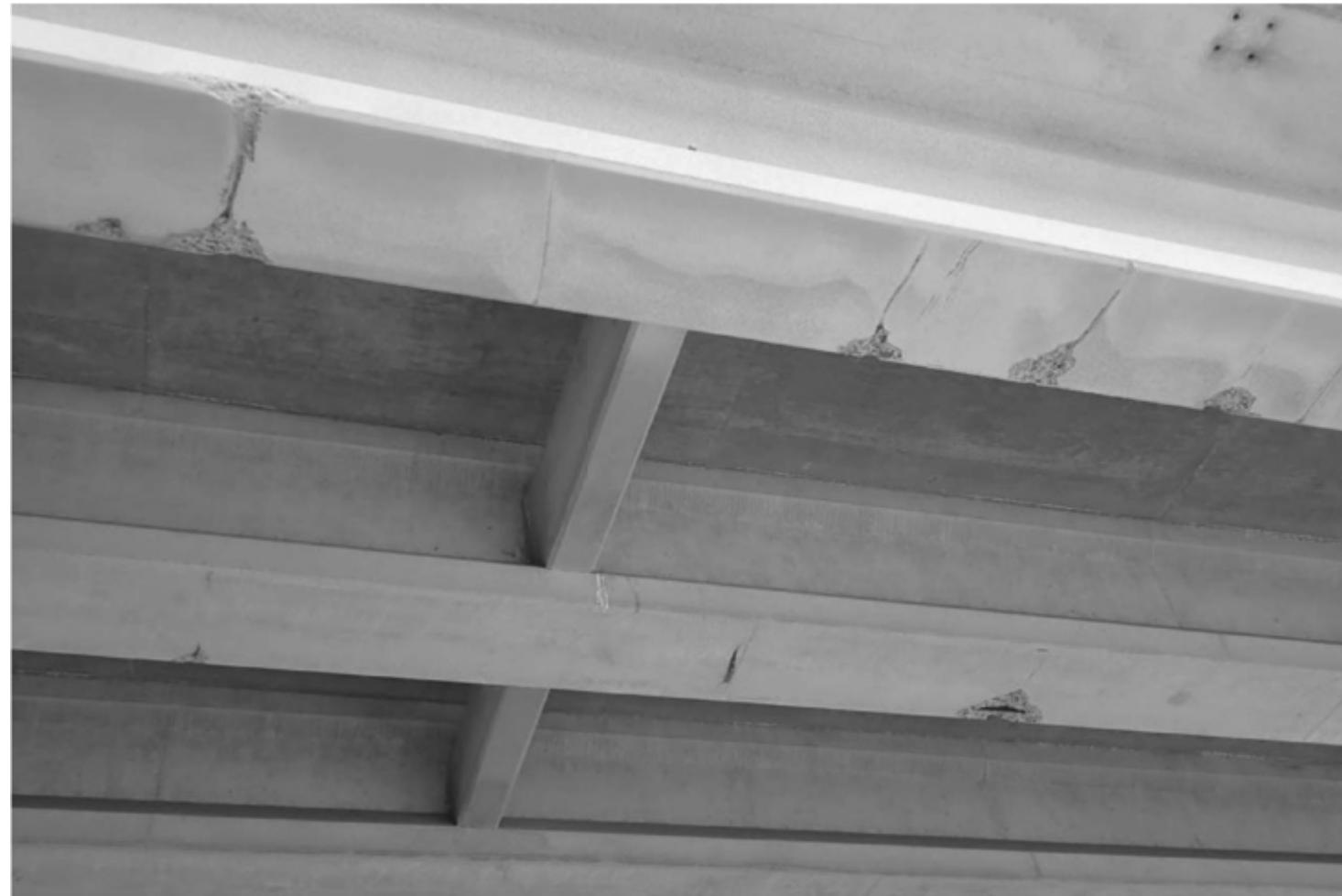
PHOTO 1. - OVERHEIGHT IMPACT SPALL OF BEAM 2 OF SPAN 2, LOOKING NORTH.
