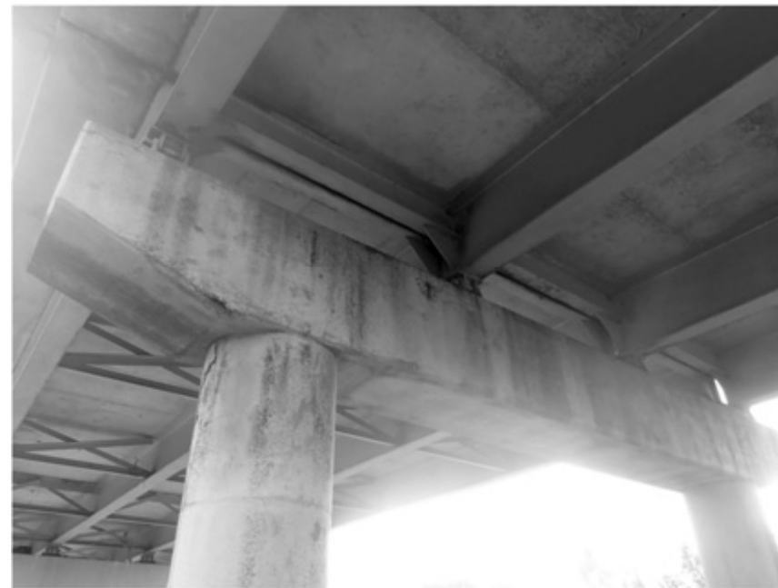
PHOTO 4. - HORIZONTAL CRACKS IN CAP AT BENT 4 FROM SOUTHWEST, LOOKING SOUTHWEST.
