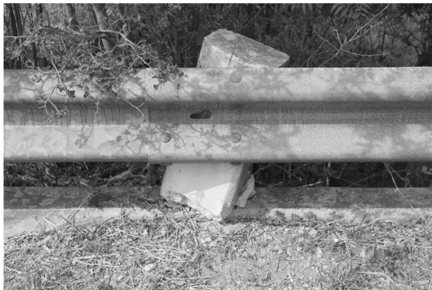
PHOTO 1. - DAMAGED CONCRETE POST AT NORTHWEST WINGWALL, LOOKING NORTH.
