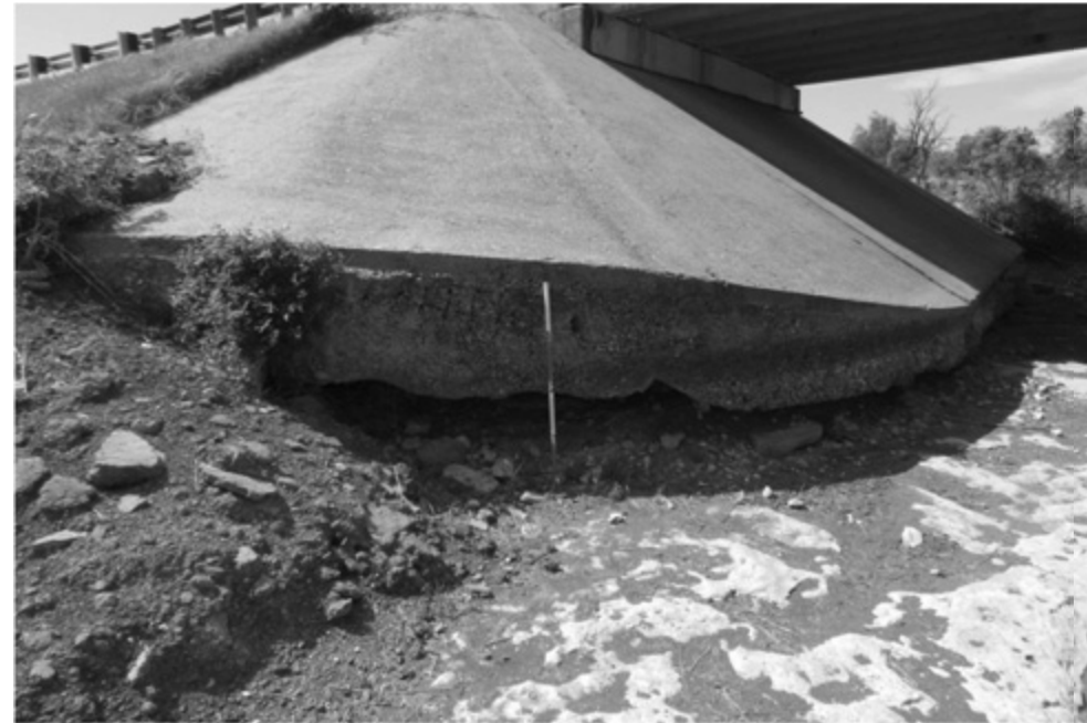
PHOTO 1. - EXPOSED AND UNDERMINED SOUTHWEST RIPRAP, LOOKING NORTHWEST.
