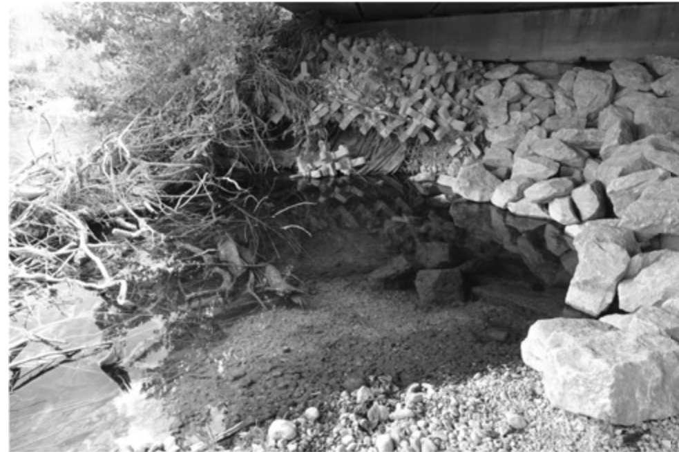
PHOTO 1. - CHANNEL BED SCOUR HOLE UNDER SPAN 11, LOOKING SOUTHWEST.
