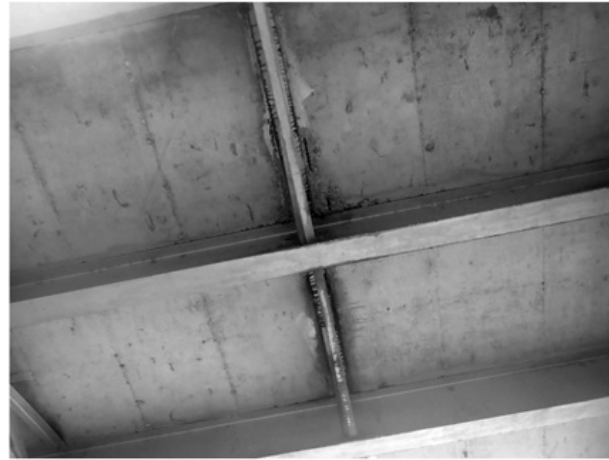
PHOTO 2. - TYPICAL DELAMINATION AND SPALLS OF DECK UNDERSIDE, COMMON ALONG THE DIAPHRAMS BELOW CONSTRUCTION JOINTS.
