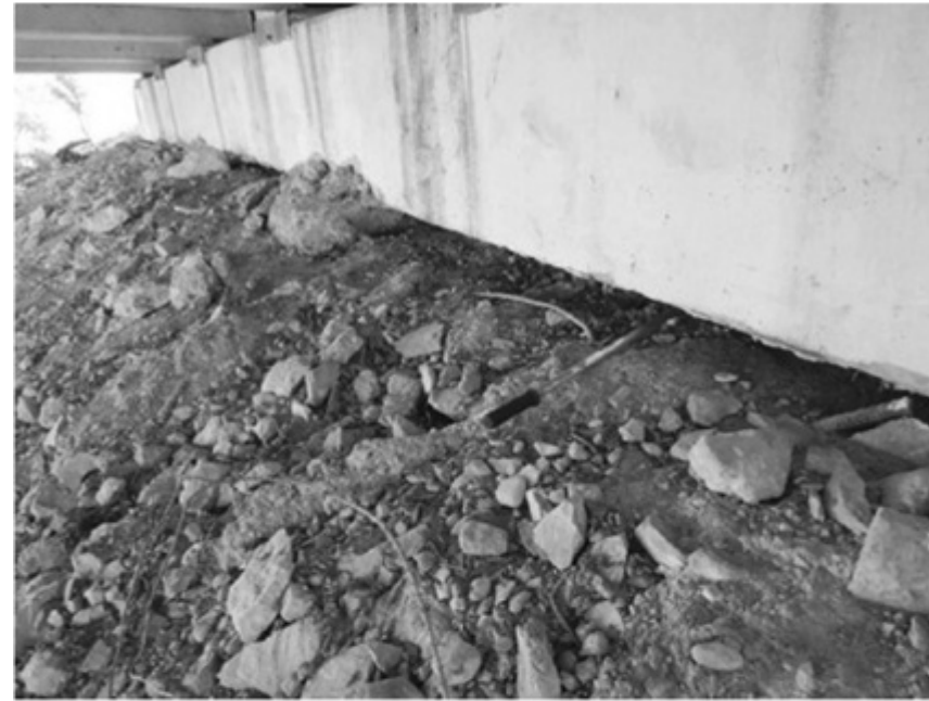
PHOTO 2. - UNDERMINED NORTHWEST ABUTMENT CAP, LOOKING WEST.
