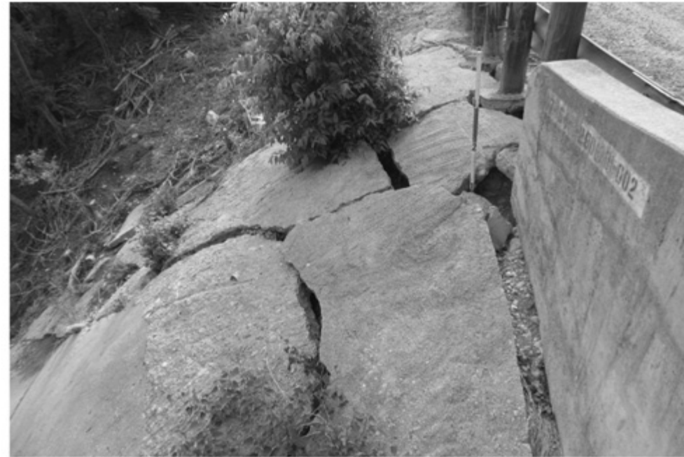
PHOTO 2. - DETERIORATION OF SOUTHWEST RIPRAP, LOOKING WEST.
