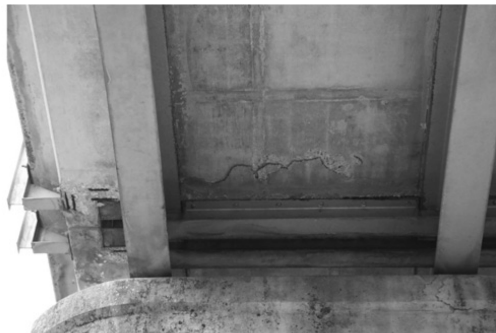
PHOTO 2. - DELAMINATION AND SPALLING IN UNDERSIDE OF DECK OVER BENT 3, LOOKING WEST.
