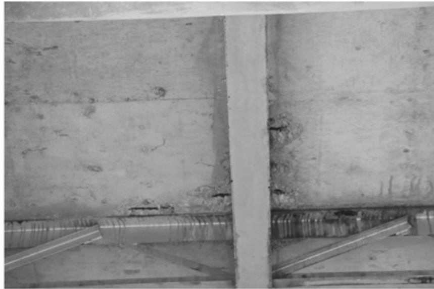
PHOTO 1. - SPALLS IN DECK SOFFIT IN SPAN 1 FROM SOUTHWEST, LOOKING SOUTHWEST.
