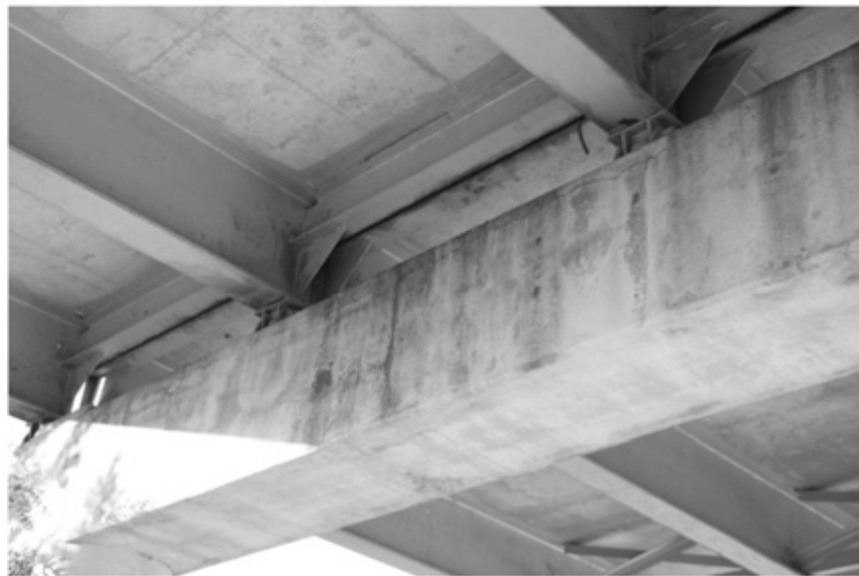
PHOTO 3. - HORIZONTAL CRACKS IN CAP AT BENT 4 FROM SOUTHWEST, LOOKING NORTH.
