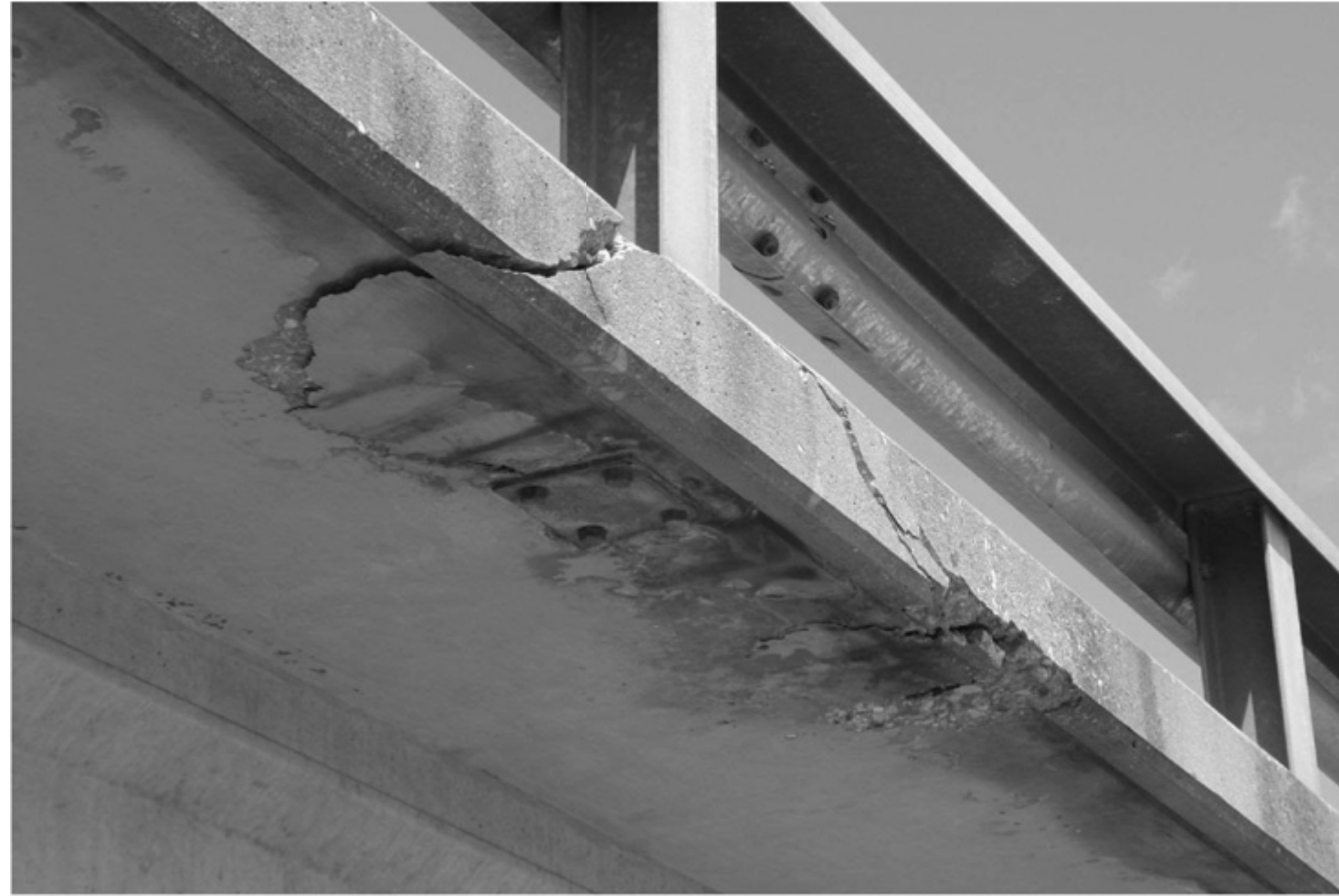
PHOTO 1. - NORTHEAST DECK OVERHANG IN SPAN 1 FROM THE SOUTH SPALLING, LOOKING WEST.
