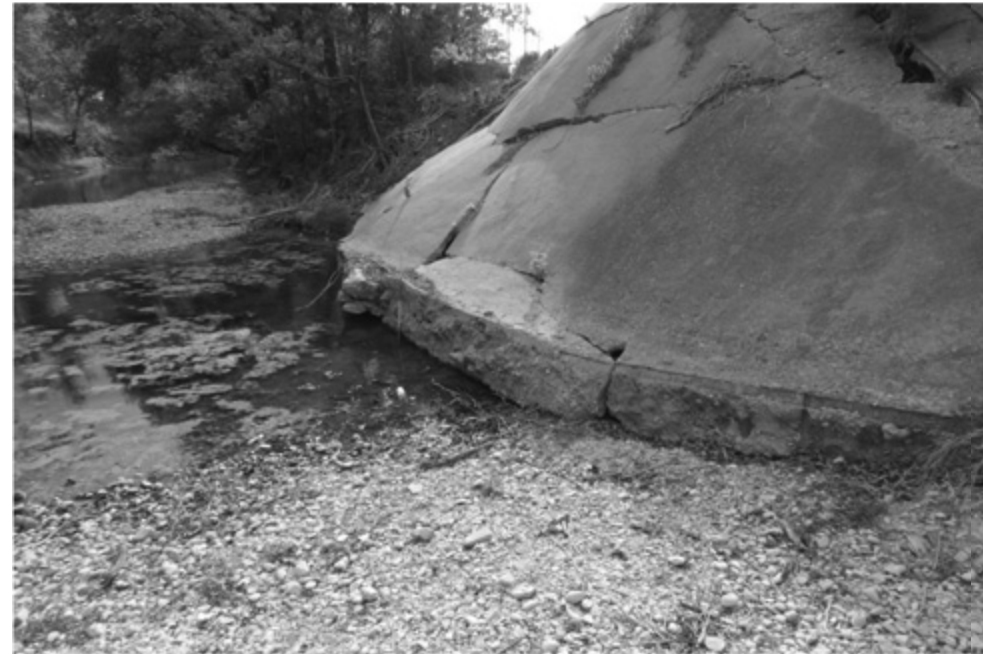
PHOTO 1. - DETERIORATION OF SOUTHWEST RIPRAP, LOOKING NORTHWEST.
