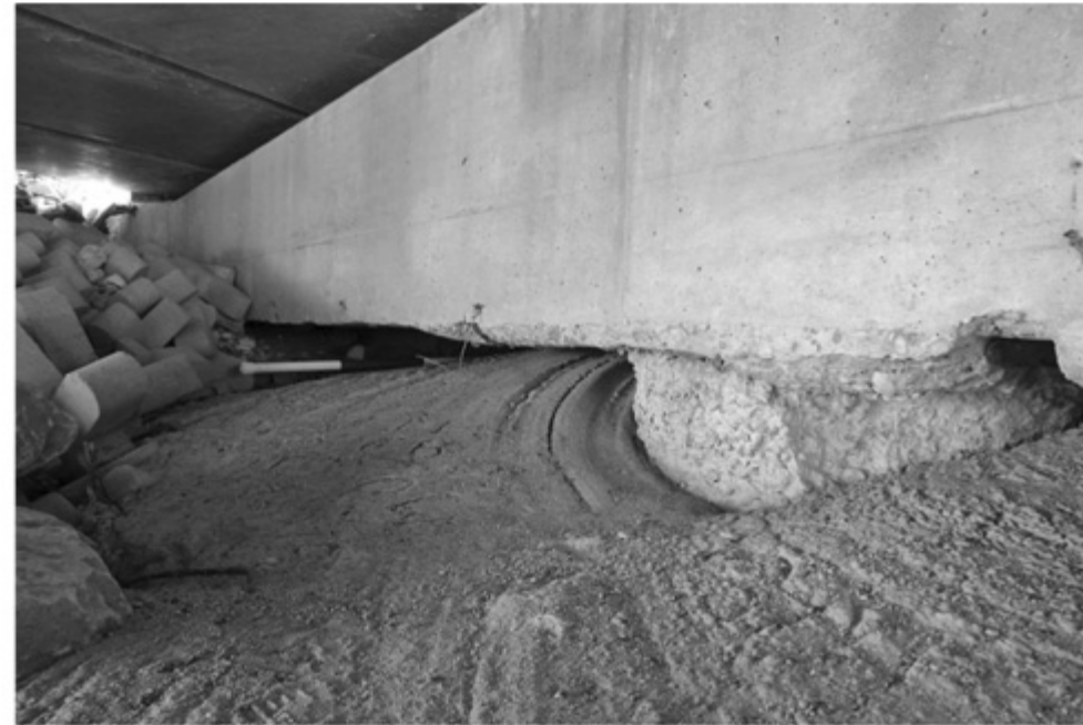
PHOTO 2. - UNDERMINED SOUTHWEST ABUTMENT, LOOKING SOUTH.
