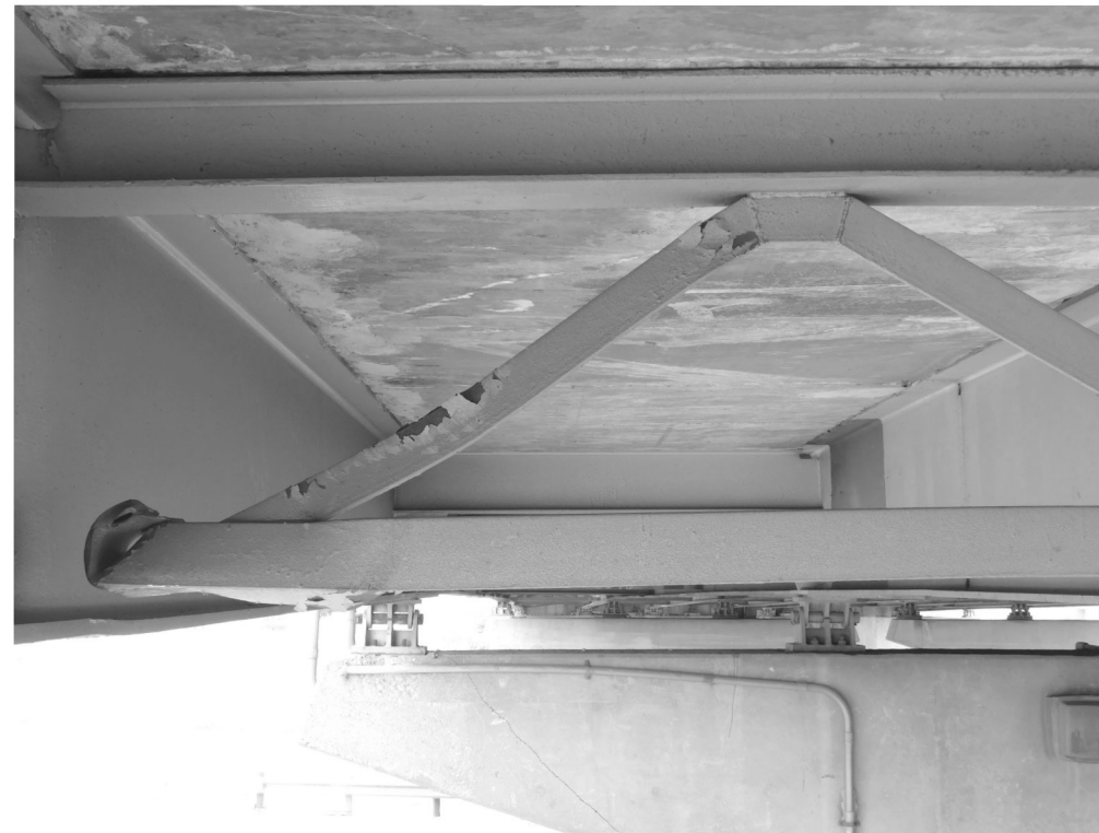
SP3 - Damaged diaphragm members and broken connection to beam A. Third diaphragm from Pier 2.
