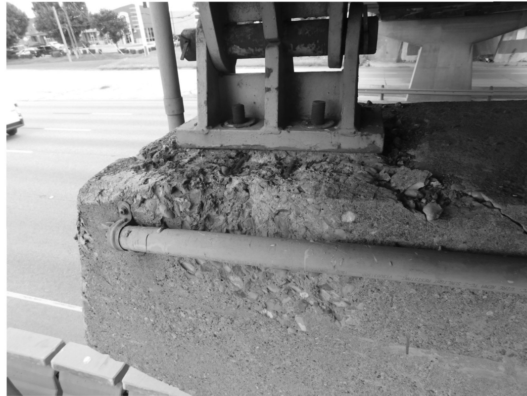
SB3 - Spall on Pier 3 under Beam A bearing
