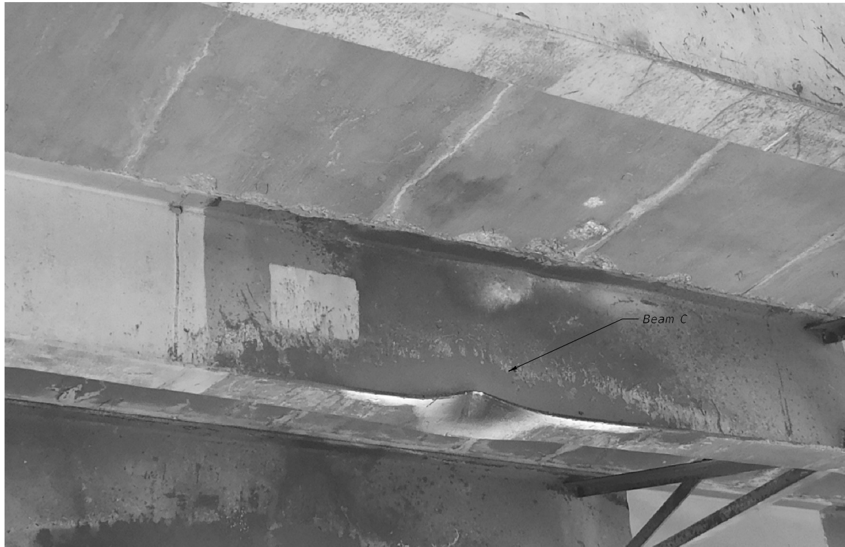
SP4 - Impact damage on Beam C with web and flange deformation
