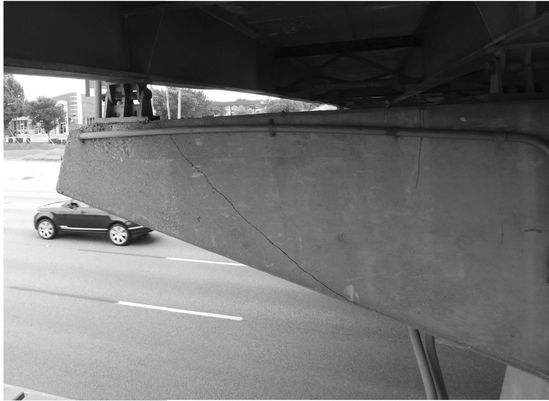
SB1 & SB2 - Crack along face of Pier 3 Cap
