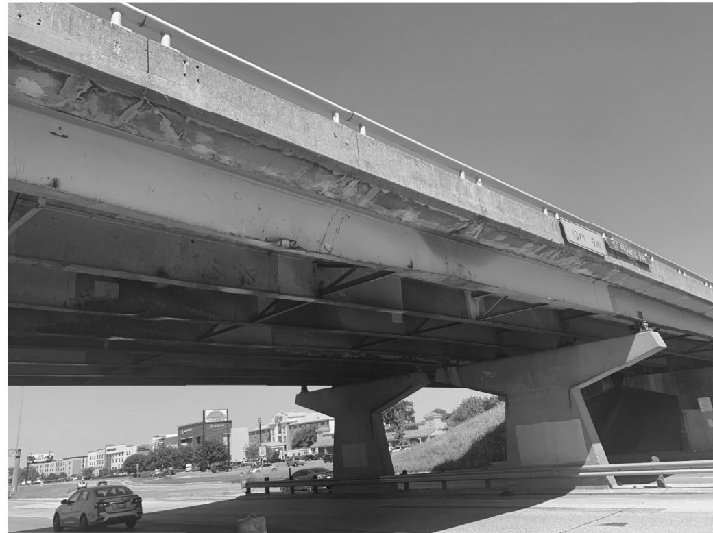
SP1 - Impact damage along Beam A with significant web and flange deformation
