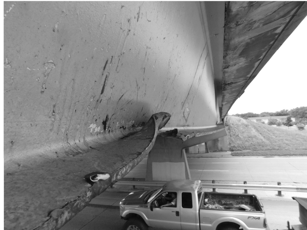
SP1 - Impact damage along Beam A with significant web and flange deformation
