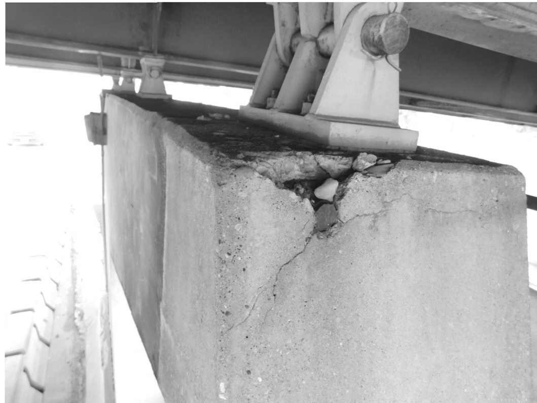
SB4 - Spall on Pier 3 under Beam D bearing
