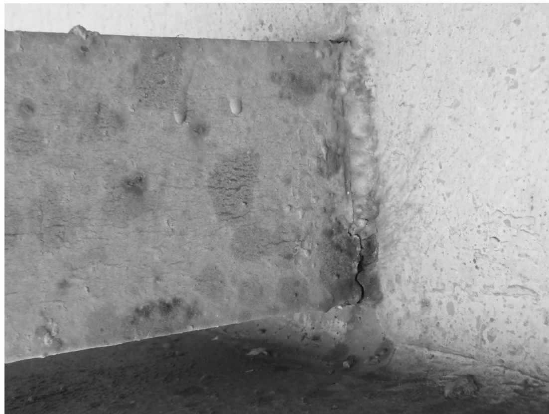
SP6 - Crack on the welded bottom connection between the second diaphragm from Pier 2 and Beam C
