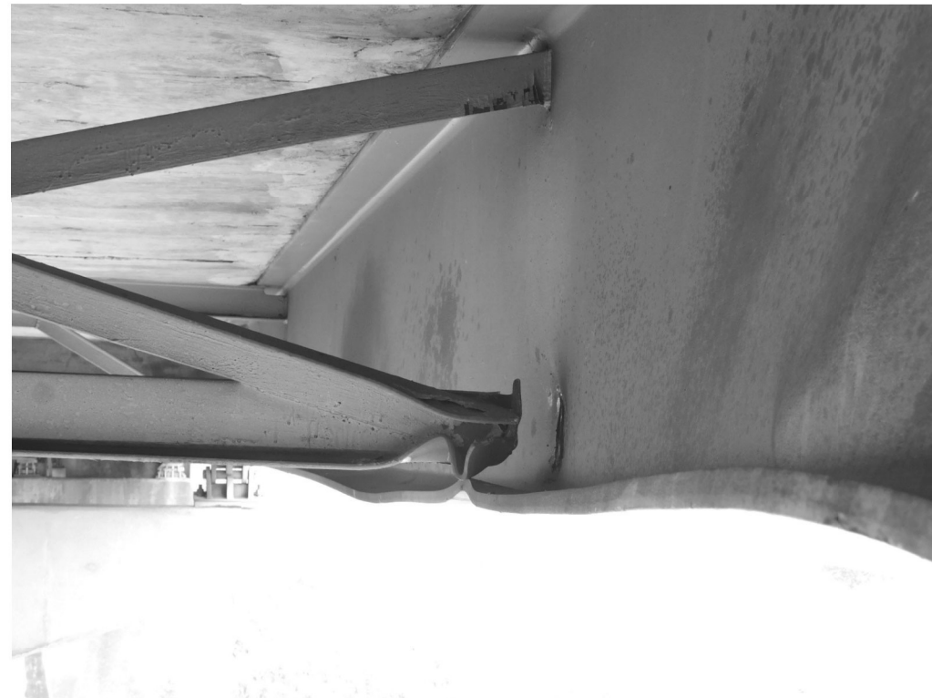
SP2 - Damaged diaphragm members and broken connection to beam A. Second diaphragm from Pier 2.
