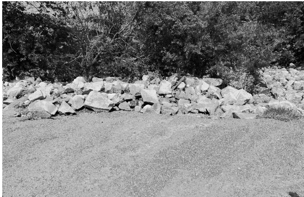
PICTURE 3 (DOWNSTREAM) ASPHALT TO REMOVE WASHED EXISTING STONE RIPRAP
