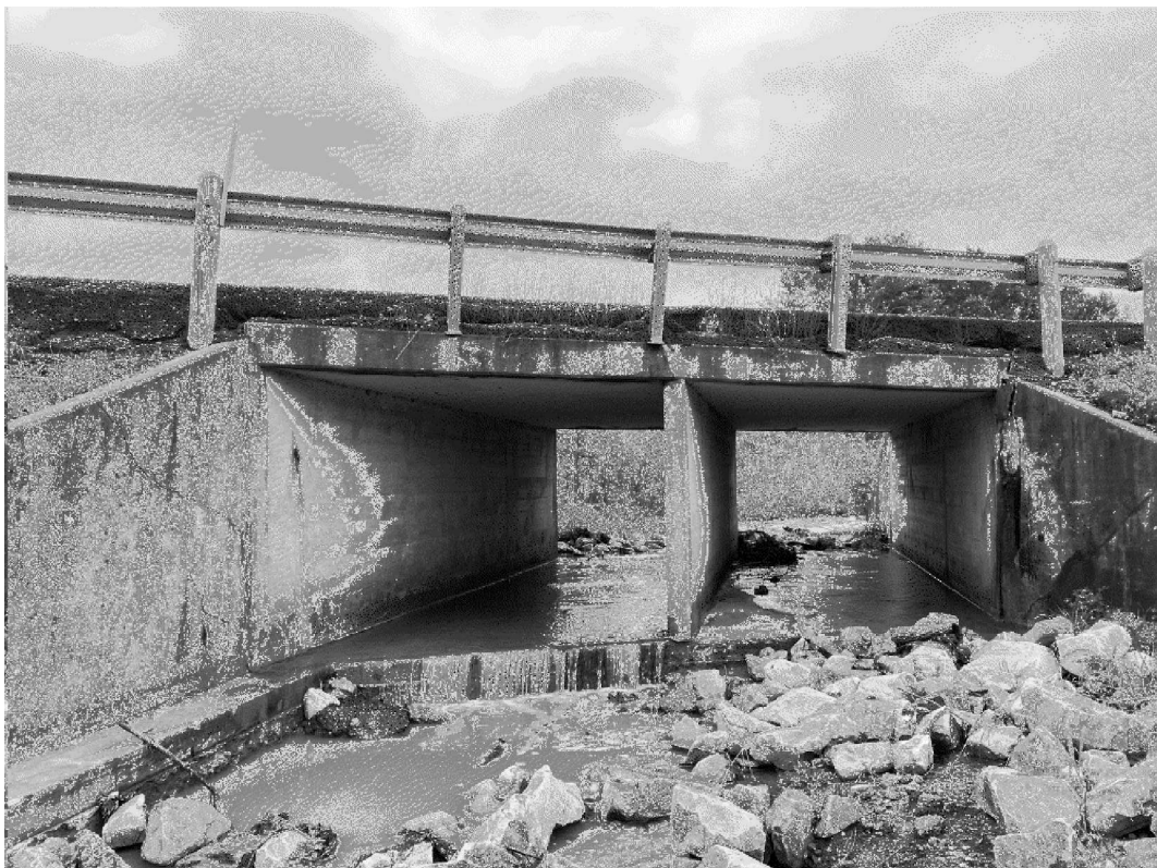
PICTURE 1 (DOWNSTREAM) SCOUR AT CHANNEL BED
