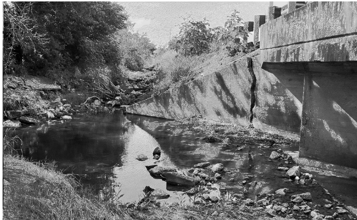
PICTURE 2 (UPSTREAM) CHANNEL BED AND CULVERT FOOTING ERODED STONE RIPRAP WASHED AWAY
