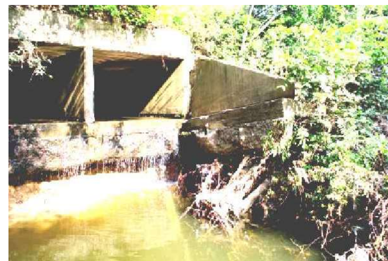
PHOTO 3 UNDERMINING OF NE WINGWALL - Looking North
