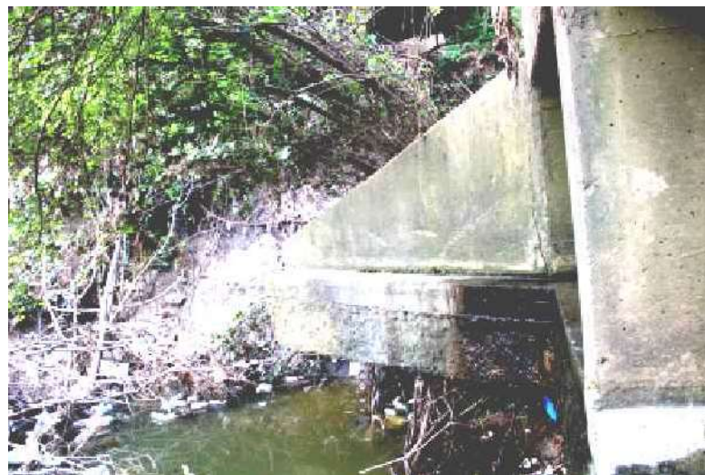
PHOTO 2 UNDERMINING OF SE WINGWALL - Looking South
