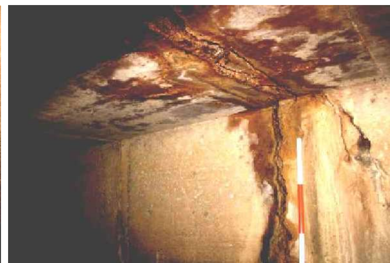
PHOTO 6 FRACTURE AT NORTH ABUTMENT - Looking NW
