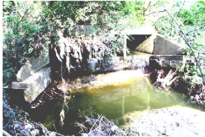
PHOTO 1 SCOUR AT CULVERT OUTLET - Looking NW
