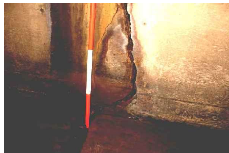
PHOTO 5 CLOSE-UP OF CRACK AT MIDDLE BOX - Looking SE
