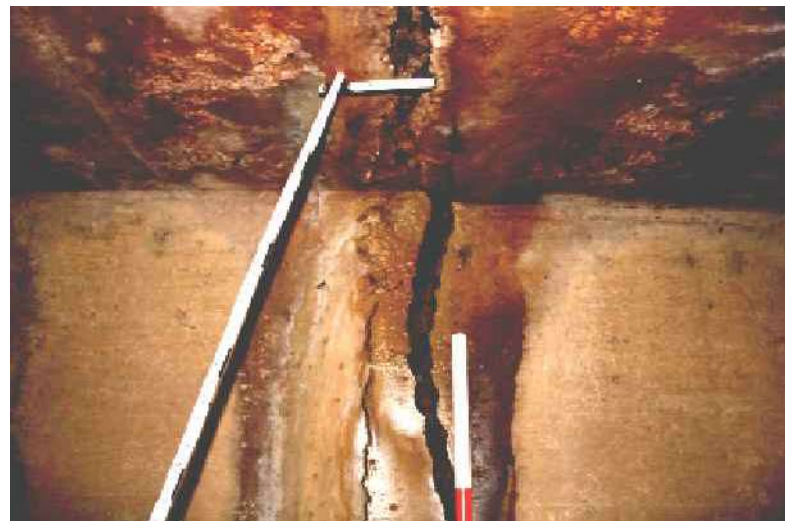
PHOTO 4 FRACTURE IN NORTH BOX - Looking South
