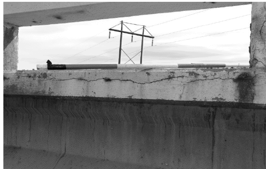
TYPICAL CRACKING AT DECK EDGE AND RAIL POSTS
