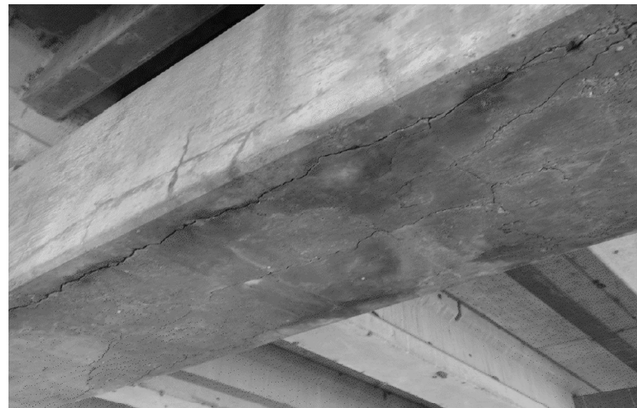
TYPICAL CRACKING ON BENT CAPS.
