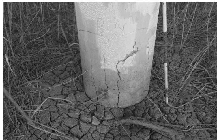
BENT 24 CENTER COLUMN. SOUND AND REMOVE ALL LOOSE MATERIAL. PERFORM CONCRETE PATCHING. WRAP COLUMN WITH CFRP SINGLE LAYER, 5 FT FROM BASE UP.
