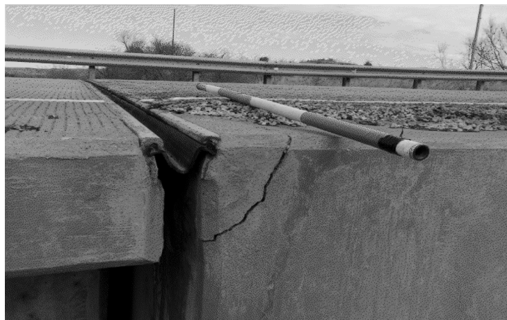
CRACK ON NORTHEAST BACKWALL. PERFORM CONCRETE PATCHING.
