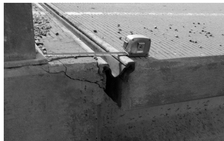
CRACK ON NORTHWEST BACKWALL. PERFORM CONCRETE PATCHING.
