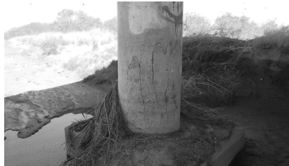
BENT 5 WEST COLUMN. SOUND AND REMOVE ALL LOOSE MATERIAL. PERFORM CONCRETE PATCHING. WRAP COLUMN WITH CFRP SINGLE LAYER, 5 FT FROM BASE UP.
