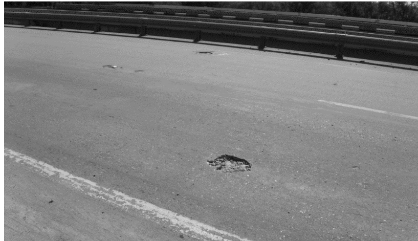
ISOLATED SPALLS ON DECK
