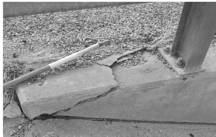
SPALL ON NORTHEAST WINGWALL. PERFORM PATCHING.
