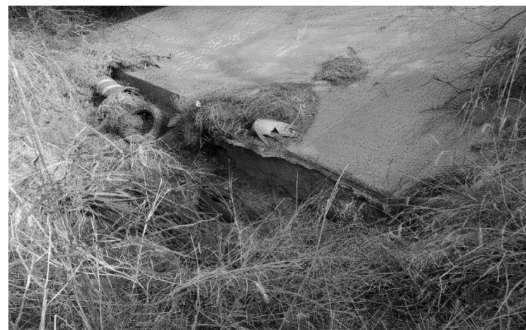
EROSION AT NORTHWEST ABUTMENT. INSTALL STONE PROTECTION.
