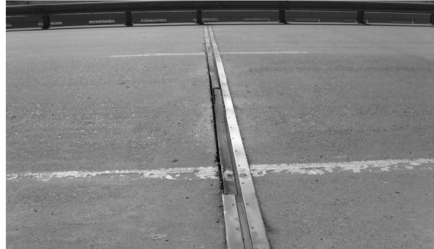
DAMAGED ARMOR JOINT
