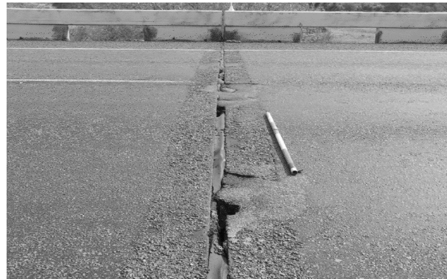
TYPICAL FAILED JOINT SEAL WITH DAMAGED HEADER MATERIAL.
