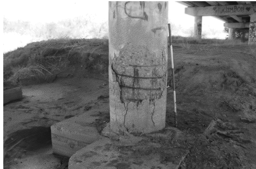
BENT 5 CENTER COLUMN. SOUND AND REMOVE ALL LOOSE MATERIAL. PERFORM CONCRETE PATCHING. WRAP COLUMN WITH CFRP SINGLE LAYER, 5 FT FROM BASE UP.
