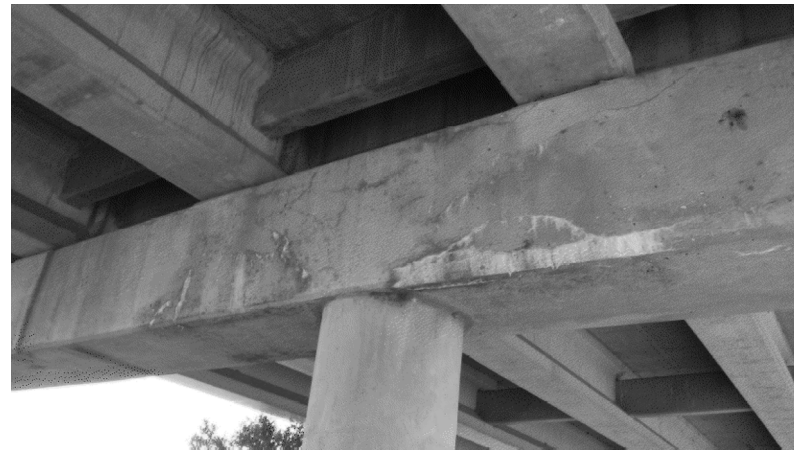
TYPICAL CRACKING ON BENT CAPS. SOUND AND REMOVE LOOSE MATERIAL. PERFORM STRUCTURAL PATCHING.
