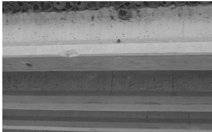
SPALL ON NORTHWEST GIRDER IN SPAN #3 PERFORM OVERHEAD PATCHING.
