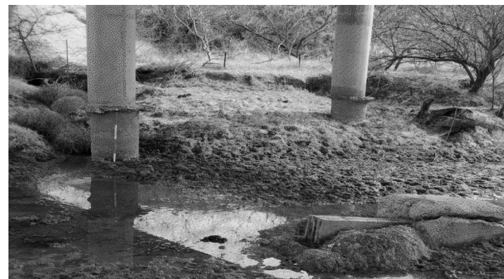
SCOUR AT BENT #8. INSTALL STONE PROTECTION.
