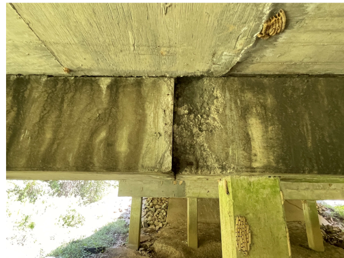
ALLEY CREEK SPALL REPAIR DETAIL LOCATION FOR SPALL REPAIR AT BENT 5 CAP (APPOX. STA. 382+16.80) OR AS DIRECTED BY THE ENGINEER
