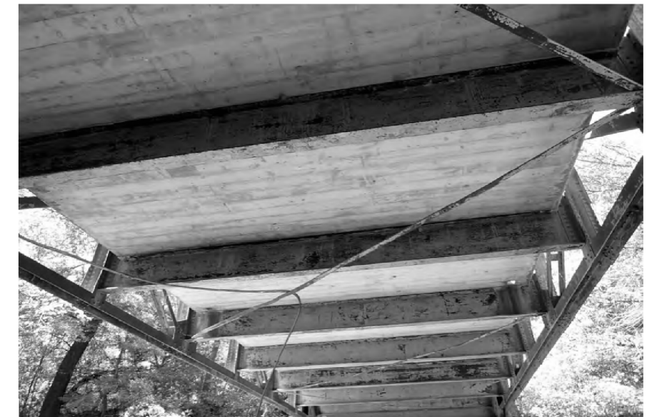
Superstructure View looking South: Lateral bracing bars missing, detached, or sagging. Replace bracing bars is estimated at three. Estimated size is (3/8" X 3" flat strap: 3.825 lbs/ft) X 24'. Dimensions to be field verified.
