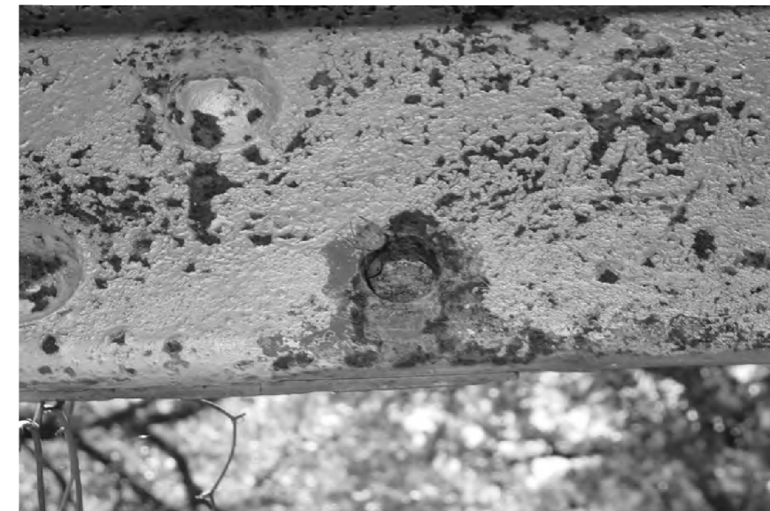
East Truss L2 Looking North: Missing rivet in bottom row of outboard gusset plate. Replace rivet.
