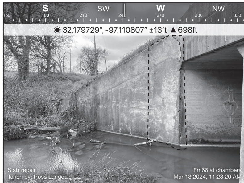
SOUTH WEST WINGWALL SHOWING LIMITS OF CONC STR REPAIR
