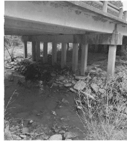
TYPICAL EROSION (M2) PHOTOS
