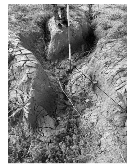
① EROSION GULLY TYPICAL
