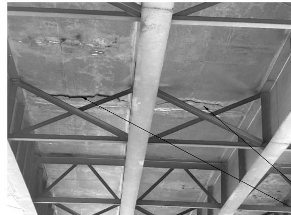
① DECK SOFFIT DELAMINATION
