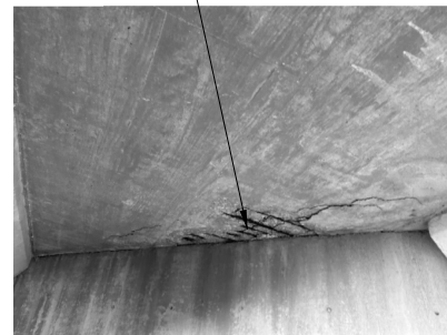
⑤ DECK SOFFIT DELAMINATION
