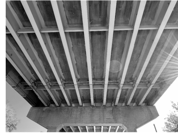
① SPAN 6, CRACKING AND SPALLING ON DIAPHRAGMS 1N, 2N, 3N, 4N, 5N, 6N, 7N, 8N, 9N, AND 10N AT EAST END OF SUSPENDED SPAN
