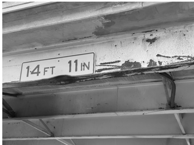
① ② IMPACT DAMAGE ON NORTH FASCIA BEAM
