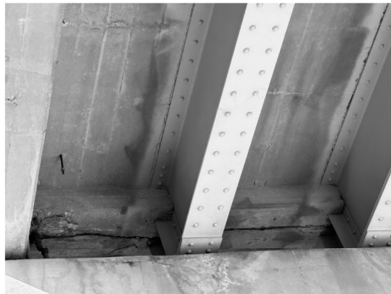
① CRACKING AND SPALLING ON DIAPHRAGM 10N AT BENT 6
