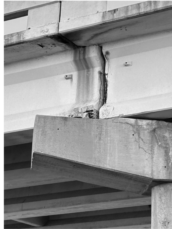
① TYPICAL BEAM END THAT REQUIRES REPAIR AT BENT. SEE BEAM REPAIR TABLE FOR LOCATION AND QUANTITY.
