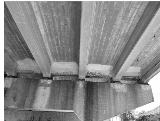
① CRACKING AND SPALLING ON DIAPHRAGMS 5N, 6N, 7N, 8N ON WEST SIDE OF BENT 3
