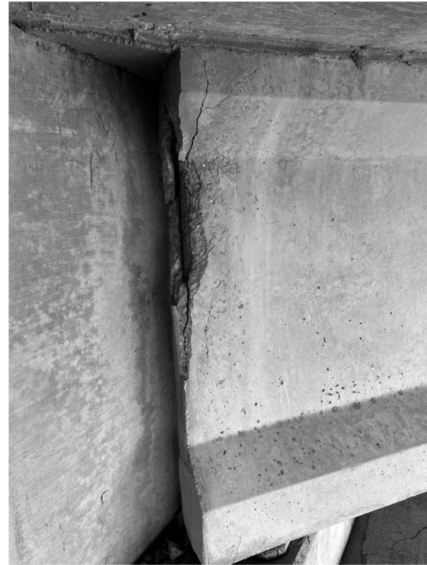
① TYPICAL BEAM END THAT REQUIRES REPAIR AT ABUTMENT. SEE BEAM REPAIR TABLE FOR LOCATION AND QUANTITY.
