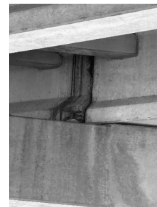
④ TYPICAL BEAM END THAT REQUIRES REPAIR AT BENT (SEE BEAM REPAIR TABLE FOR LOCATION AND QUANTITY)
