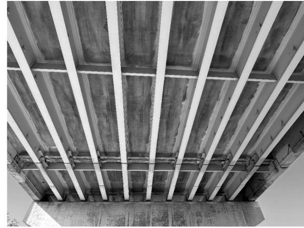
① SPAN 6, CRACKING AND SPALLING ON DIAPHRAGMS 2N, 3N, 4N, 8N, AND 9N AT WEST END OF SUSPENDED SPAN
