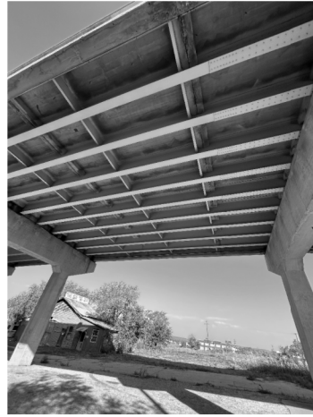
① CRACKING AND SPALLING ON DIAPHRAGMS 1N AND 10N AT BOTH EAST AND WEST CONCRETE DIAPHRAGM LINES, SPAN 7 LOOKING NORTH
