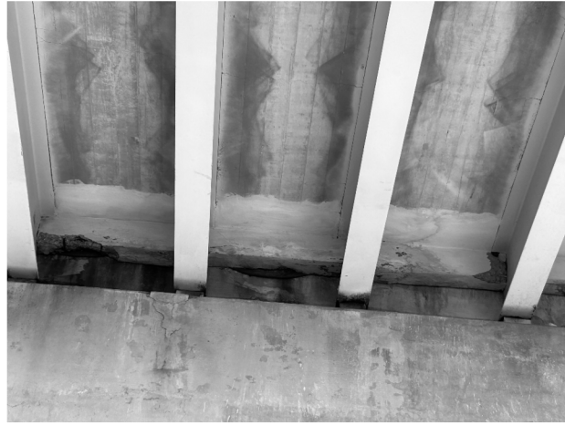
① CRACKING AND SPALLING ON DIAPHRAGMS 6N, 7N, AND 8N ON EAST SIDE OF BENT 8
