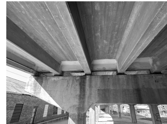
① CRACKING AND SPALLING ON DIAPHRAGMS 5N, 6N, 7N, 8N ON EAST SIDE OF BENT 3
