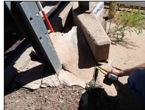
TYPICAL RIPRAP DAMAGE AT WINGWALL (Showing Abutment 4 from SH 207 SB Overpass at SH 136 WB)
