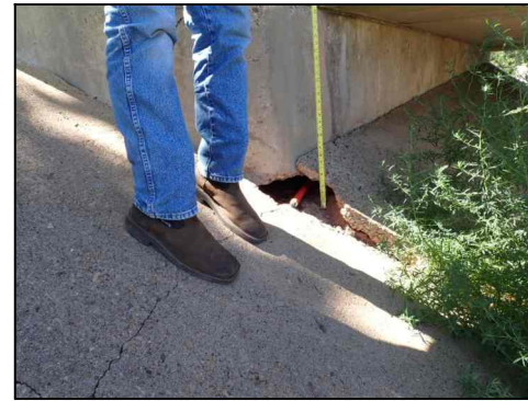
TYPICAL RIPRAP DAMAGE AT ABUTMENT (Showing Abutment 1 from SH 207 NB Overpass at SH 136 WB)
