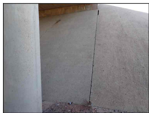
TYPICAL OPEN RIPRAP CONSTRUCTION JOINT (Showing Abutment 1 from SH 207 SB Overpass at SH 136 EB)
