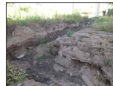
TYPICAL EROSION GULLY (Showing South of Bent 2 from IH 27 SB Over P.D.T. Fork Red River)
