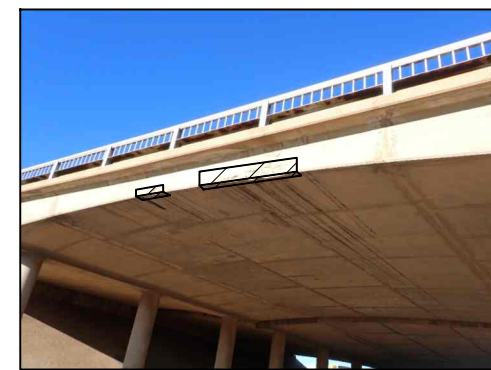
TYPICAL SUPERSTRUCTURE ARCH DAMAGE (Showing Span 2 from SH 207 NB Overpass at SH 136 EB)
