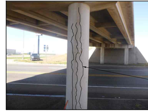
TYPICAL COLUMN SPLIT CRACKING (Showing Bent 3 Column 1 from IH 40 EB Overpass at US 385)
