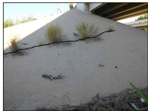
TYPICAL RIPRAP CRACKING (Showing Abutment 1 from IH 27 SB at P.D.T. Ford Red River)
