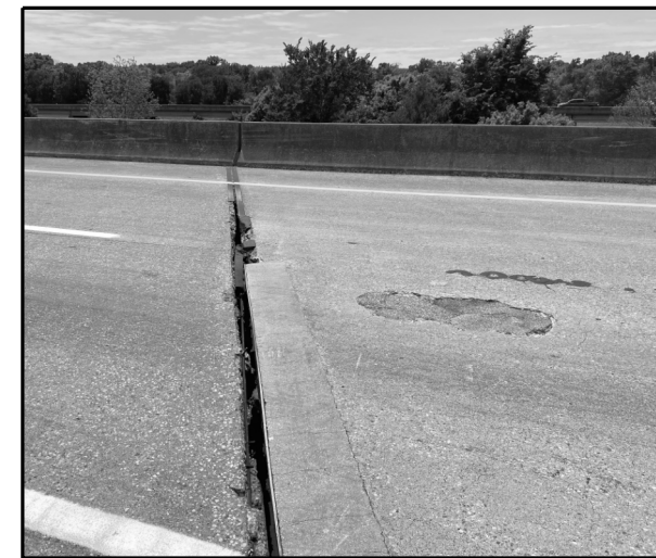
(Approx. 10 SF near Bent 5)
