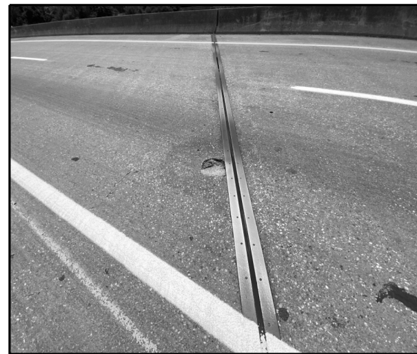
(Approx. 2 SF near Bent 4)
