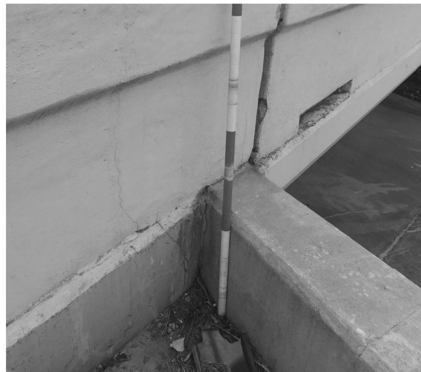
SB3 - Cracking on abutment 4 wingwall and rail at North end of abutment
