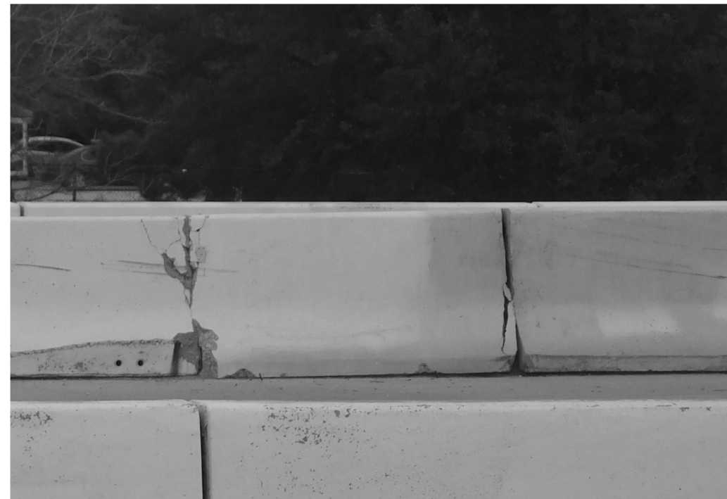
R1a/R1b - Impact damage on south face of portable CTB sitting on approach slab at abutment 1
