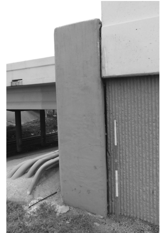
M2 - Joint seal failure on retaining wall at North end of abutment 1
