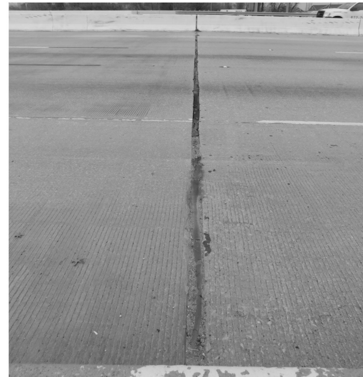
D4 - Relief joint seal failure at abutment 4 approach slab
