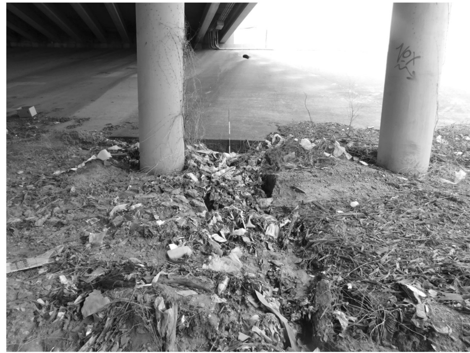
M3 - Erosion caused by drainage outlet on riprap at North end of abutment 1
