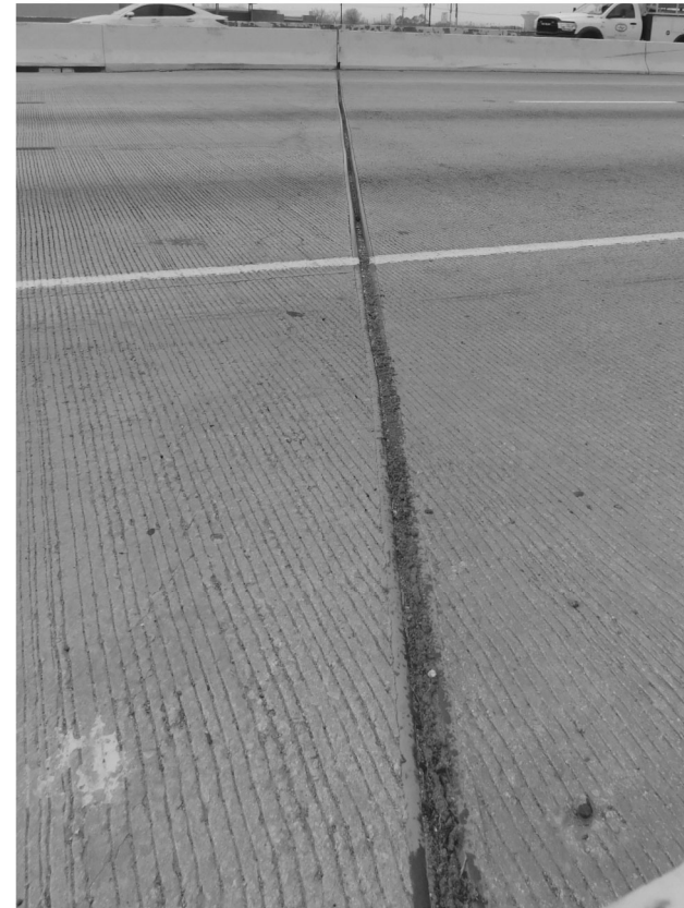
D3 - Expansion joint seal failure at abutment 4
