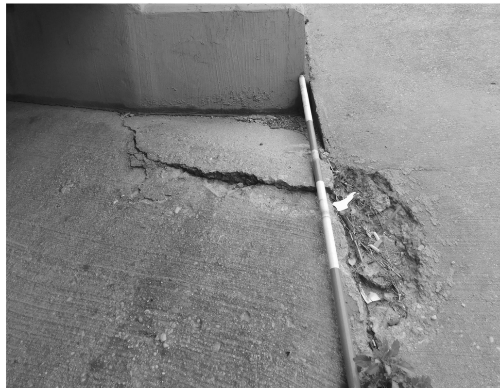
M1/M2/M3 - Riprap spalling at Southern corner of abutment 4, likely caused by seal failure between abutment cap and riprap
