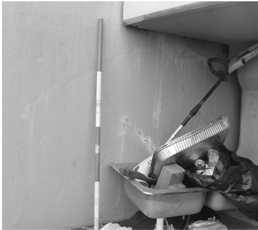
SB1/SB2 - Cracking and delamination on the face of abutment 4 backwall at the North end of the abutment
