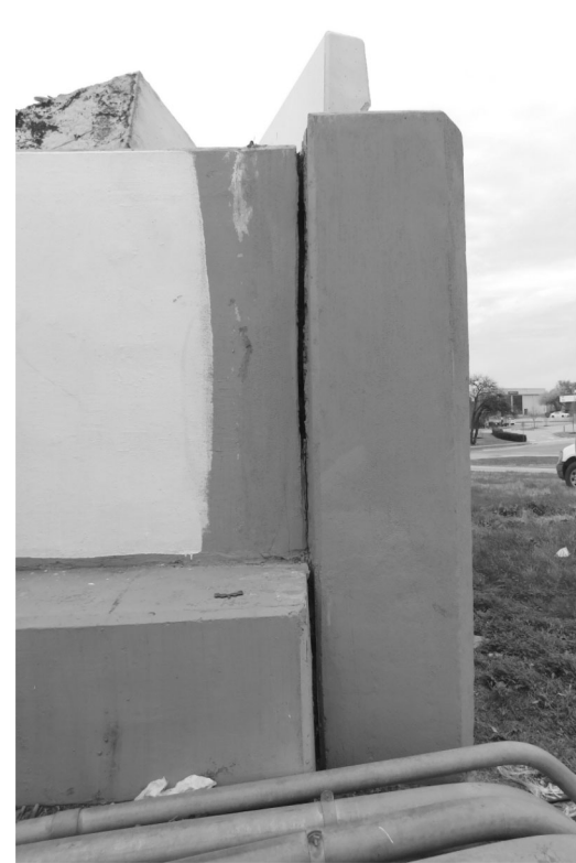
M1 - Joint seal failure between abutment 1 and retaining wall at North end of abutment
