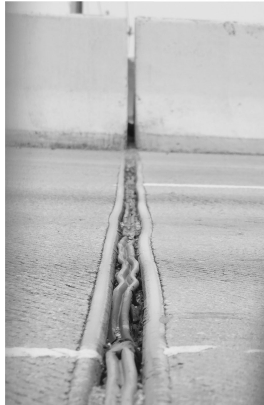
D2 - Expansion joint seal failure at abutment 1
