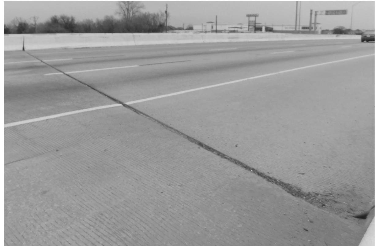
D2 - Expansion joint seal failure at abutment 1
