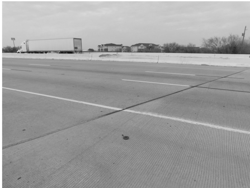
D3 - Expansion joint seal failure at abutment 4
