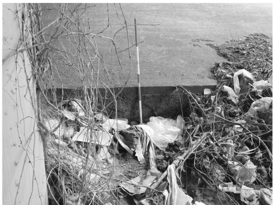
M3 - Erosion caused by drainage outlet at the riprap toewall on riprap at North end of abutment 1
