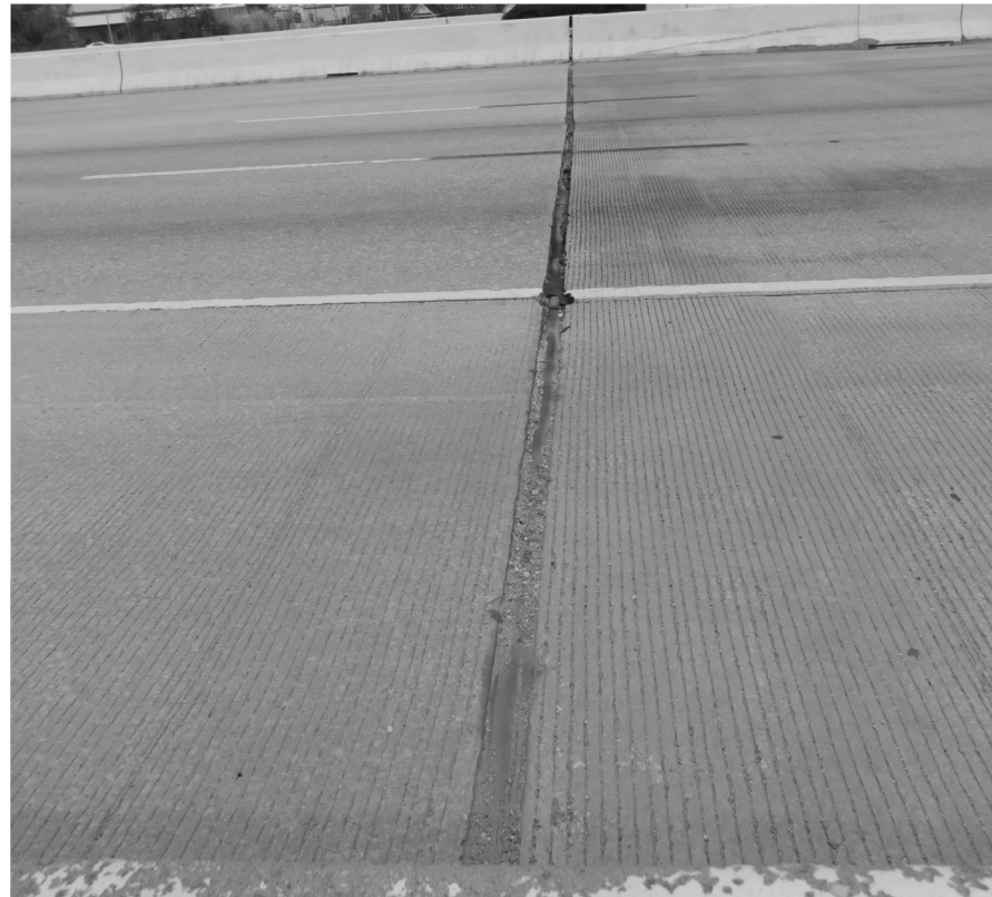
D1 - Relief joint seal failure at abutment 1 approach slab
