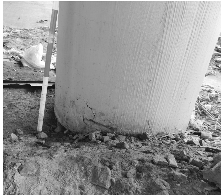
SB3 - Spall on the bottom of the second column for the South on bent 3
