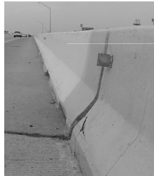
R2 - Spalling on South face of North rail at the joint on abutment 4
