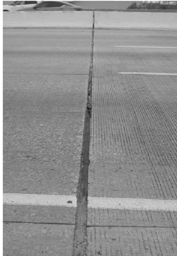
D1 - Relief joint seal failure at abutment 1 approach slab
