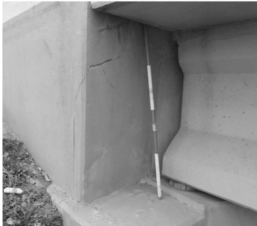
SB1/SB2 - Spall and cracking on the face of abutment 1 backwall at the south end of abutment
