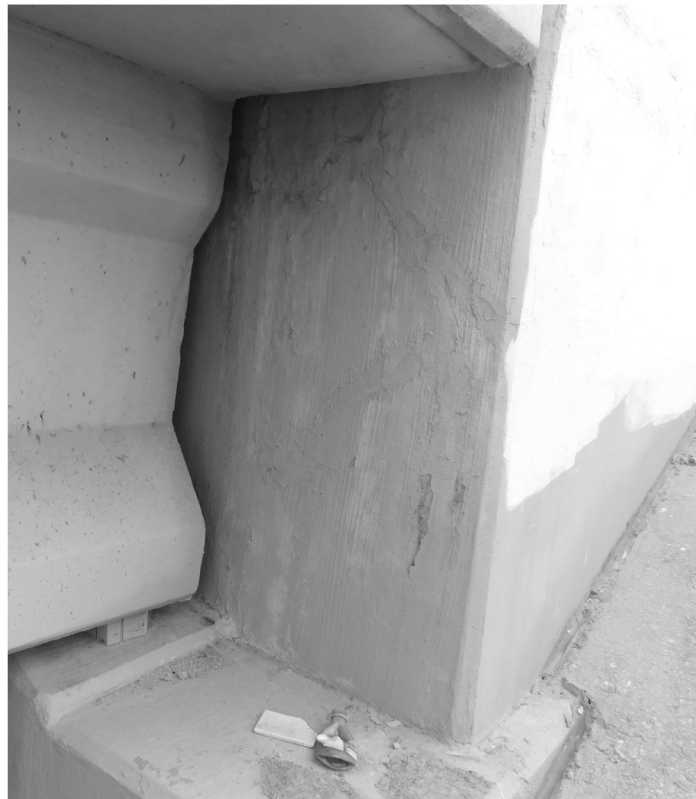
SB4 - Previous crack repair failing on the southern face of abutment 4
