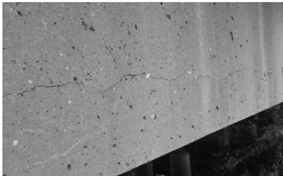
SW exterior girder stem has a horizontal crack over span 1.
