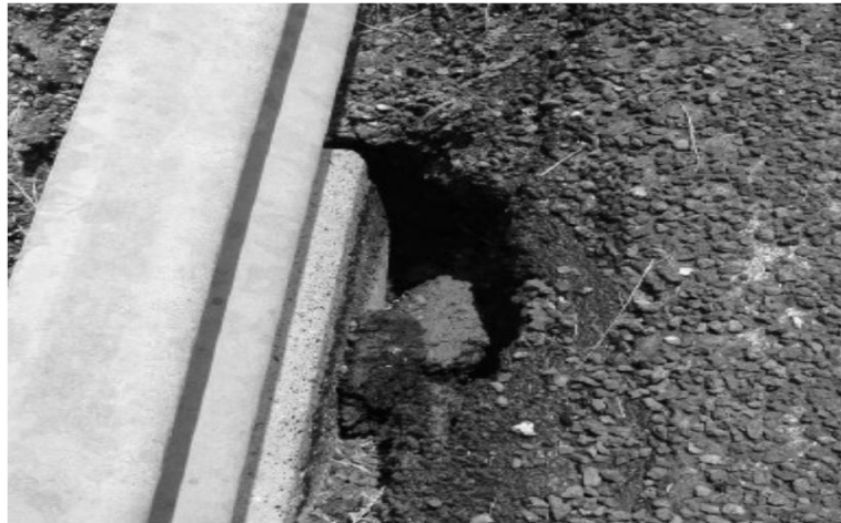
Void at southeast approach roadway encroaching onto roadway. Fill with flowable backfill.
