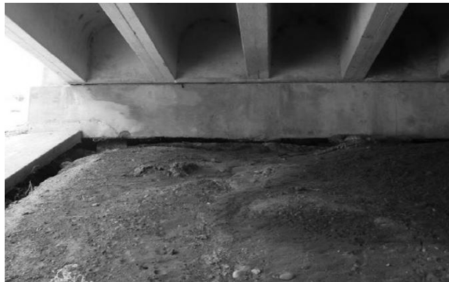
Erosion has scoured west riprap exposing and undermining west corner abutment cap.
