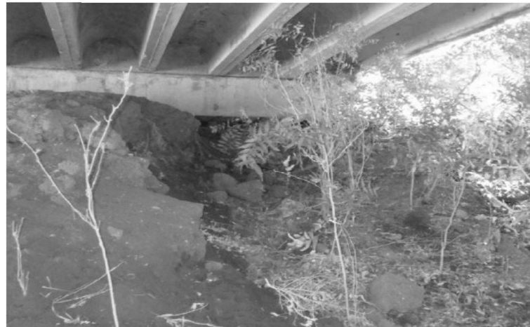
Erosion gully at south corner has undermined south corner cap and pile.
