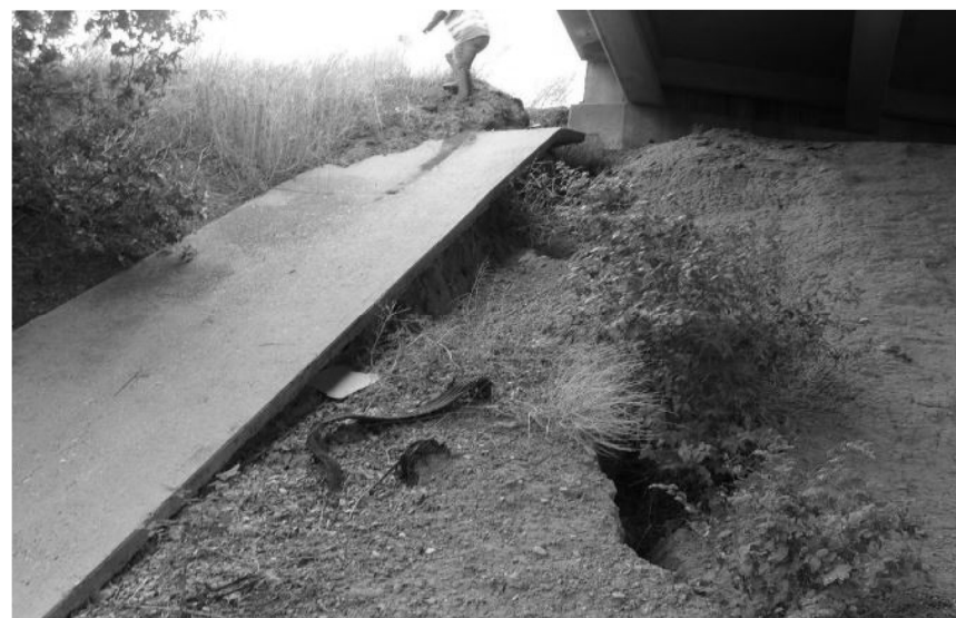
East abutment (bent #4), erosion and undermining of drain flume at northeast corner (~30 yards of erosion).
