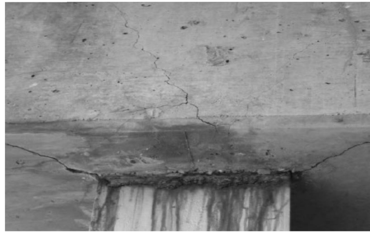
Bottom of cap have stress cracks at piles 1 at bent 3 and exists at pile 7 bent 3, piles 1,5 and 7 at bent 2. Repair with overhead patching.
