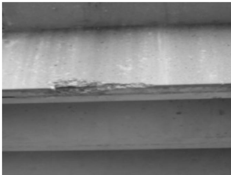
Minor spall with exposed rebar on southwest exterior beam over center span.
