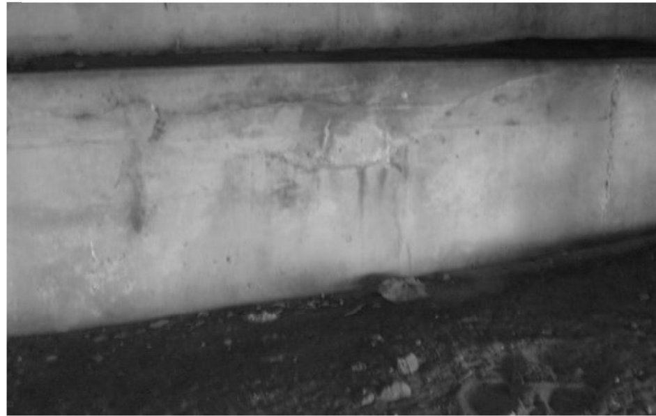
West abutment cap (bent #1), cracks and delaminations.
