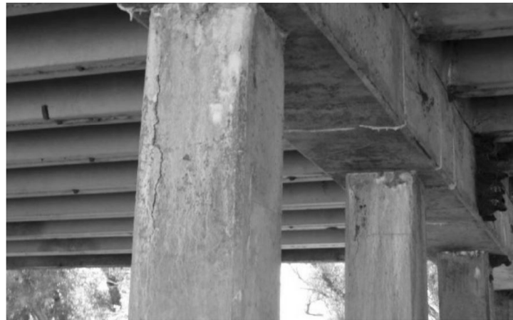
Typical cracks on columns and bent cap.
