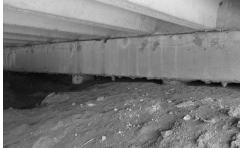
Northwest abutment cap is exposed and undermined due to run off.
