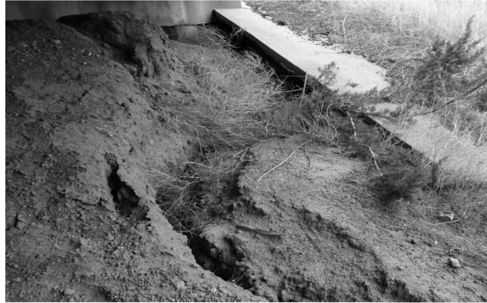
West abutment cap (bent #1), erosion and undermining of cap and drain flume at northwest corner (~30 yards of erosion). 3' of exposed drilledshaft.
