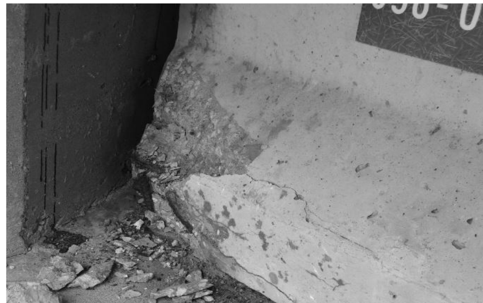
Typical spalling w/exposed reinforcing on ends of 10 girders.
