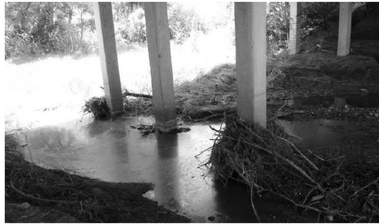
Drift accumulation caught at bent 3 piles. Remove drift (approx. 5 CY). This work is paid by item 0100-6002 Preparing ROW, 1 STA.
