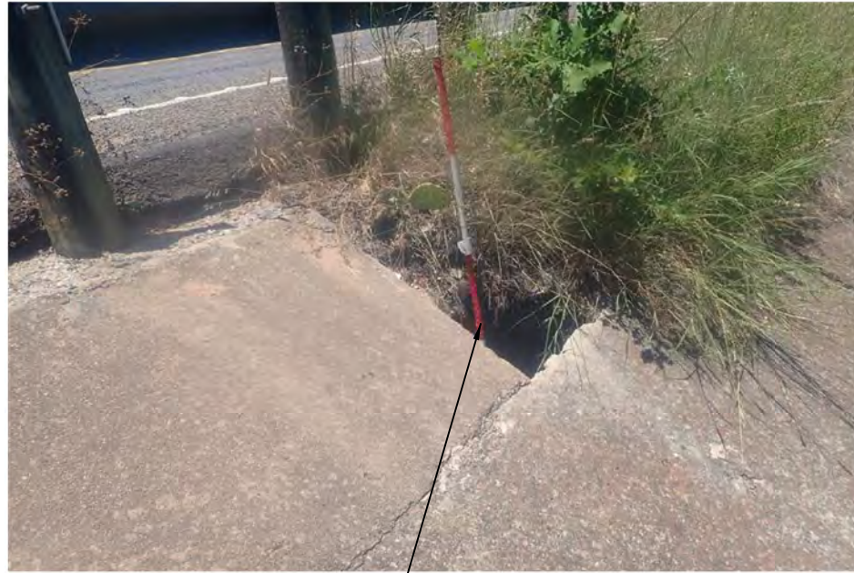
Embankment erosion at the NW corner
