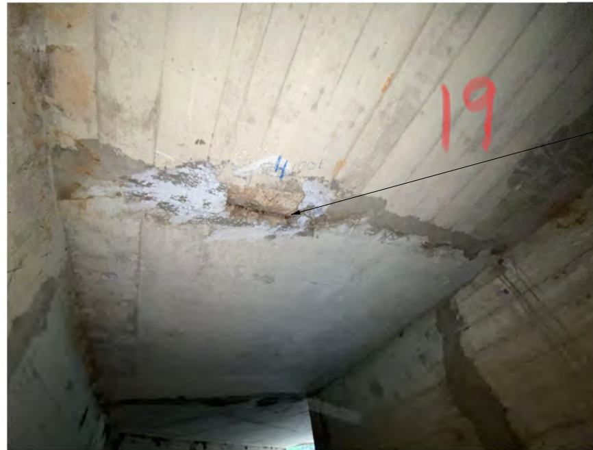
CRACKS AND MINOR SPALLS AT WIDENING JOINTS
