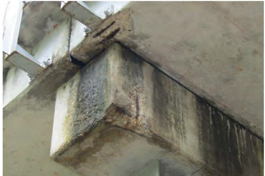
PHOTO 1 Description West end of Bent cap 3 has up to 1.5 SF by 2" deep spall with exposed rebar.
