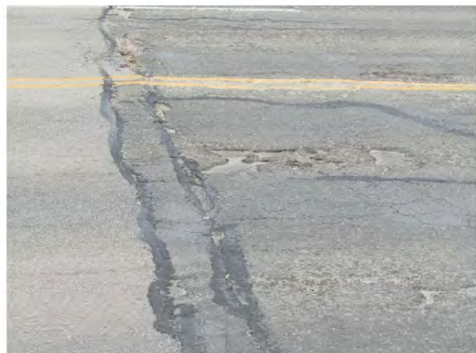
PHOTO 1 Description Span 1 wearing surface at Abutment 1 showing moderate wear, moderate cracks and potholes
