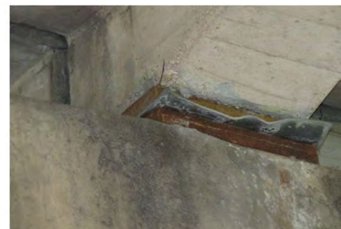
PHOTO 1 Description Beam 6 bearing in Span 4 at Bent 5 showing moderate corrosion on the bearing plates and the displaced bearing material
