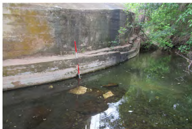
PHOTO 1 Description Southwest riprap toe wall exposed 3.5' due to scour (looking southwest).
