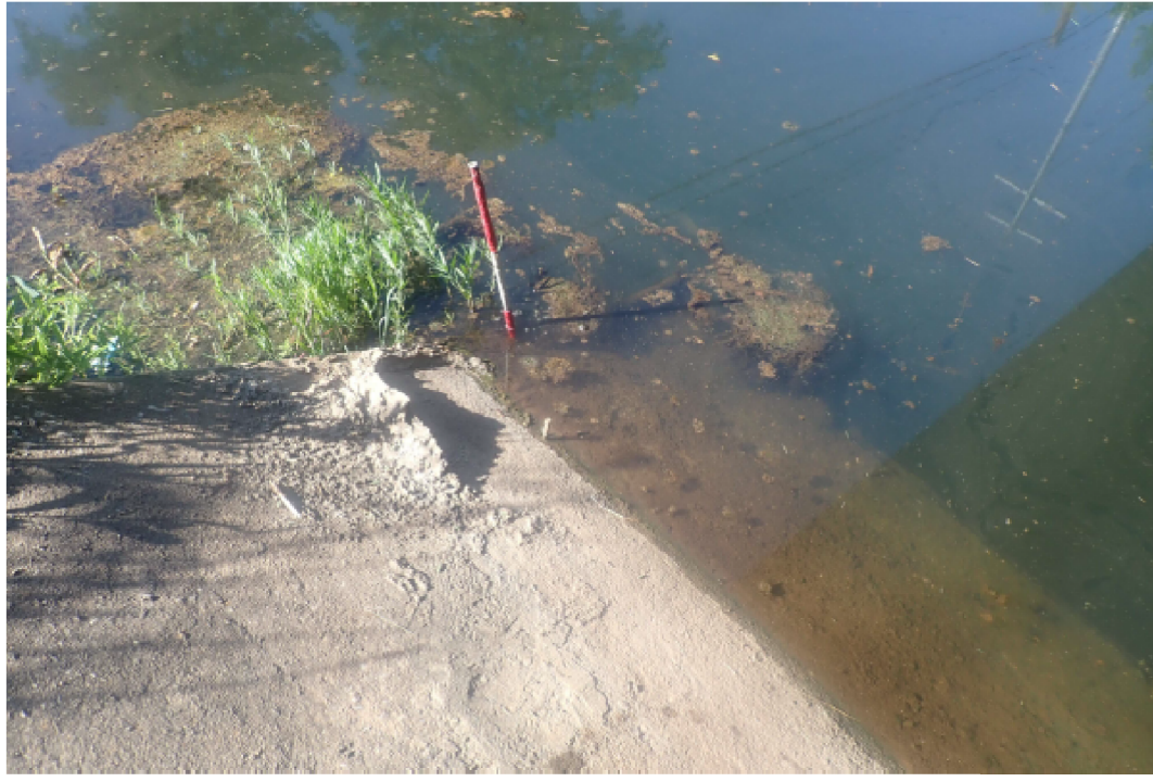
PHOTO 1 Description Moderate scour has exposed 7' of northeast riprap toewall.
