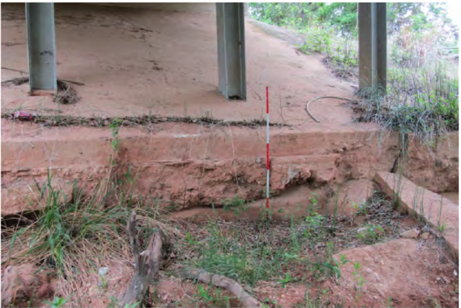
PHOTO 1 Description Channel scour exposes Abutment 1 rip rap toe wall up to 42" deep.
