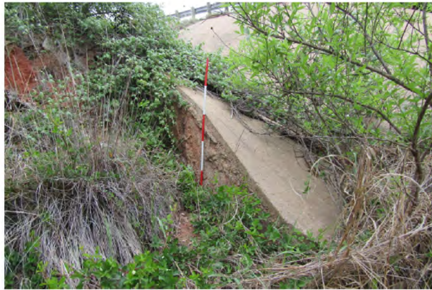
PHOTO 3 Description Erosion exposes the northwest riprap edge
