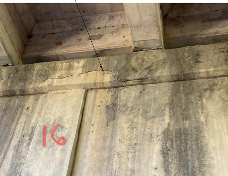
BENT CAP 4 CRACK/ DELAMINATION,
