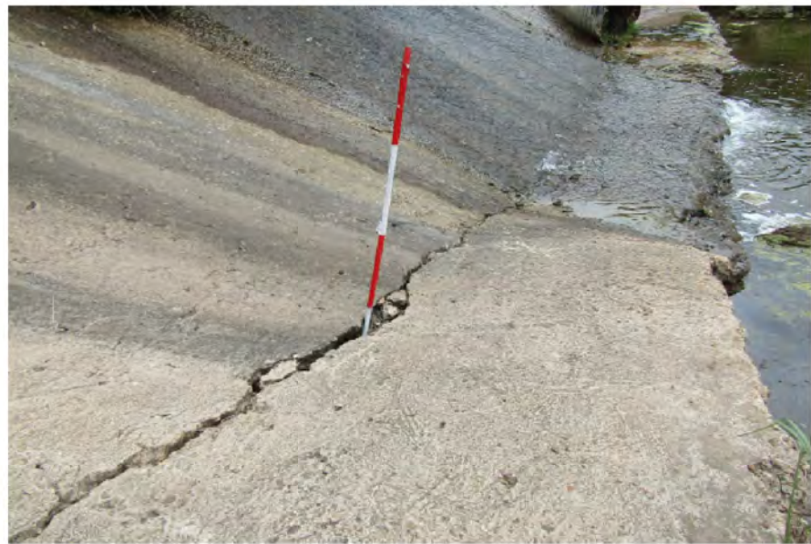
PHOTO 1 Description 2" wide crack in the downstream channel liner
