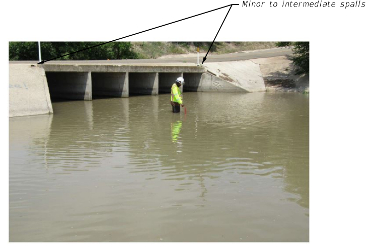
PHOTO 1 Description: Channel scour exposes the downstream culvert apron slab toe wall up to 36" deep.
