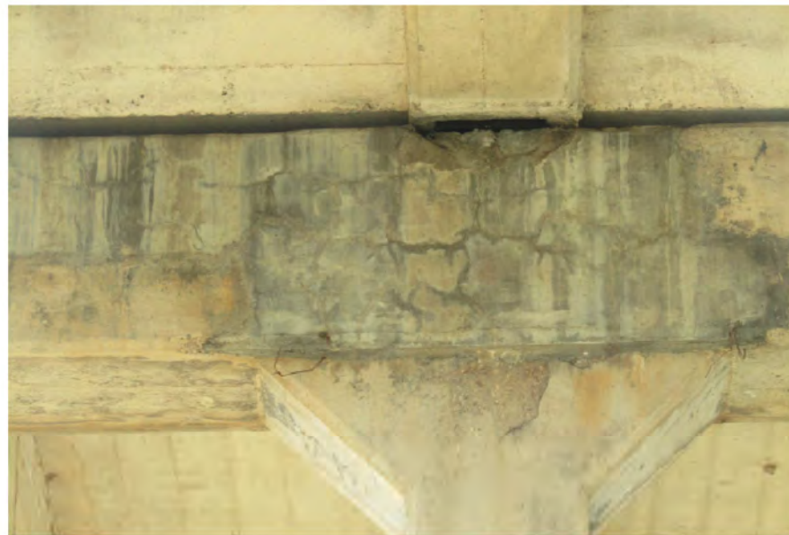
PHOTO 2 Description South face of upper cap 13 with previous repair now spalled below Beam 3 up to 2 SF by 3" deep spall with exposed rebar (looking north). Note delamination spall at top of column.
