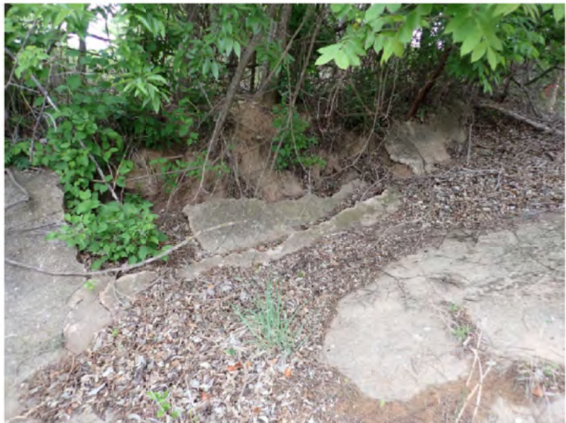
PHOTO 1 Description The southeast drain flume is fractured due to settlement.
