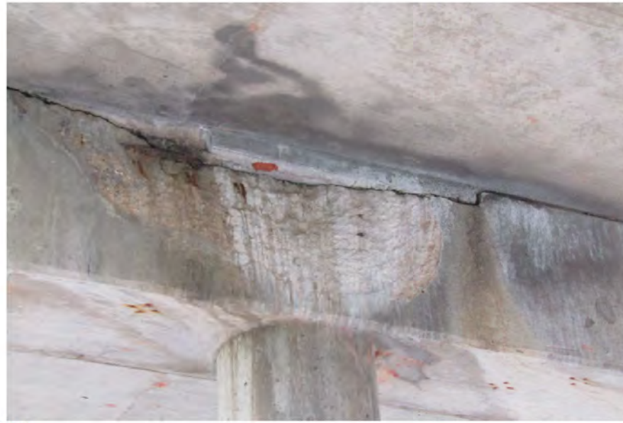
PHOTO 1 Description 12 SF by 5" deep spall with exposed rebar in the Bent 8 cap
