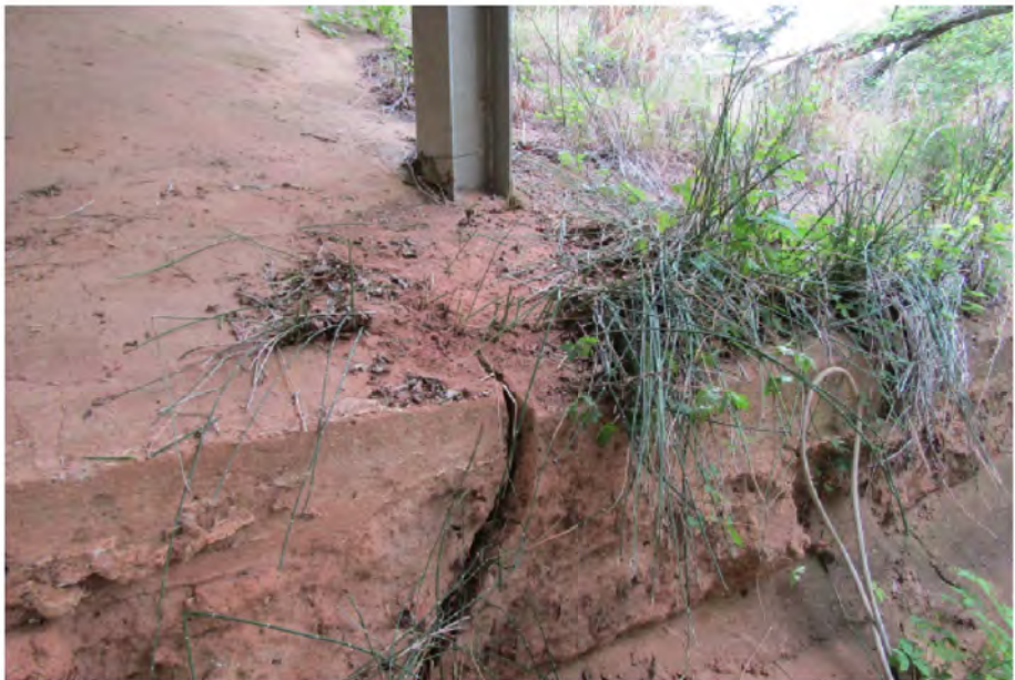
PHOTO 1 Description The west concrete rip rap has up to 2" wide cracks extending from Pile 1 at Bent 2.
