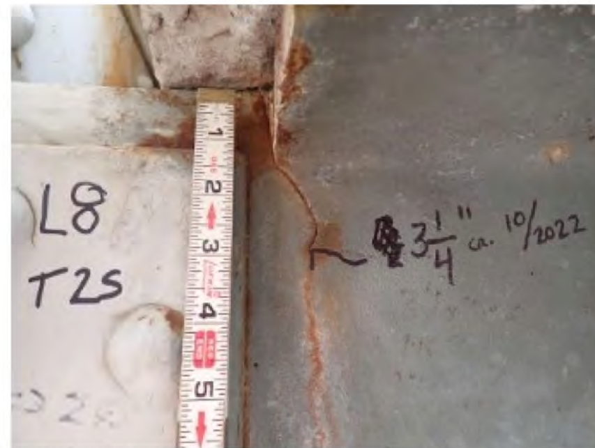
PHOTO 2 Recommended Maintenance Needs Description Span 10, Floorbeam 8, West Truss 3-1/4" long crack in floorbeam web at cope
