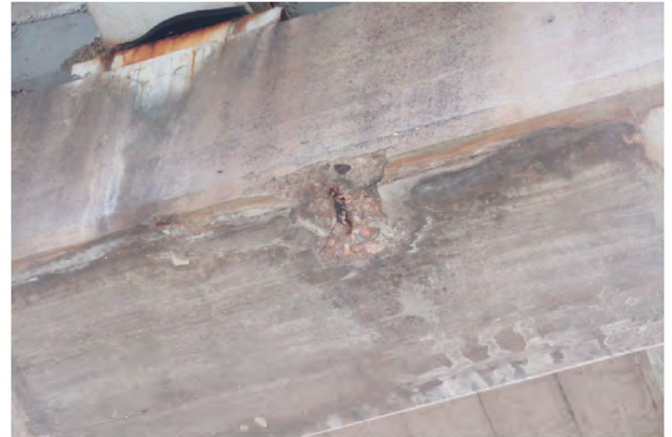
PHOTO 3 Description Bent 8 upper cap soffit spall 1 SF by 2" deep with exposed rebar (looking north).
