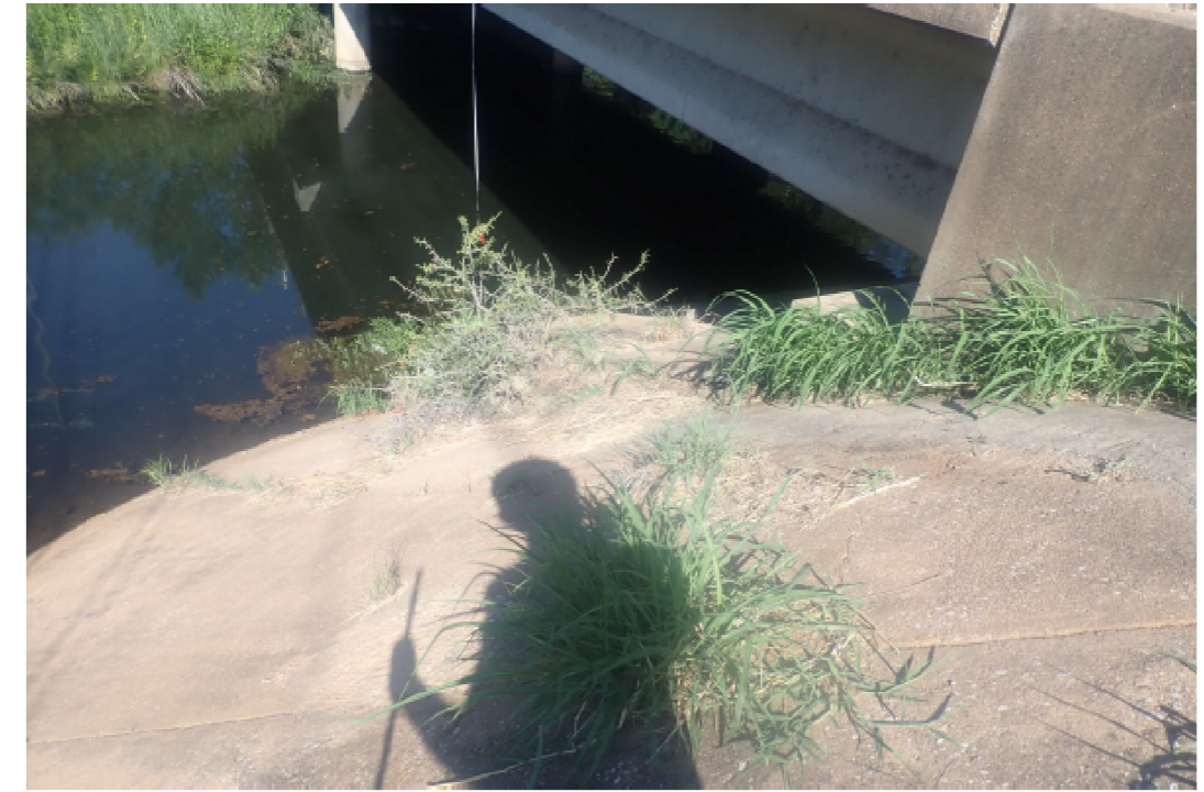
PHOTO 1 Description The northeast concrete riprap has settled up to 30" deep.
