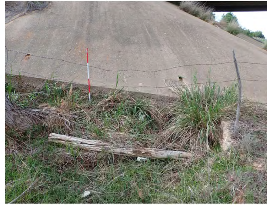
PHOTO 1 Description Southwest riprap toe wall is exposed up to 3'
