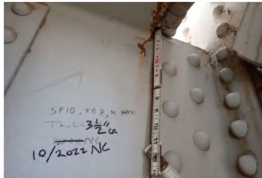
PHOTO 1 Recommended Maintenance Needs Description Span 10, Floorbeam 8, West Truss 3-1/2" long crack in floorbeam web at cope
