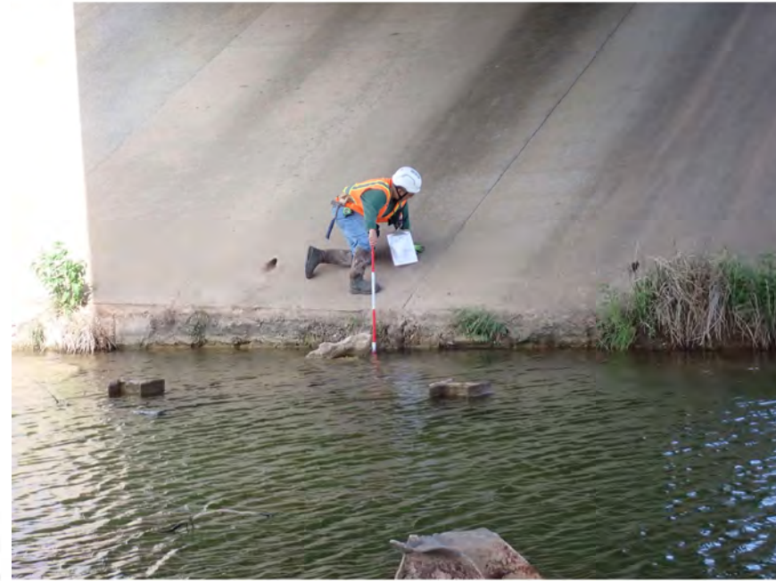
PHOTO 1 Description East riprap toe wall exposed up to 3'
