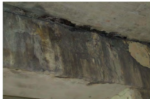
PHOTO 1 Description North face of Bent cap 3 with 48" wide by 24" high by 3" deep spall with exposed rebar over Column 2 (looking southwest).
