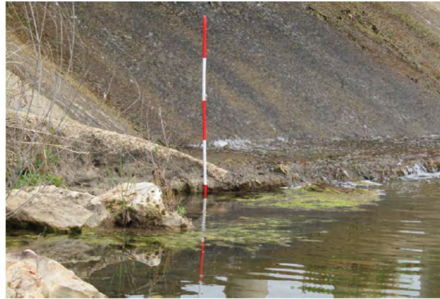
PHOTO 2 Description Scour at the downstream channel liner toe wall
