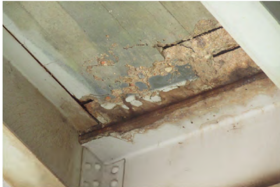
PHOTO 1 Description Span 10 deck soffit spall 3 SF by 2" deep with exposed rebar above Floorbeam 7 (looking northwest).
