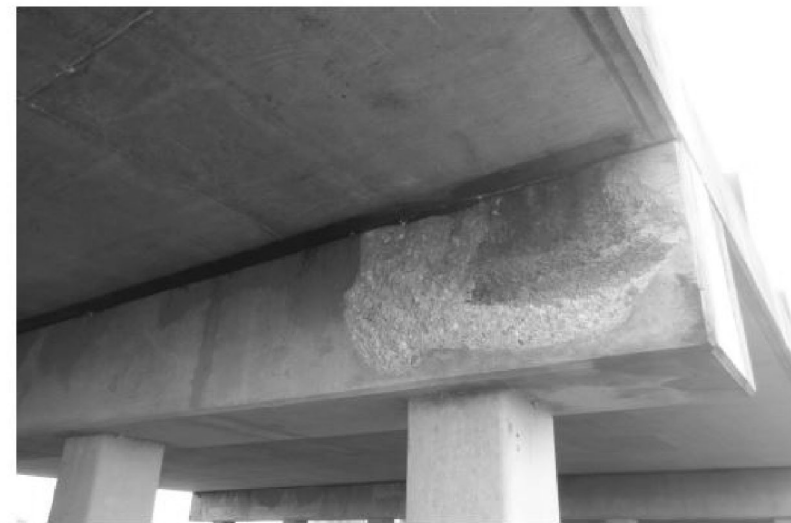
PHOTO 1 Description FAILED PATCH (SPALL) ON BENT CAP 21 AT WEST END LOOKING SOUTH
