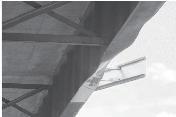
IMPACT DAMAGE SPAN 3 GIRDER 5
