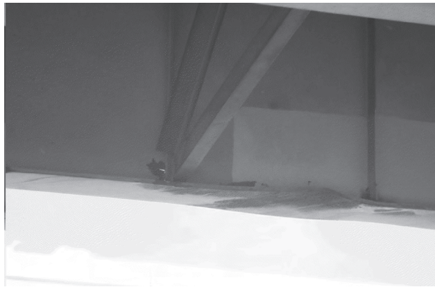
IMPACT DAMAGE SPAN 3 GIRDER 1
