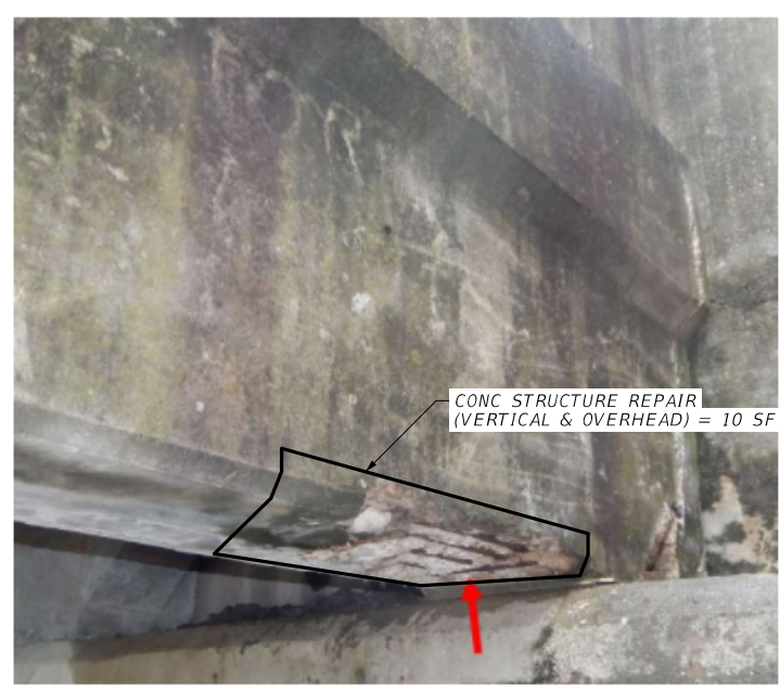
PHOTO 7 INTERMEDIATE SPALL WITH EXPOSED REINFORCEMENT ON BOTTOM SURFACE ON BEAM 7 OF SPAN 5
