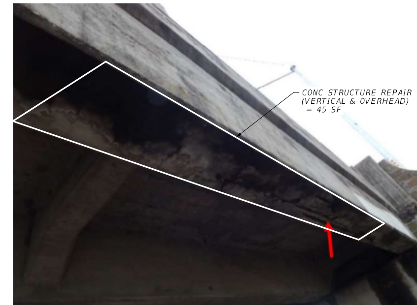
PHOTO 2 MINOR SPALL WITH EXPOSED STEEL REINFORCEMENT ON BOTTOM SURFACE OF BEAM 1 OF SPAN 1
