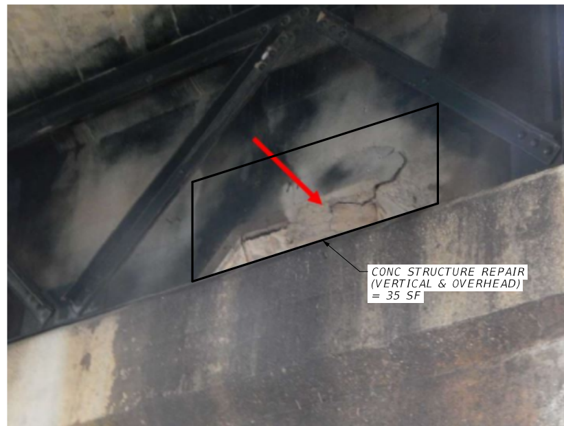
PHOTO 1 INTERMEDIATE SPALL ON CONCRETE DIAPHRAGM OVER BENT 2
