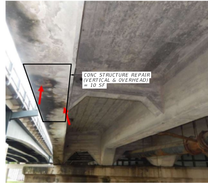
PHOTO 9 MINOR SPALLS ON BEAM 7 BOTTOM SURFACE OF SPAN 5
