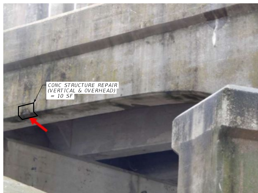
PHOTO 3 MINOR SPALL WITH EXPOSED REINFORCEMENT ON EAST SIDE ON BEAM 7 OF SPAN 1
