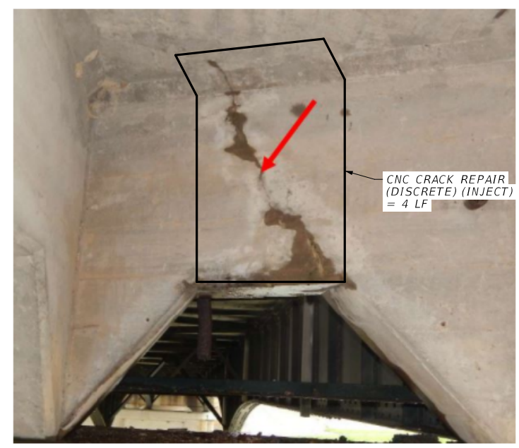
PHOTO 5 CRACK ON DIAPHRAGM BETWEEN BEAM 1 AND BEAM 2 AT BENT 5.
