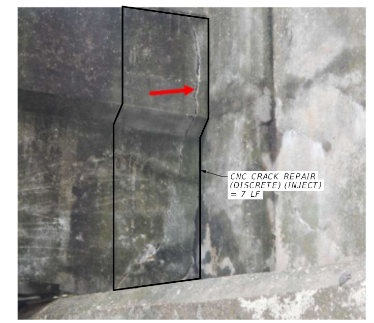
PHOTO 6 CRACK ON NORTH END ON BEAM 7 OF SPAN 5
