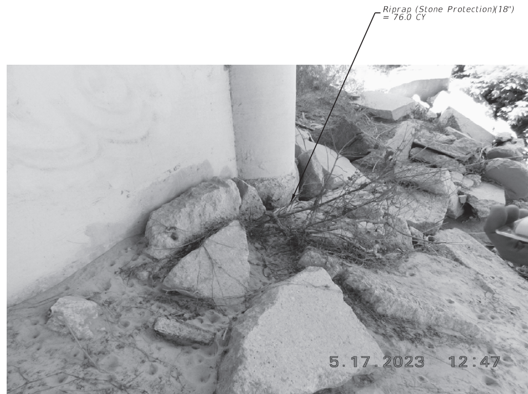
M-2 (Photo-7): Scour at Bent-17 for all 3-DS (scour depth 2.5')
