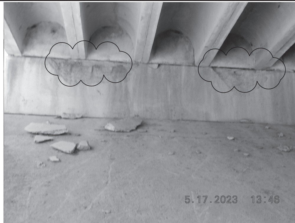
SB-5,6_PIC-1 @ ABUT30 8'x3' & 4'x3' CONCRETE SPALL BETWEEN GIRDER 1-5 (VERTICAL OVERHEAD)
