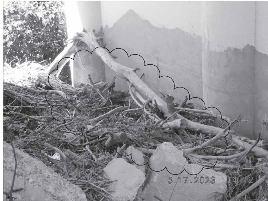
M-3,_PIC-9 @ BENT17 & DEBRIS PILE 3x5x40 TO BE REMOVED THRU OUT THE PART OF COLUMN & DRILL SHAFT
