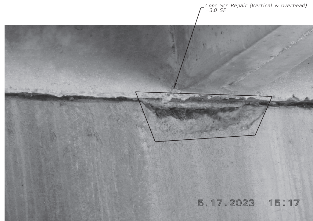
SB-2 (Photo-2): Spall & Rebar exposed at Abut-1
