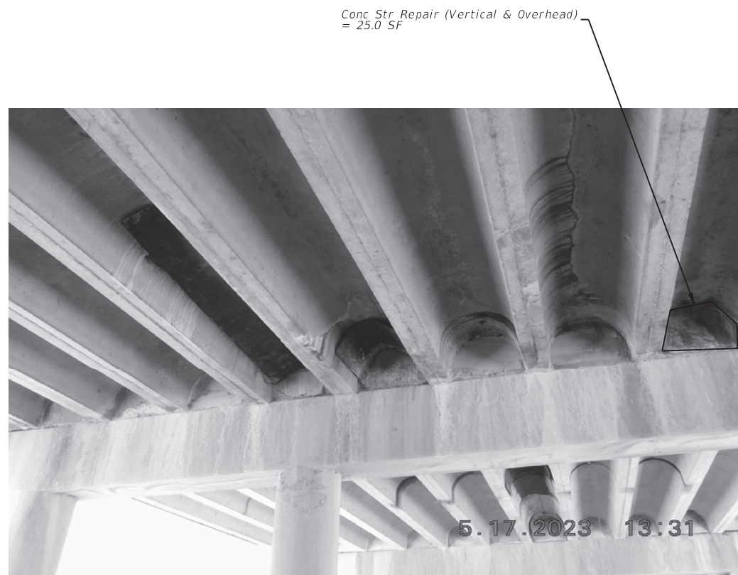
SP-10 (Photo-19): Pan girder end spall at Bent-28
