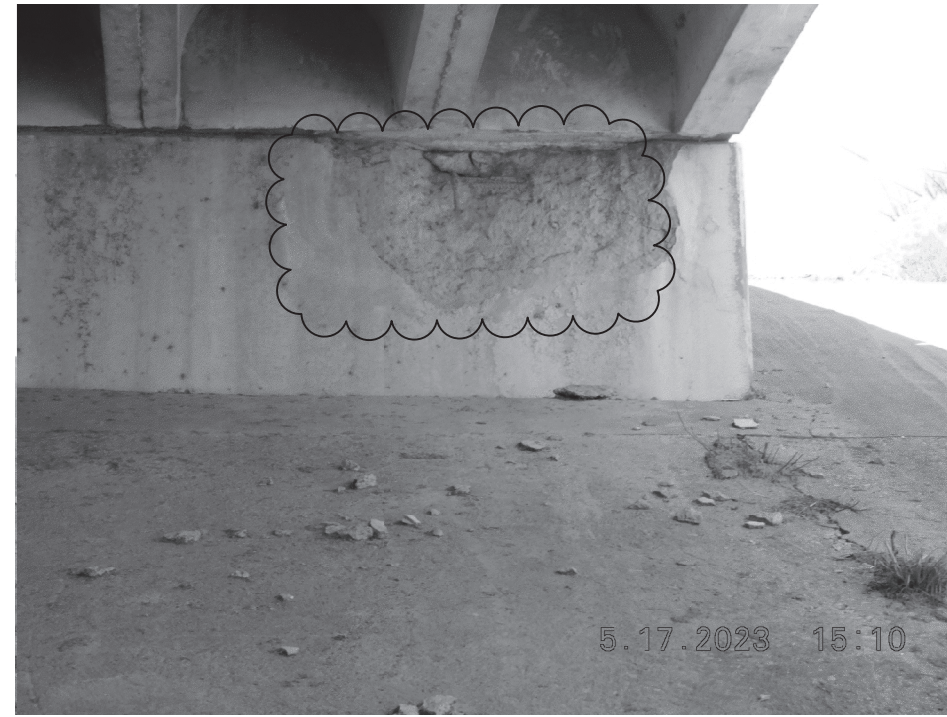
SB-1,_PIC-17 @ ABUTMENT-1 BEGIN GIRDER 7'x4'=28SF CONCRETE SPALLING, DELAMINATION & BAR EXPOSED (VERTICAL OVERHEAD)
