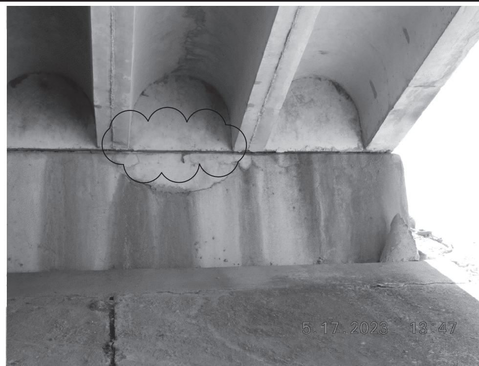
SB-7_PIC-2 @ ABUT30 5'x2' CONCRETE DELIMITATION BETWEEN GIRDER 11-12 (VERTICAL OVERHEAD)
