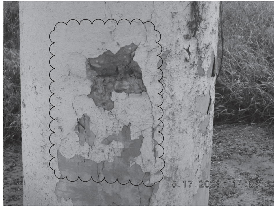
SB-4,_PIC-14 @ BENT-9 COLUMN-1 6'x2.5' CONCRETE SPALL & BAR EXPOSED (VERTICAL OVERHEAD)
