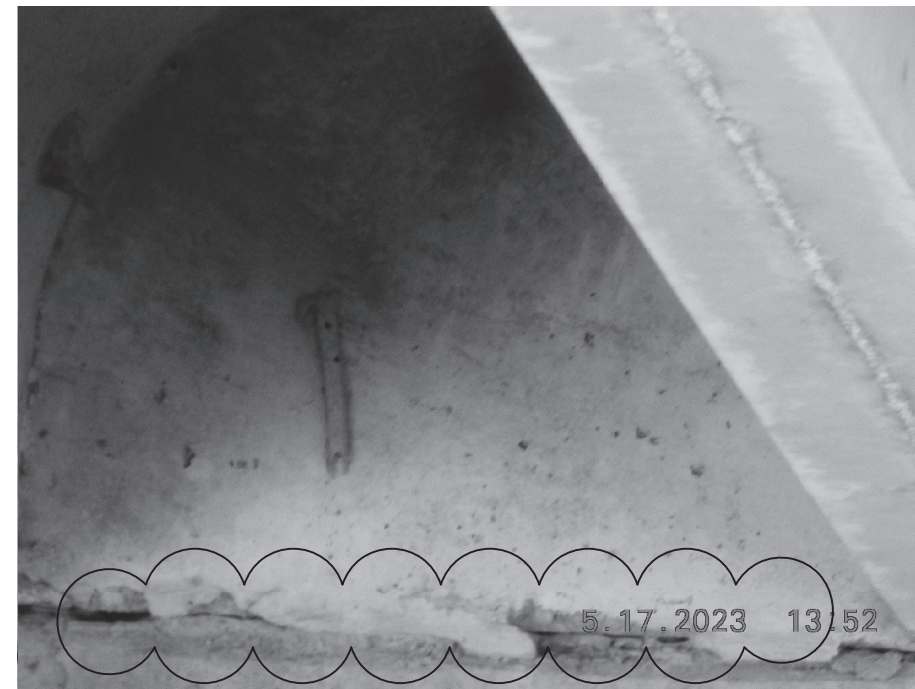
SP-6_PIC-4 @ SPAN29 5'x2' CONCRETE SPALL (VERTICAL OVERHEAD)
