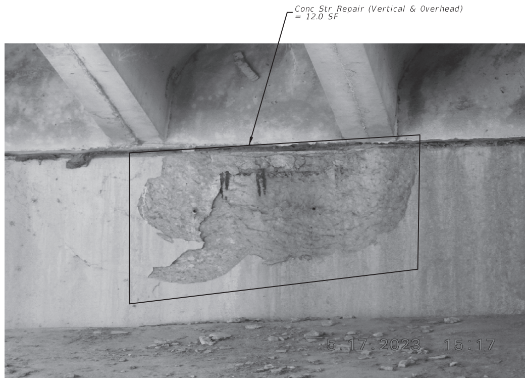
SB-1 (Photo-1): Spall & Rebar exposed at Abut-1
