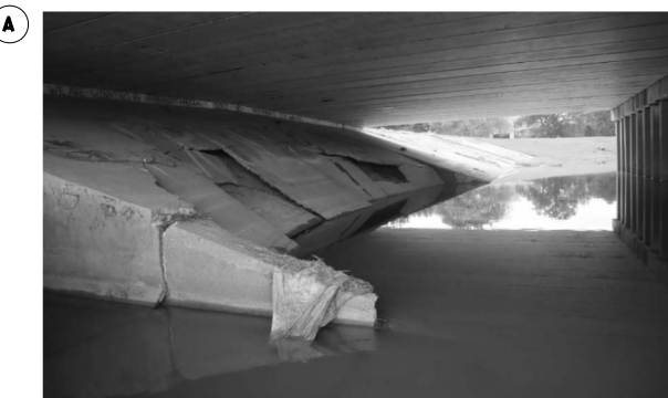
(A) REPAIR HEADWALL WORK TO BE PAID FOR UNDER ITEM: 104 6031 REMOVING CONC (HEADWALL) APPROX. 8 CY 420-6054 CONC (HEADWALL) APPROX. 8 CY
