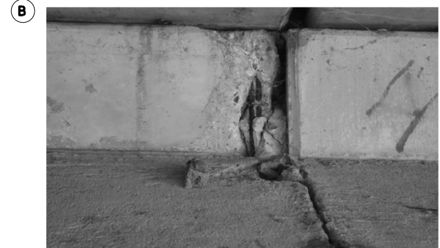
(B) SPALL WITH EXPOSED REBAR ON ABUTMENT WORK TO BE PAID FOR UNDER ITEM: 0429-6007 "CONC STR REPAIR (VERTICAL & OVERHEAD)" APPROX. 10 SF
