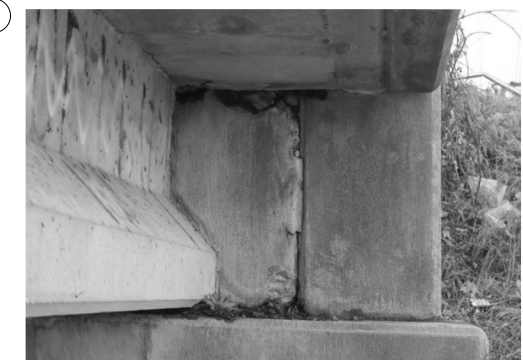
(C) REPAIR SPALL WORK TO BE PAID FOR UNDER ITEM: 0429-6007 "CONC STR REPAIR (VERTICAL & OVERHEAD)" APPROX. 10 SF
