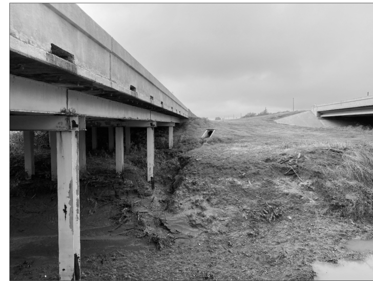
EROSION GULLY AT SW DITCH TO CHANNEL (M2)
