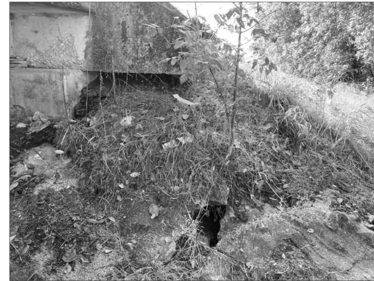
EROSION AT SW BRIDGE CORNER (M1, M2, M3)
