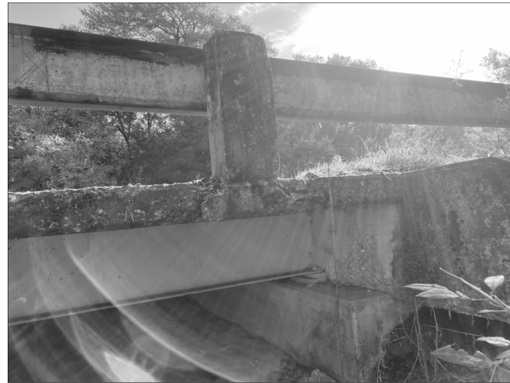
SPALL IN DECK SOFFIT AT SW CORNER (D2)
