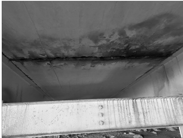
SPALL ON UNDERSIDE OF DECK SOFFIT (D2)
