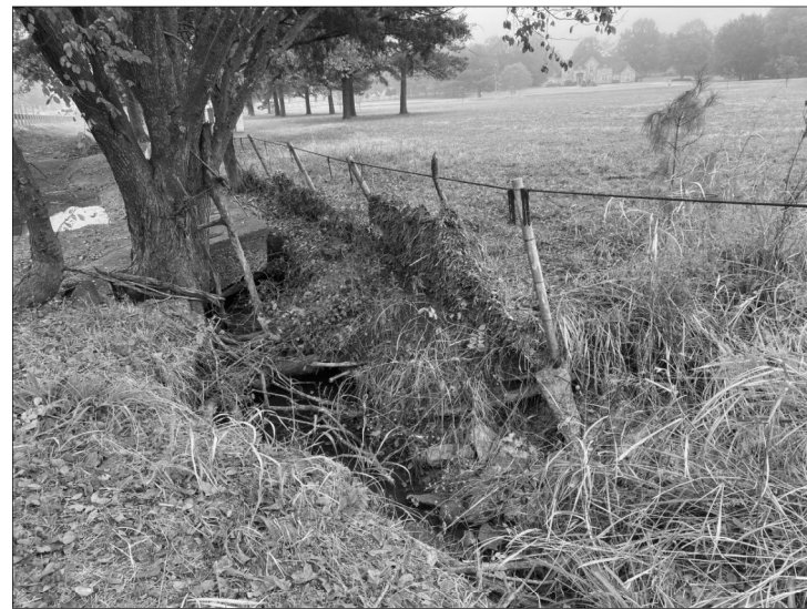
EROSION AT SE DITCH (M1 AND M2)
