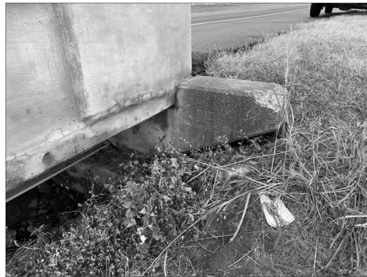
UNDERMINING AT NE WINGWALL (M1 AND SB2)
