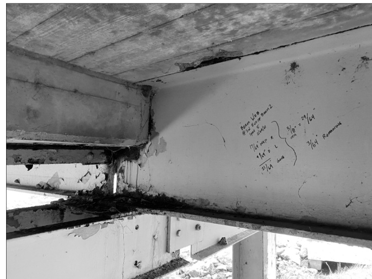
STEEL BEAM REPAIR AND TYPICAL BEAM END PAINTING LOCATIONS (SP1 AND SP2)
