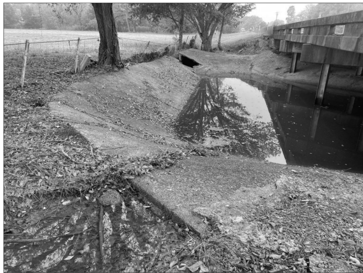
BROKEN AND SETTLED CONCRETE RIPRAP (M1 AND M2)
