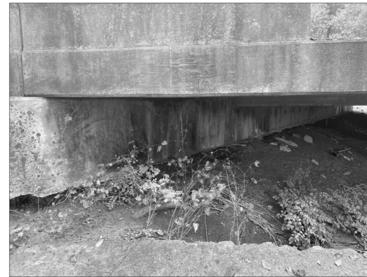
UNDERMINING AT SOUTH ABUTMENT (NORTH SIMILAR) (SB1)
