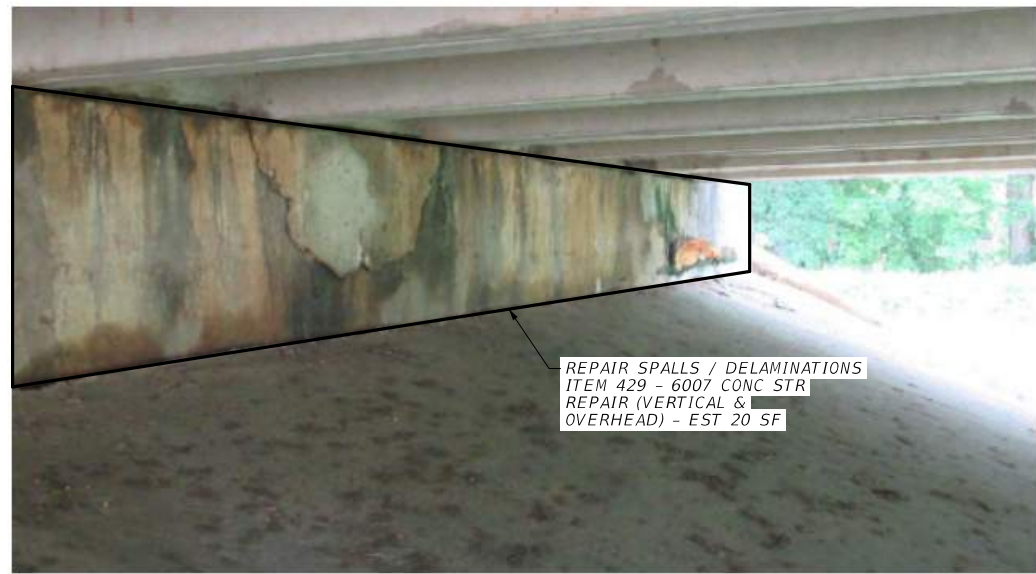
PHOTO 2 (MODERATE DELAMINATION ON NORTH ABUTMENT CAP)
