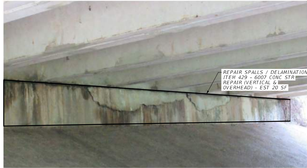
PHOTO 1 (MODERATE DELAMINATION ON SOUTH ABUTMENT CAP)
