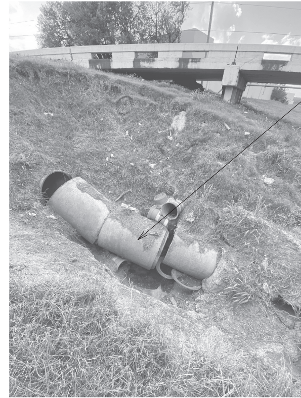
CONCRETE PIPES AND DEBRIS AT OUTFALL (Photo taken on 3-08-2023)
