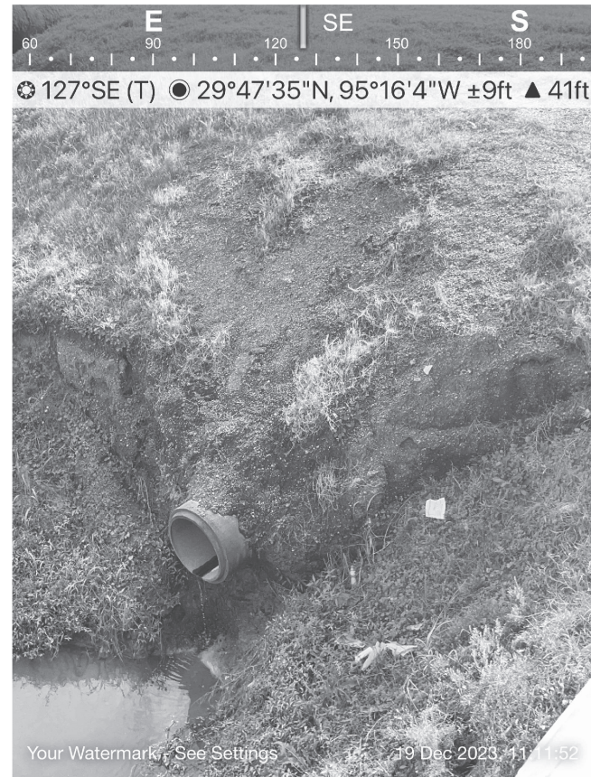
SIDE VIEW OF EROSION AT OUTFALL (Photo taken on 12-19-2023)
