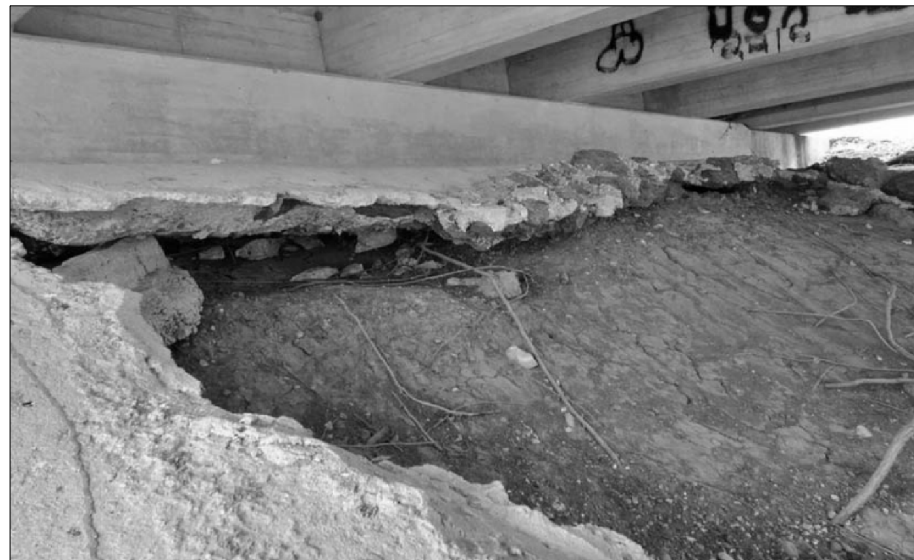
Abutments 1 and 6 - Failed concrete riprap
