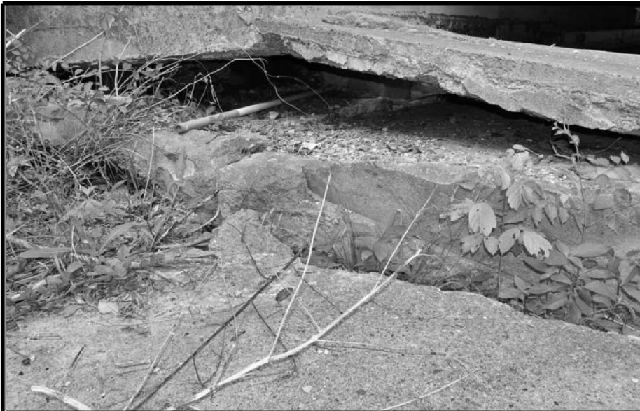
Voids under Northwest Wingwall and Abutment
