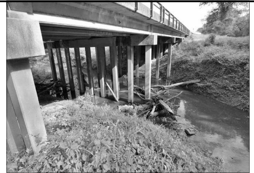
Bent 4 - Debris near bent 4
