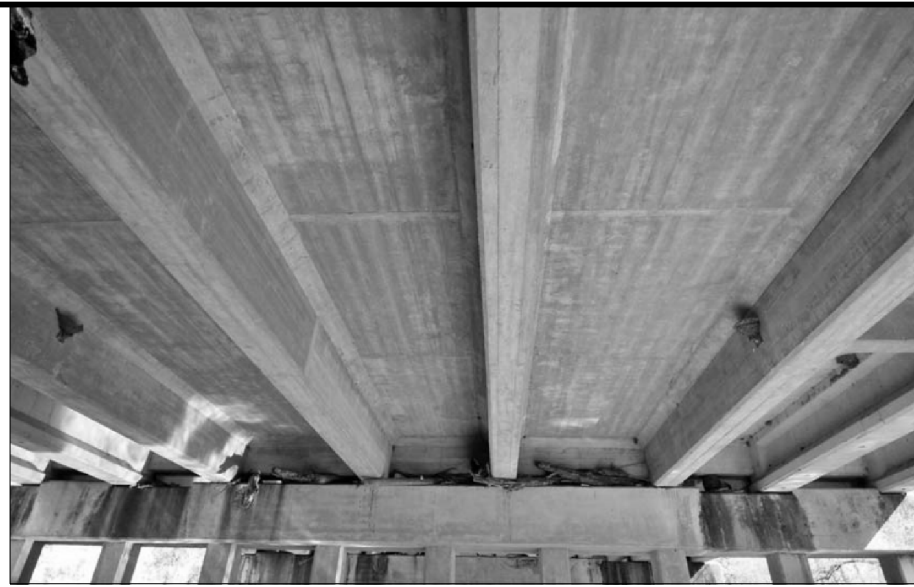
Bents 3, 4 and 5 - Debris on top of bents
