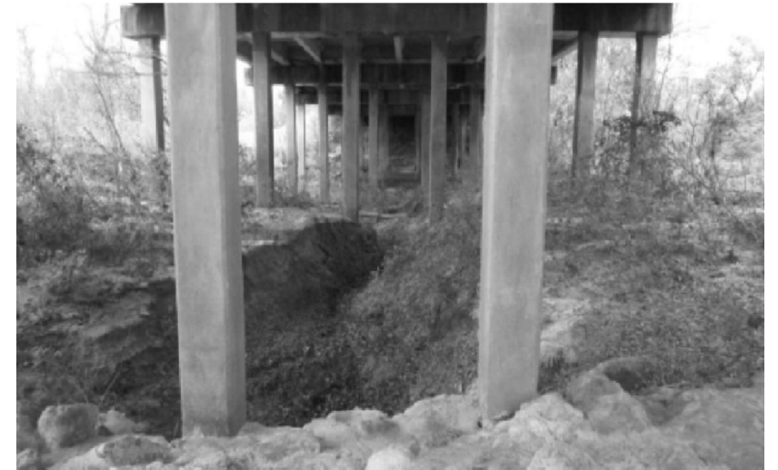
Erosion gully under bridge.
