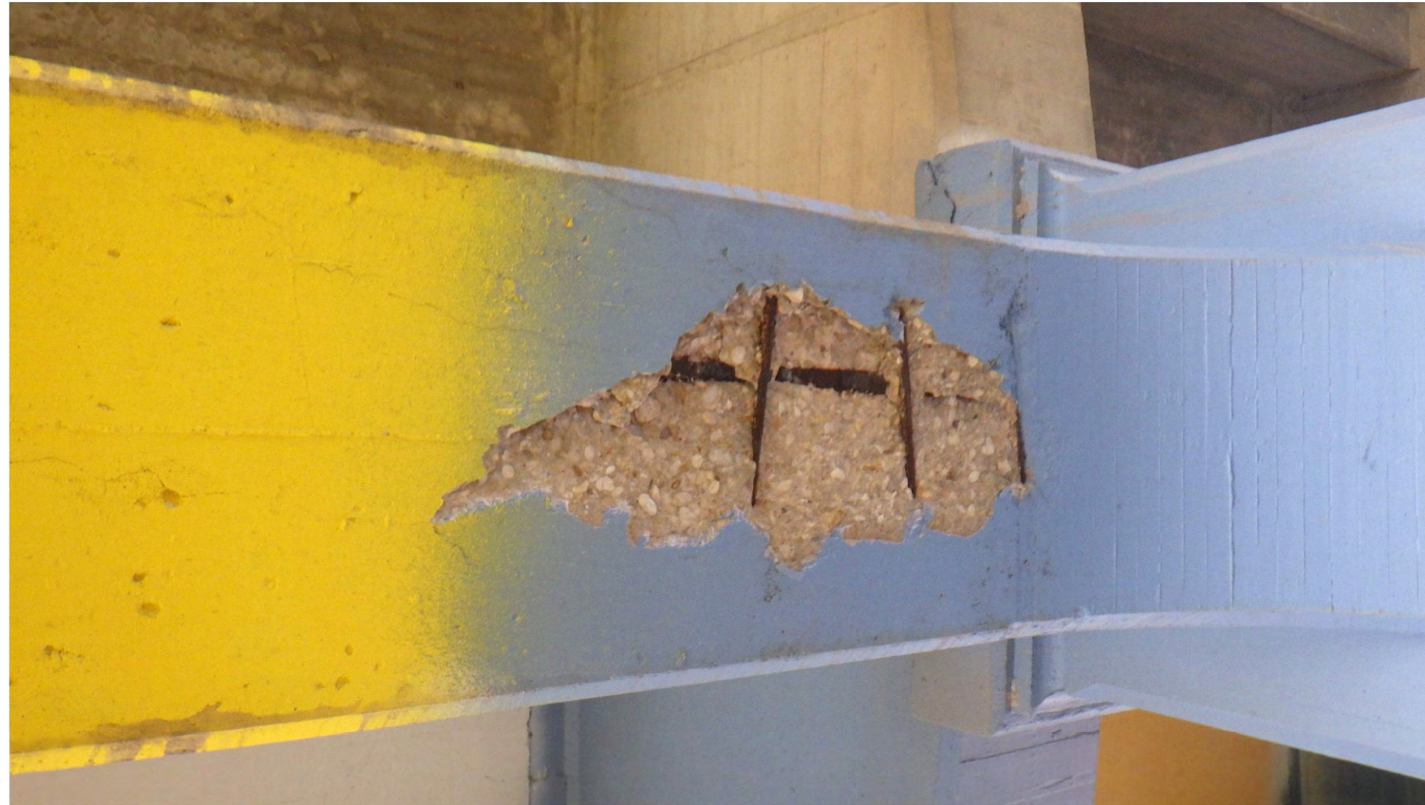
EXAMPLE OF PIER 10 SPALL DAMAGE
