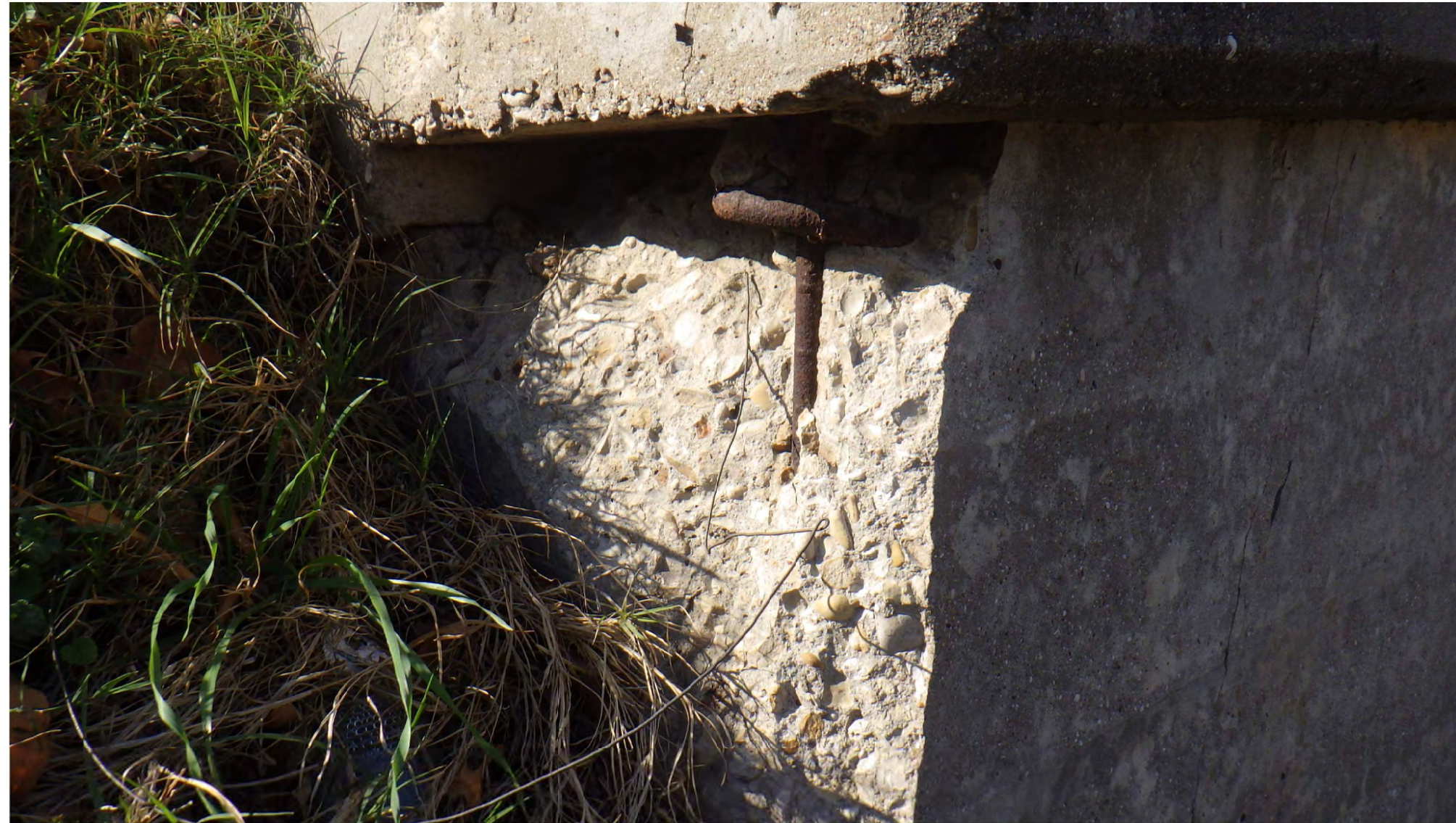
EXAMPLE OF SOUTH ABUTMENT SPALL DAMAGE
