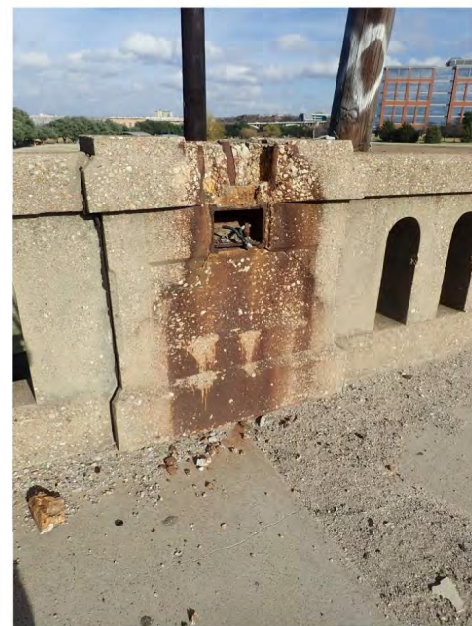
Typical pilaster spall damage
