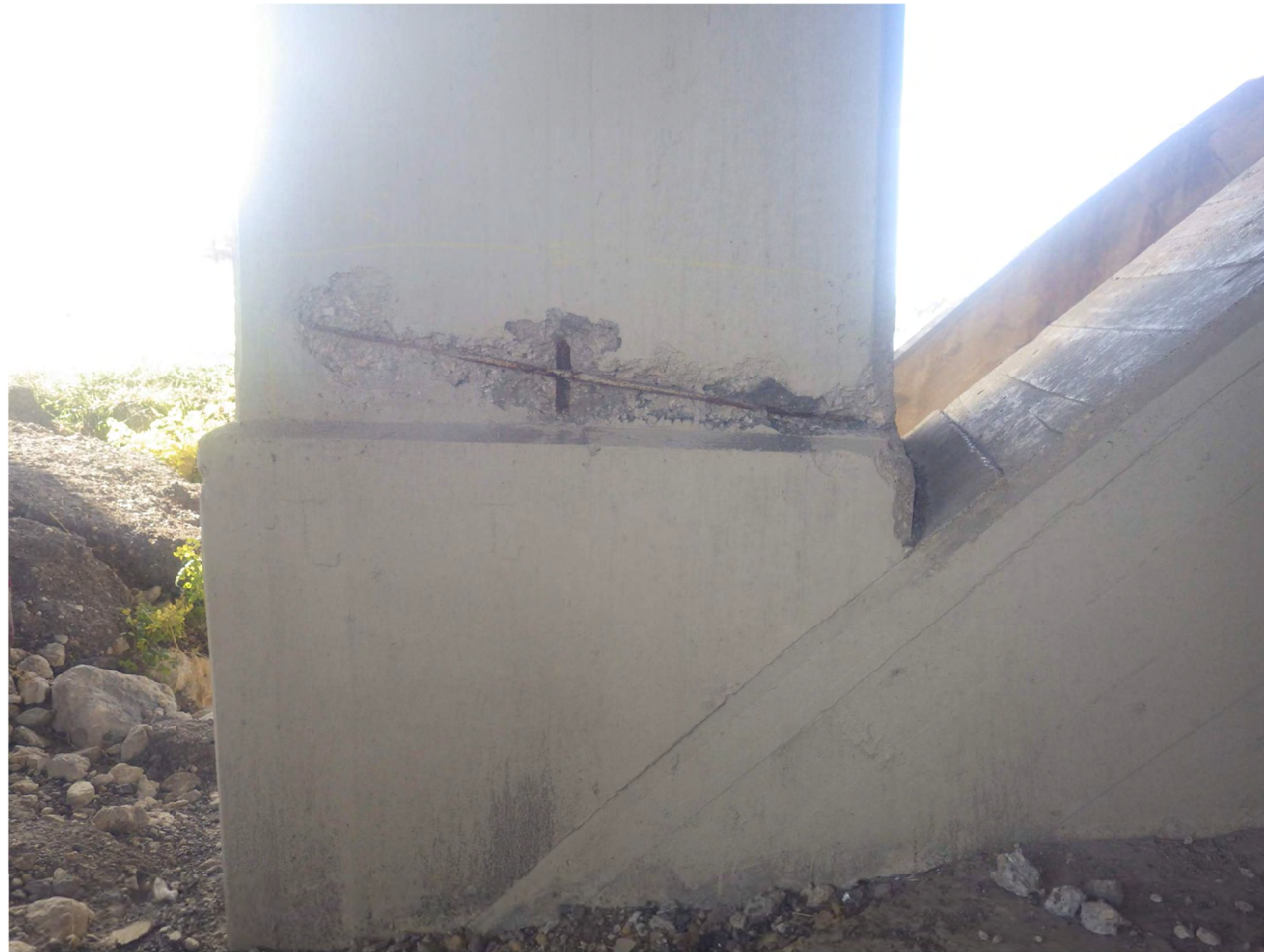
EXAMPLE OF PIER 11 SPALL DAMAGE
