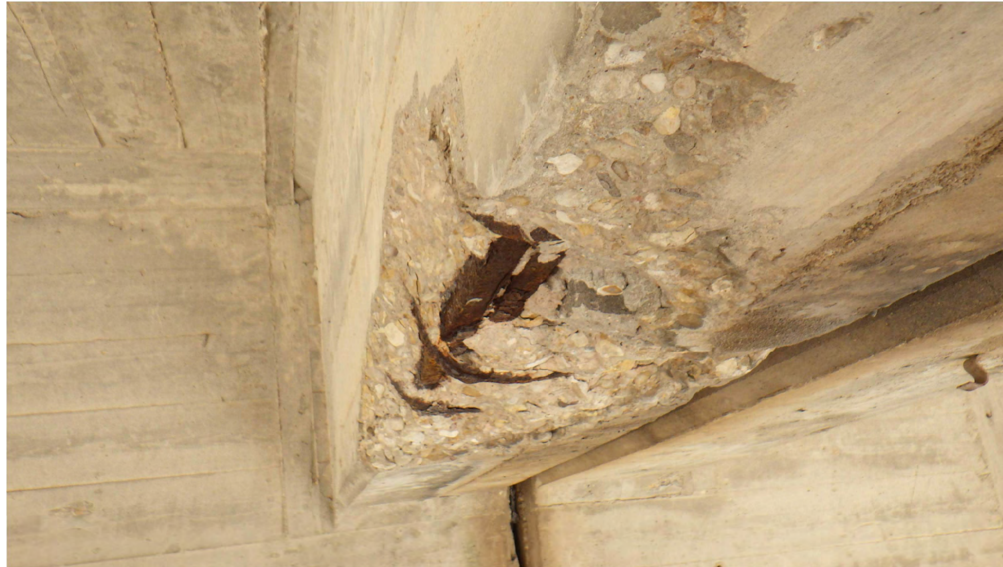
EXAMPLE OF SPAN 5 SPALL DAMAGE
