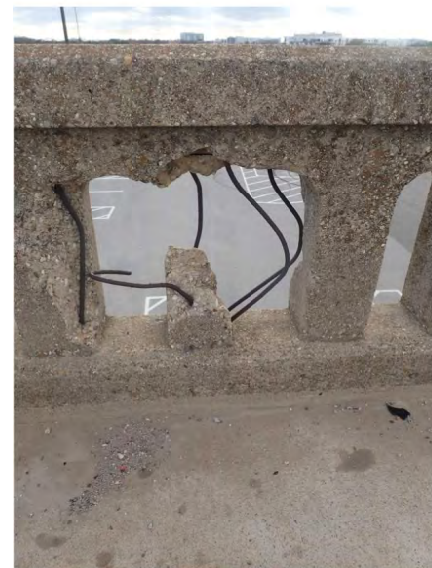
Typical impact damage at post
