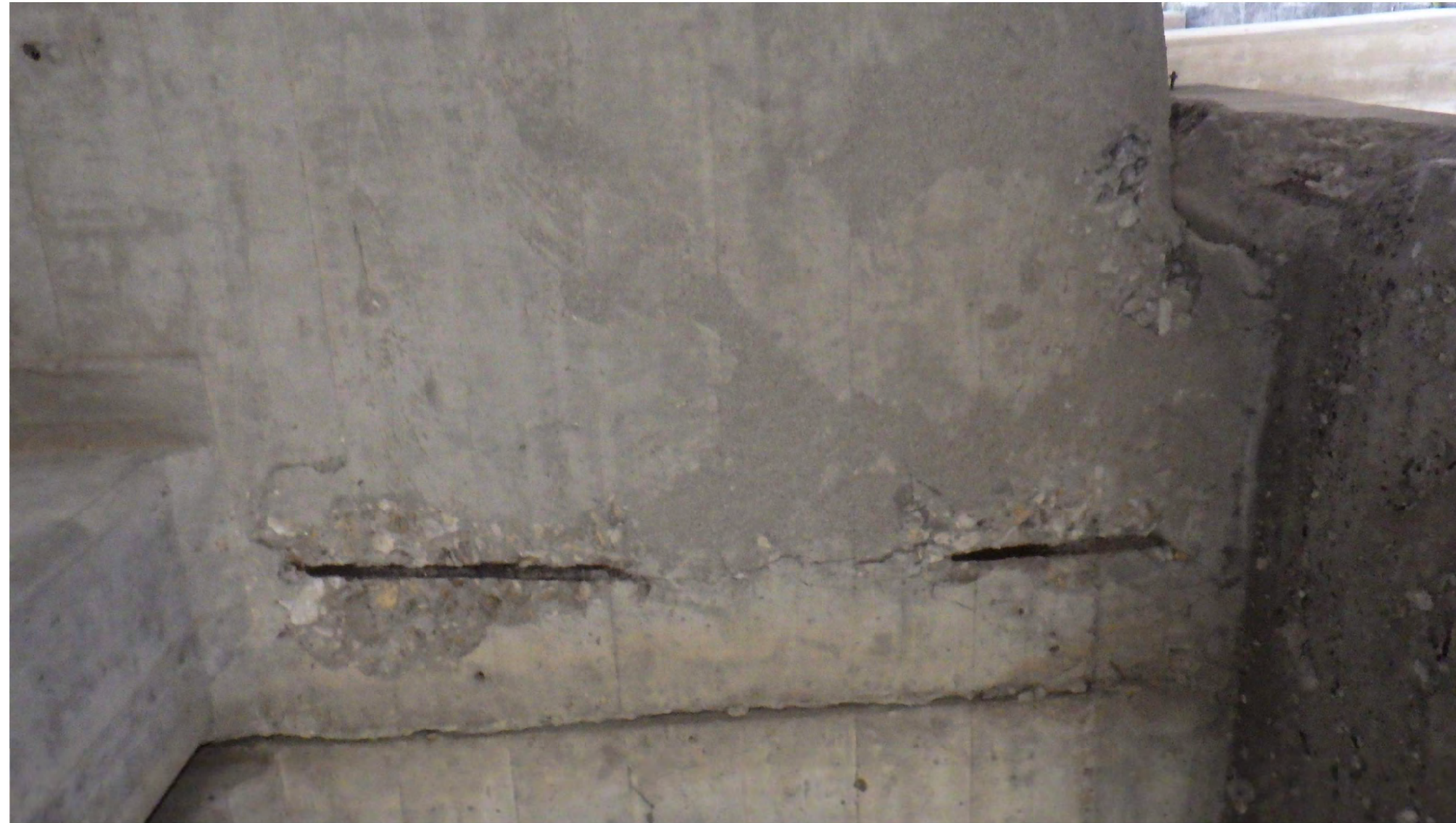
EXAMPLE OF SPAN 6 SPALL DAMAGE
