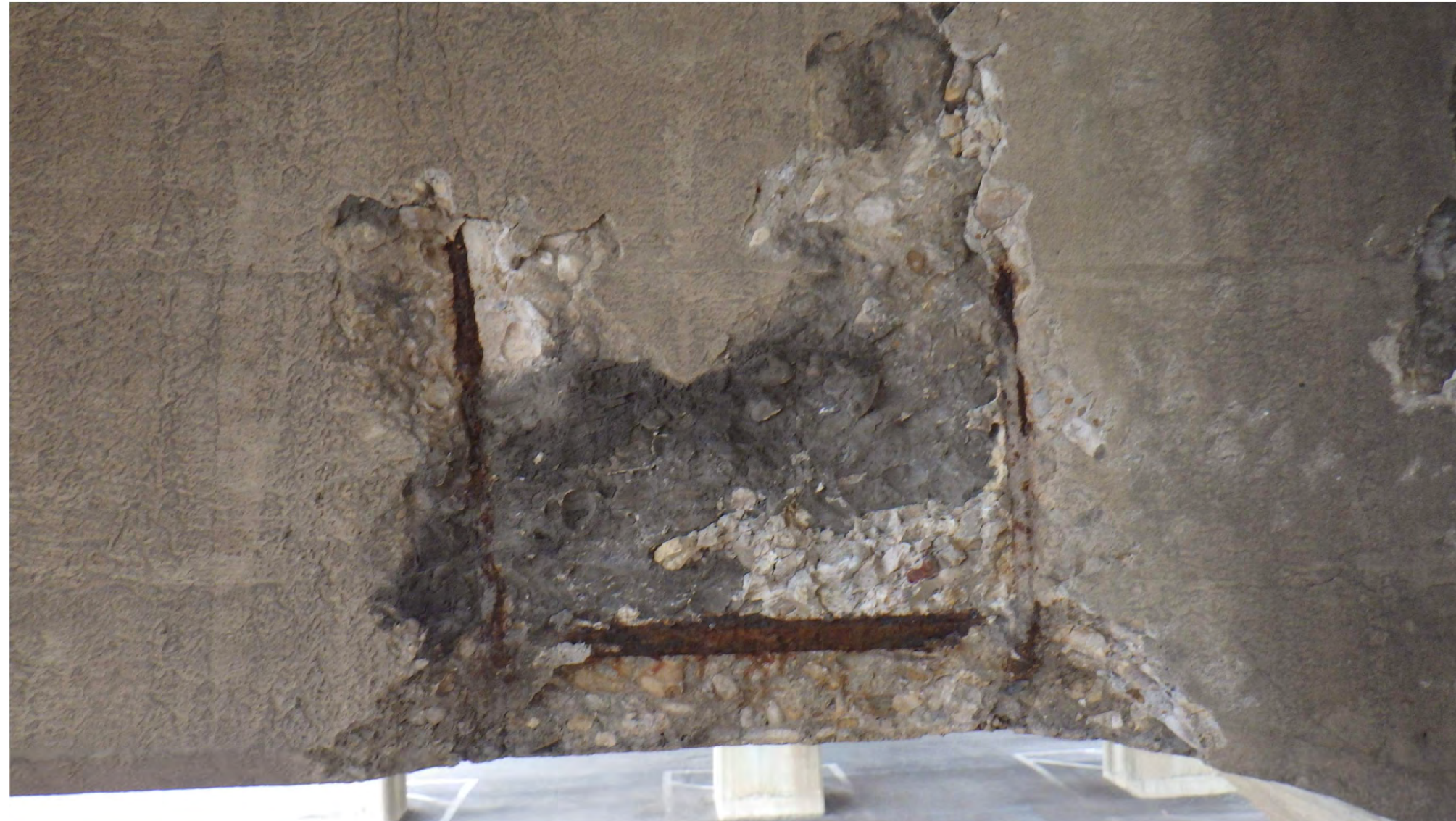
EXAMPLE OF PIER 7 SPALL DAMAGE
