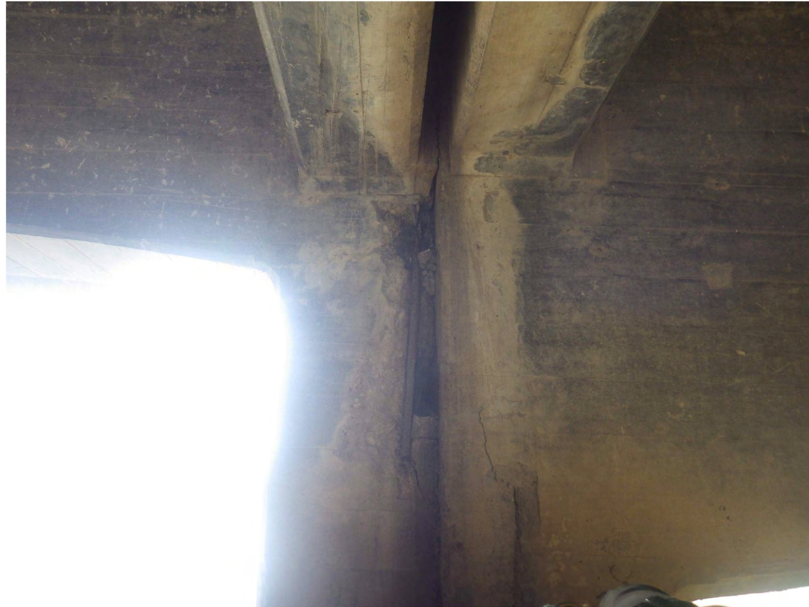
EXAMPLE OF SPAN 13 SPALL DAMAGE
