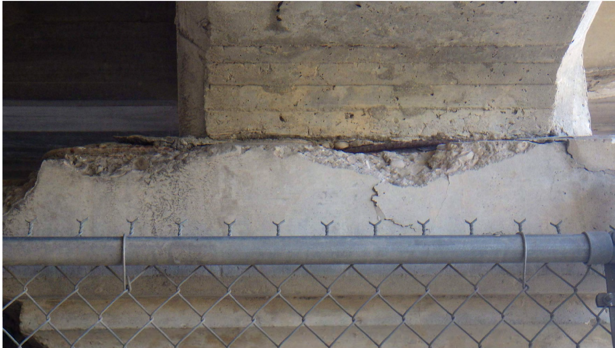
EXAMPLE OF PIER 1 SPALL DAMAGE
