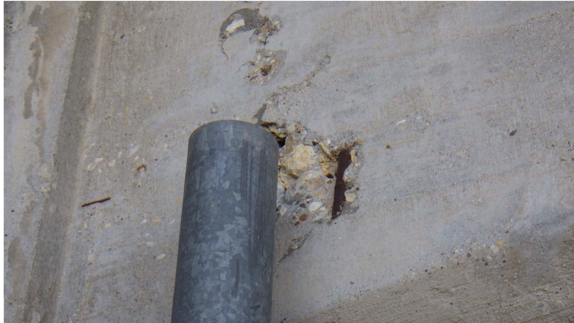
EXAMPLE OF SPAN 1 SPALL DAMAGE
