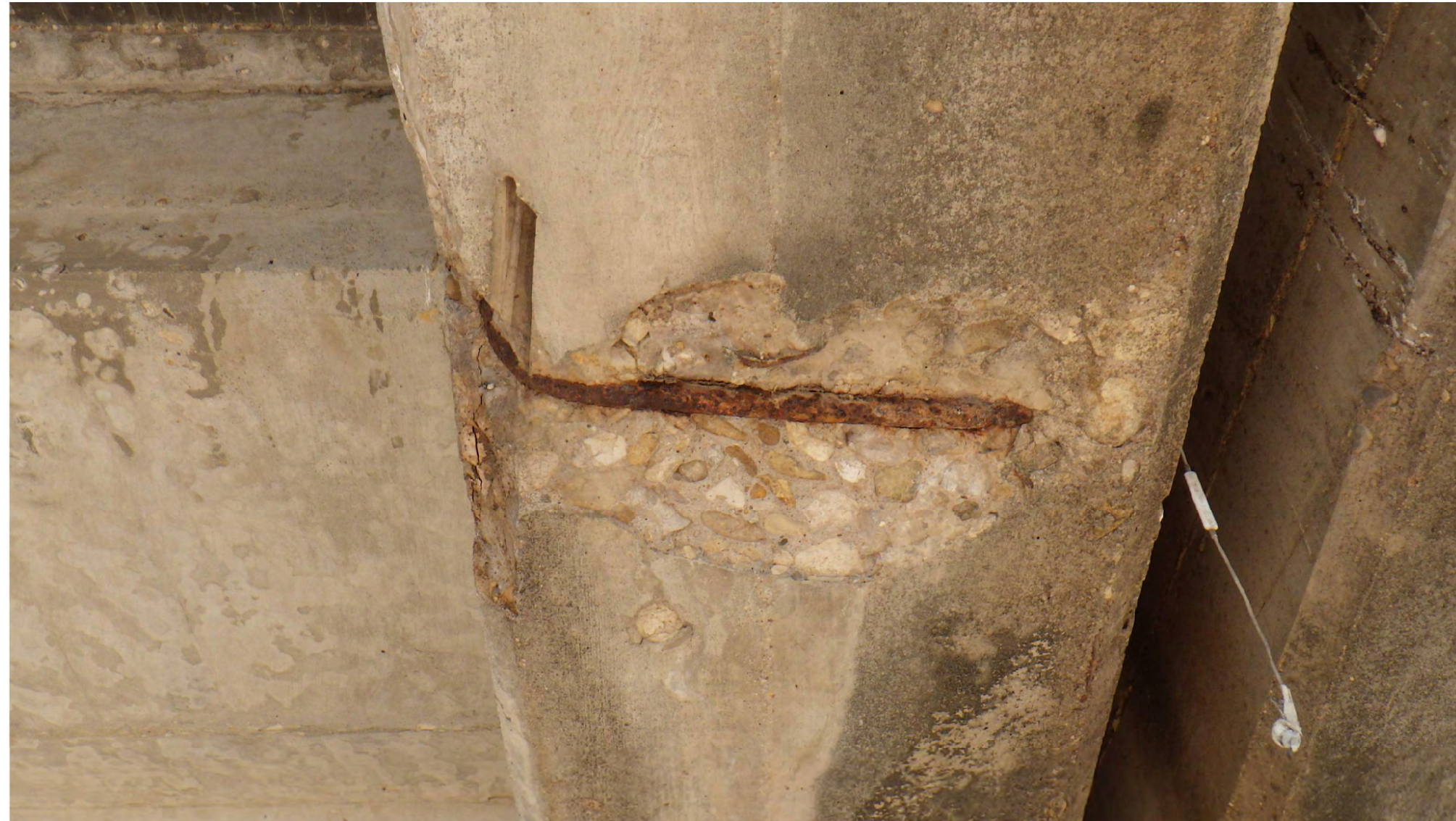
EXAMPLE OF SPAN 3 SPALL DAMAGE
