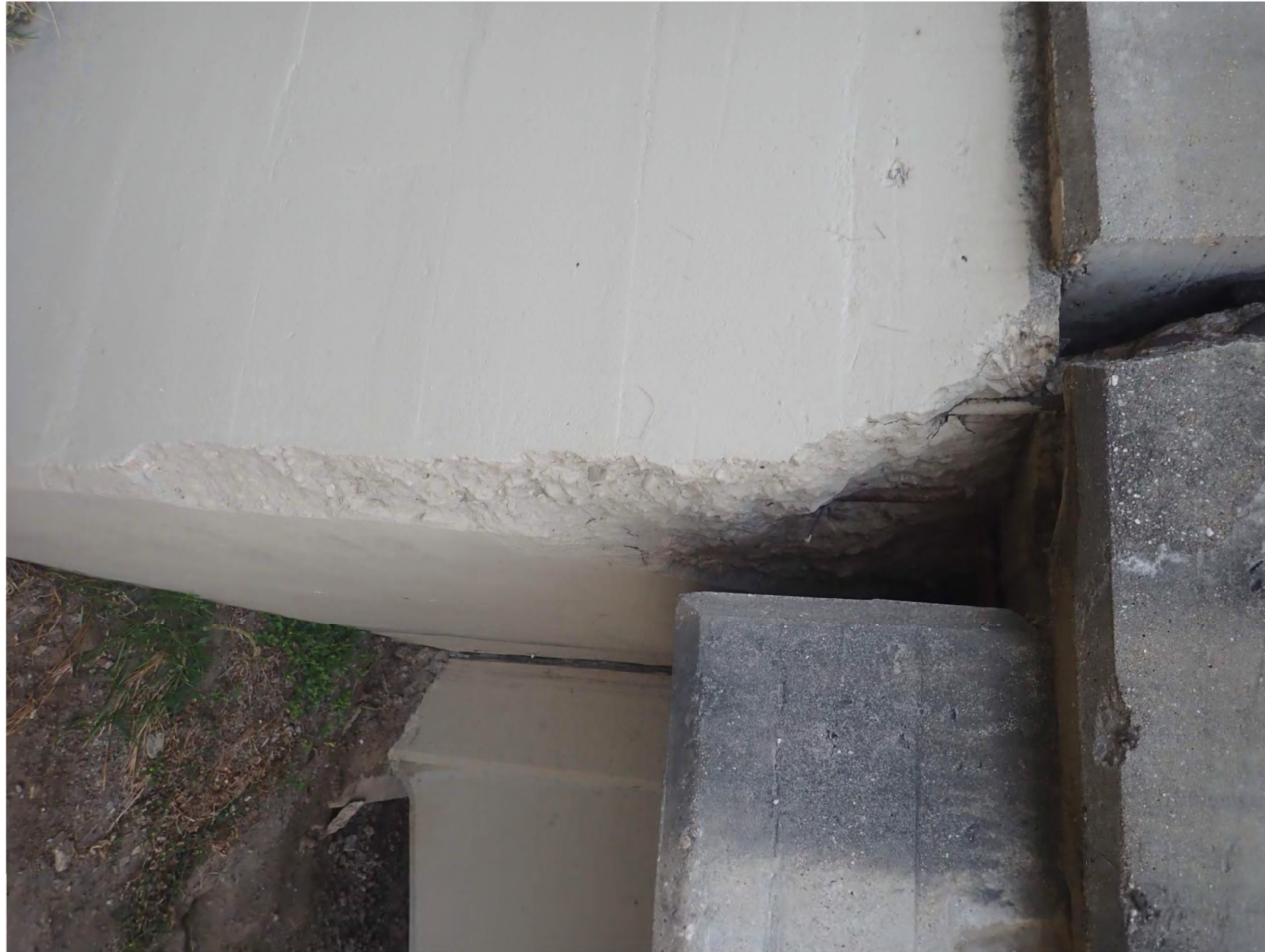
EXAMPLE OF NORTH ABUTMENT SPALL DAMAGE
