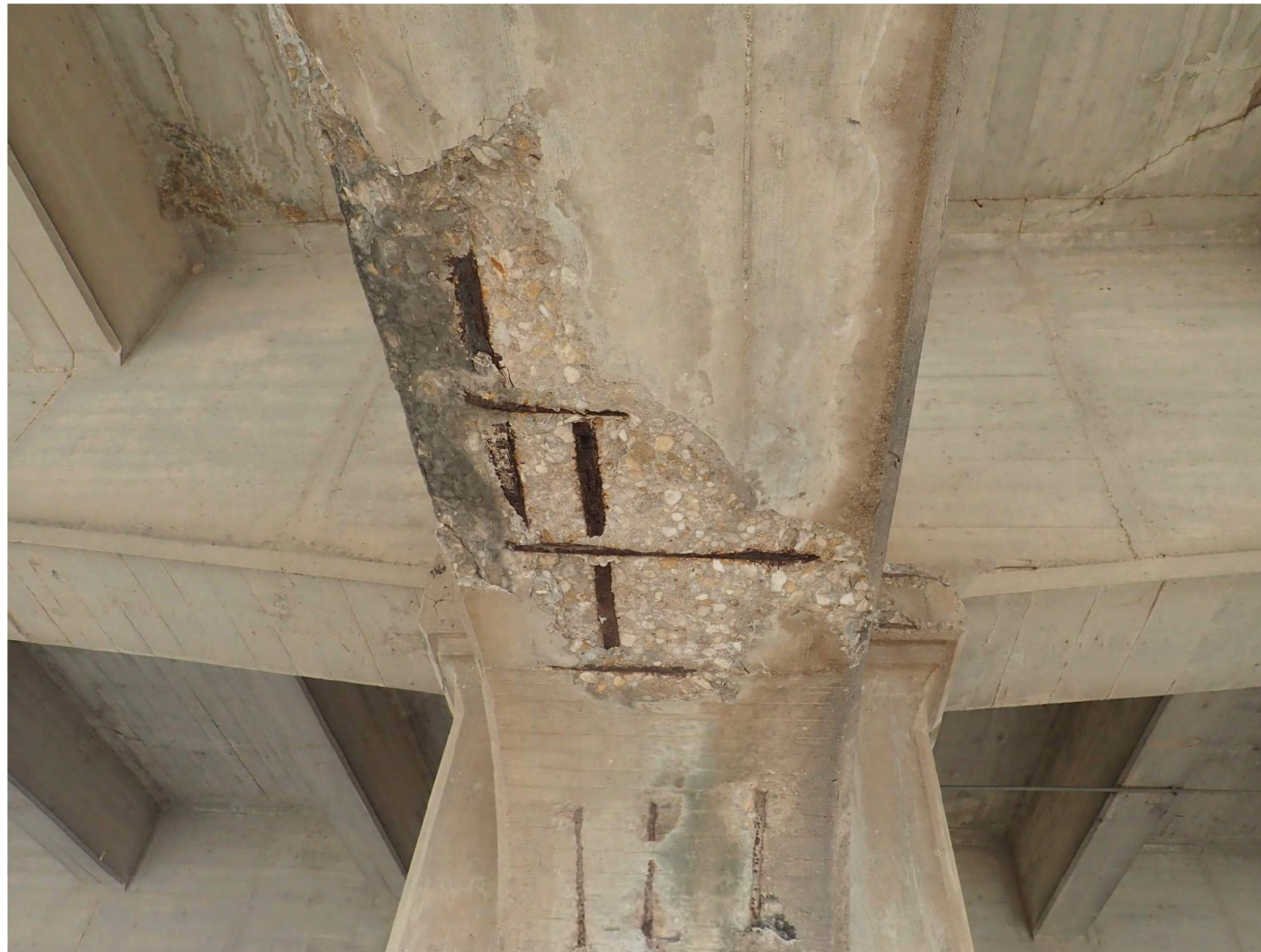
EXAMPLE OF PIER 8 SPALL DAMAGE
