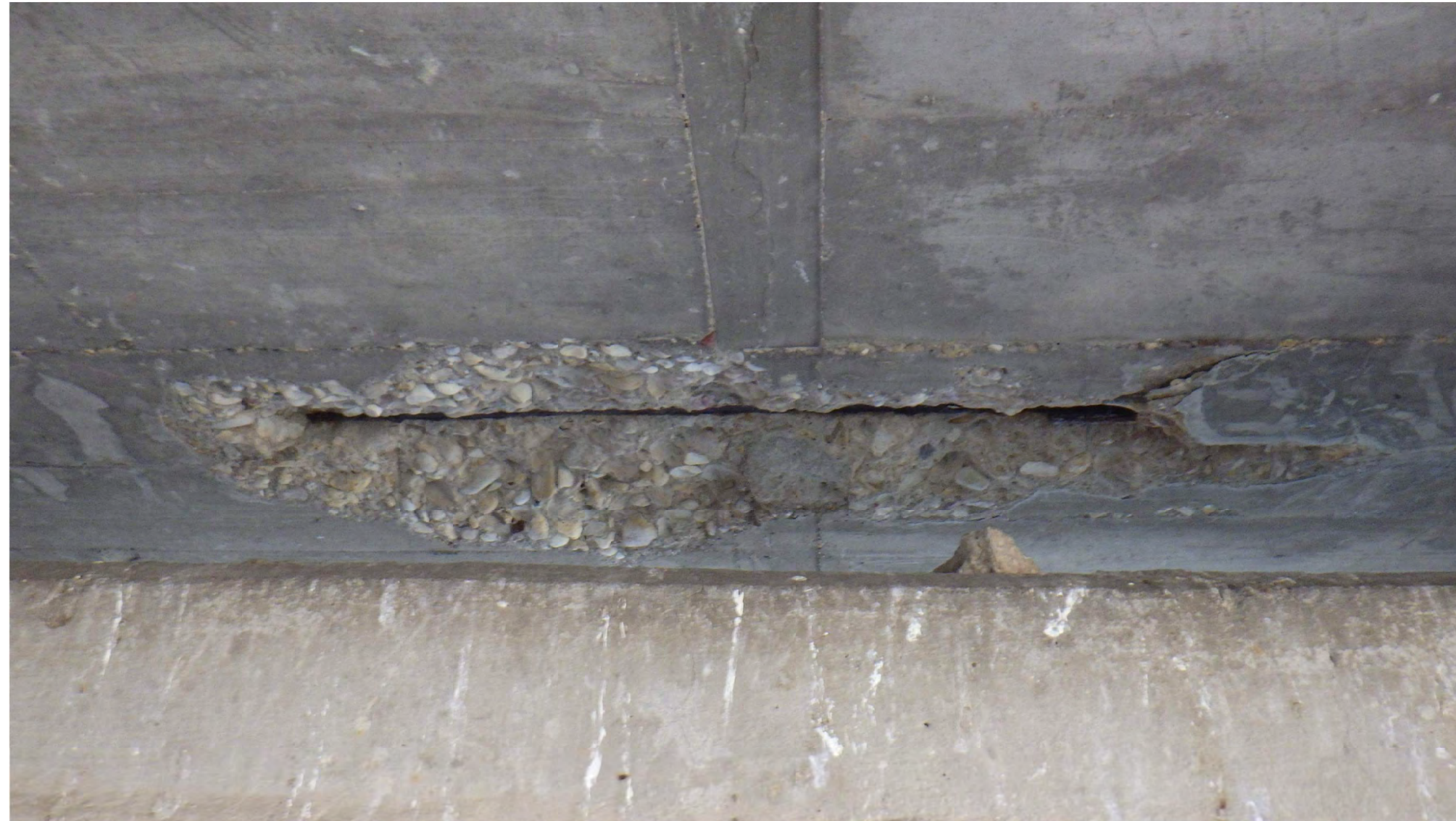
EXAMPLE OF SPAN 8 SPALL DAMAGE
