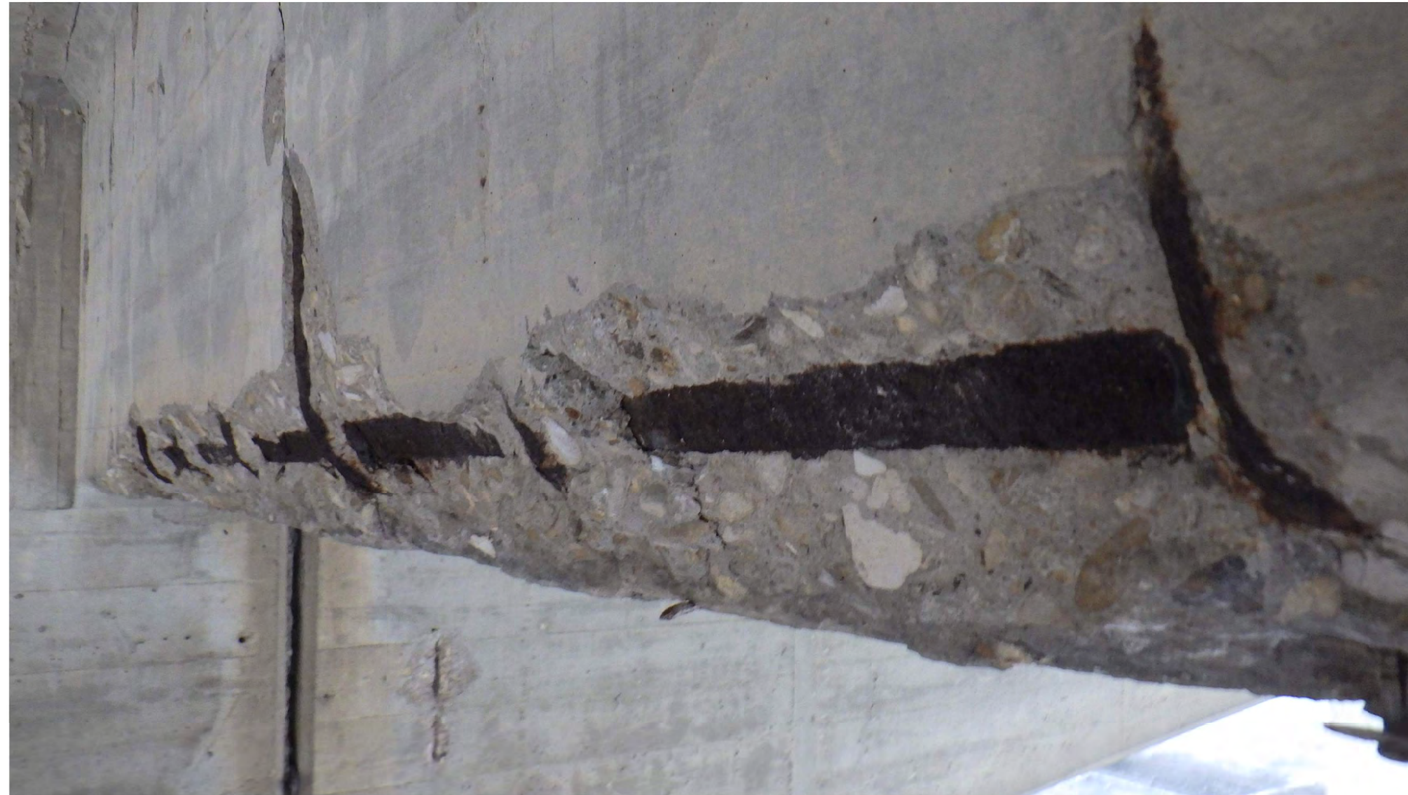
EXAMPLE OF SPAN 7 SPALL DAMAGE
