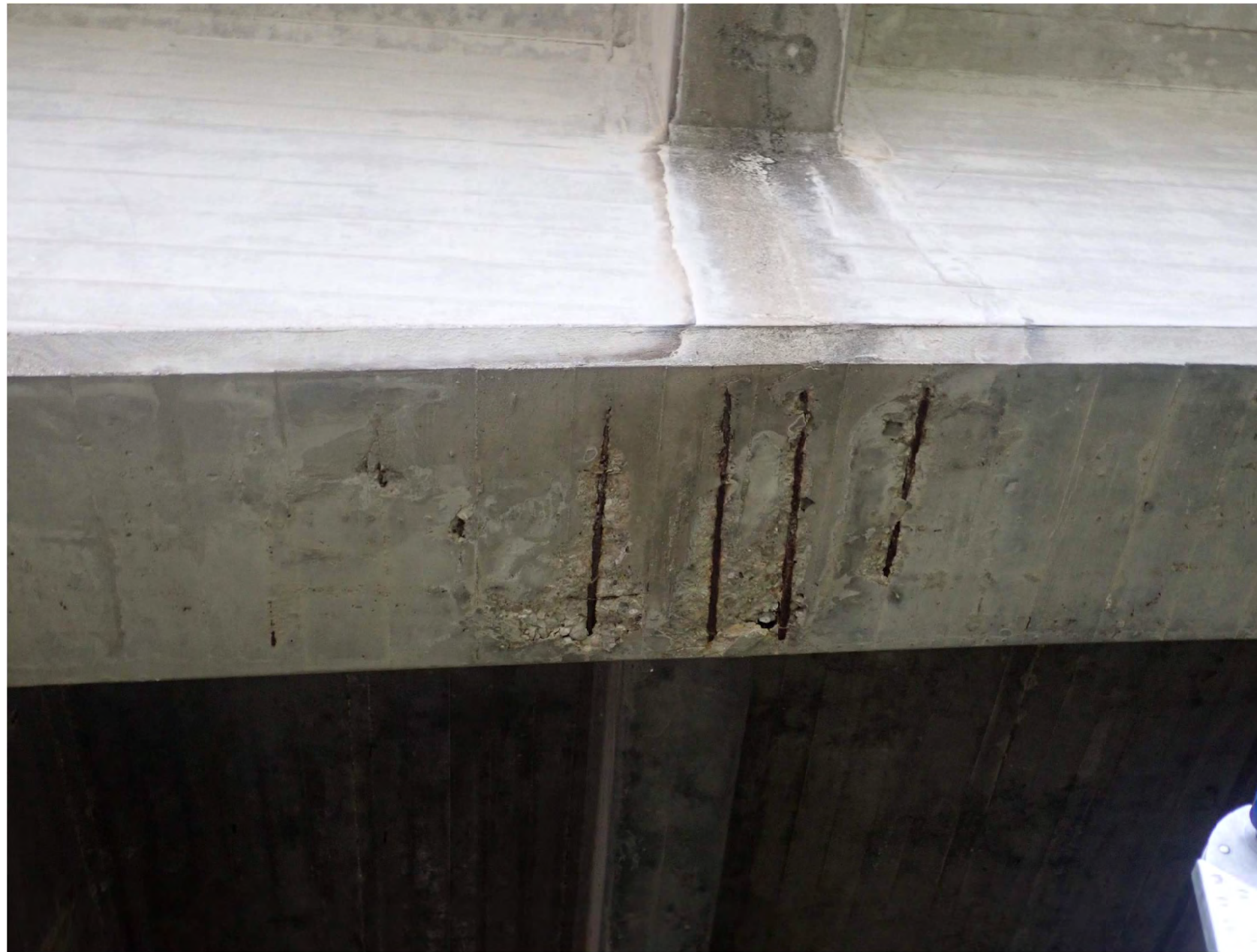
EXAMPLE OF SPAN 15 SPALL DAMAGE
