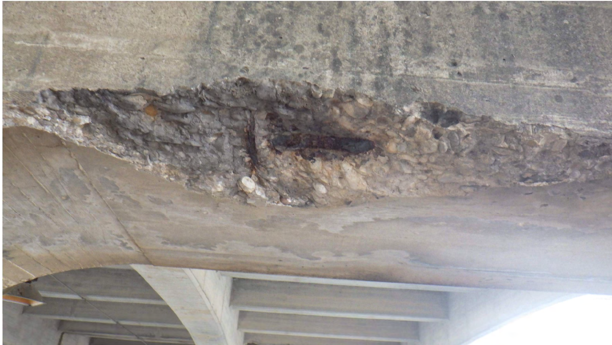
EXAMPLE OF PIER 6 SPALL DAMAGE
