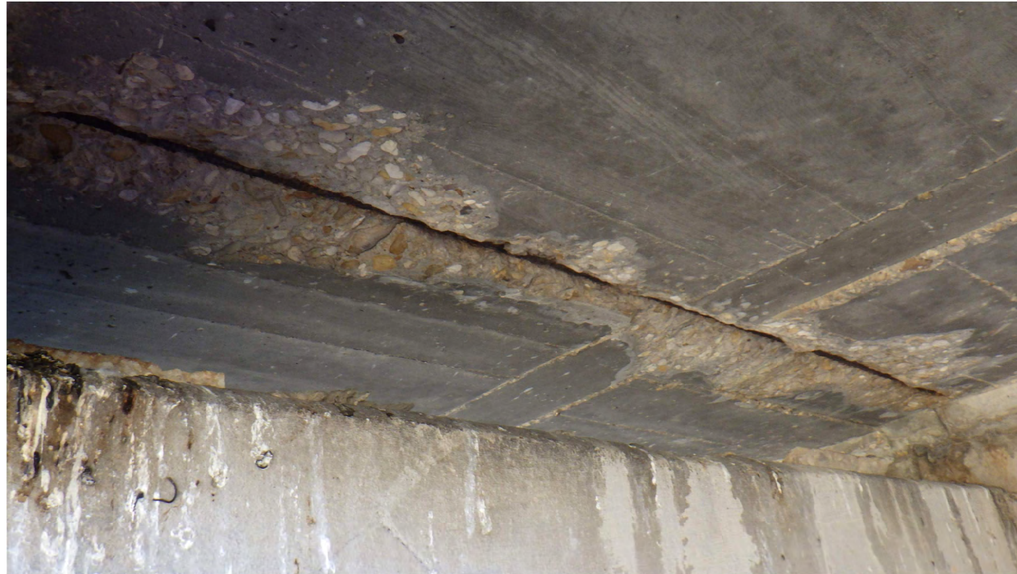
EXAMPLE OF SPAN 4 SPALL DAMAGE
