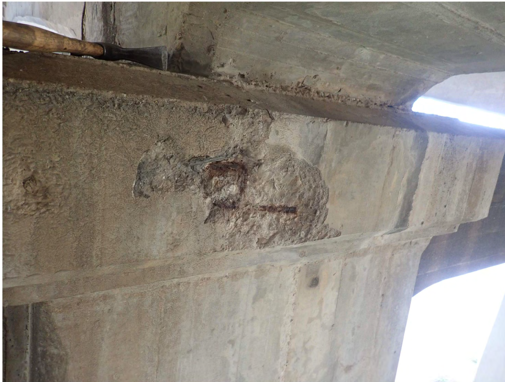
EXAMPLE OF PIER 14 SPALL DAMAGE
