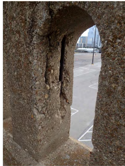
Typical spall damage at post
