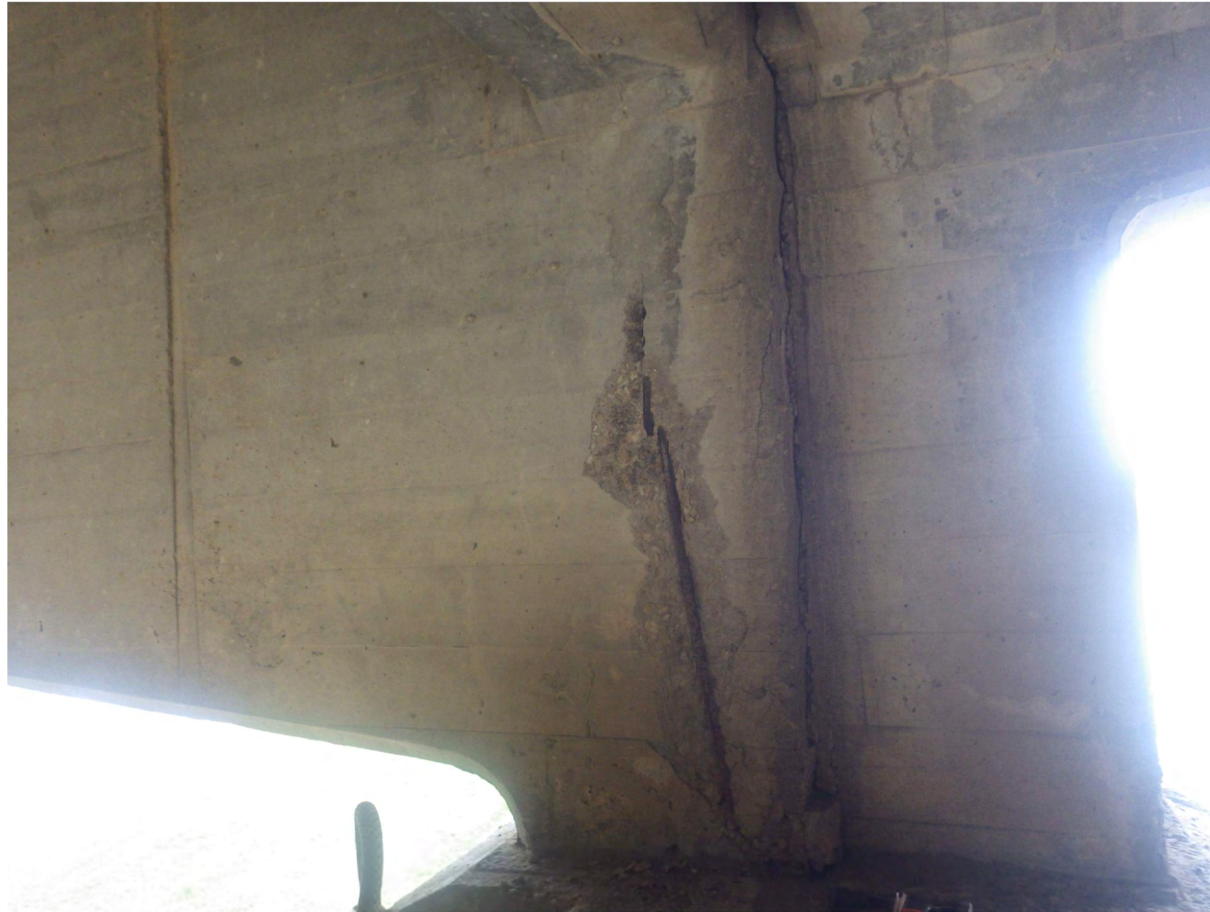
EXAMPLE OF SPAN 11 SPALL DAMAGE
