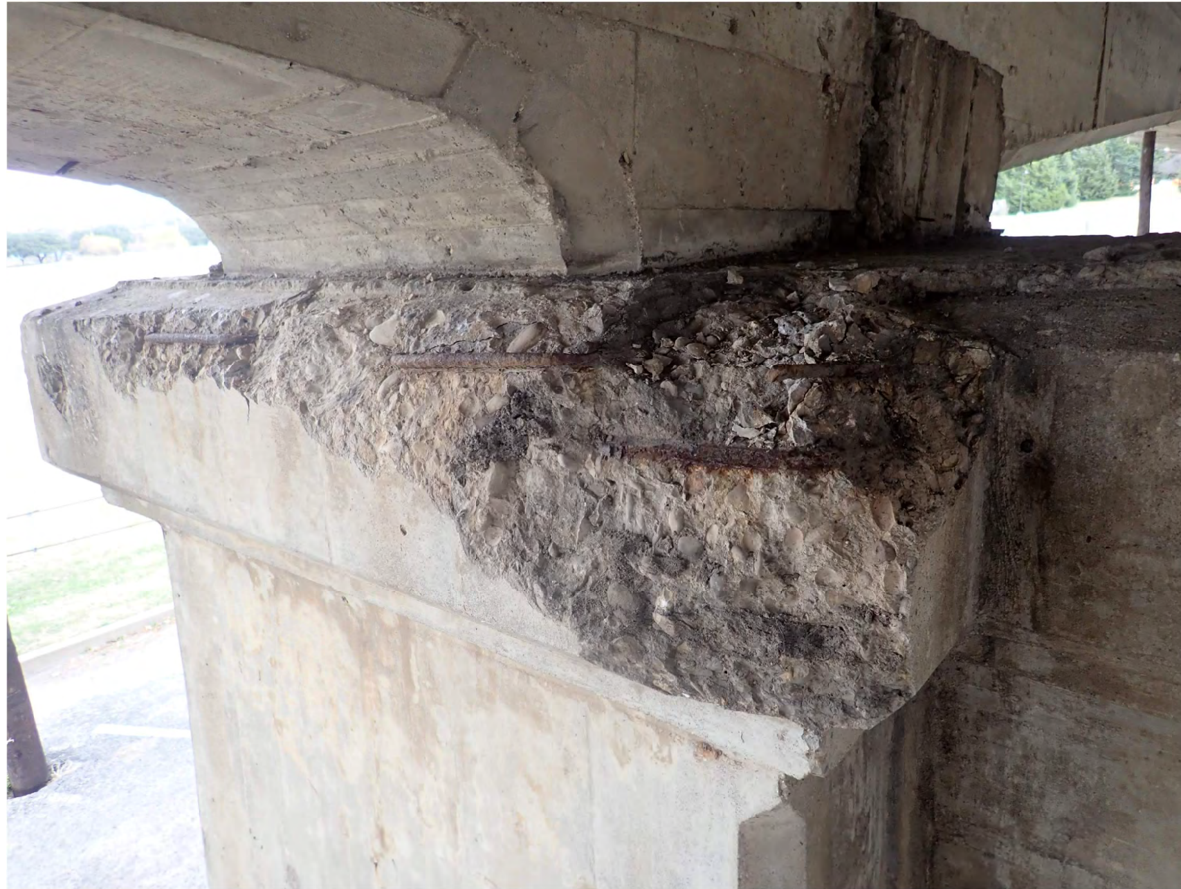
EXAMPLE OF PIER 5 SPALL DAMAGE
