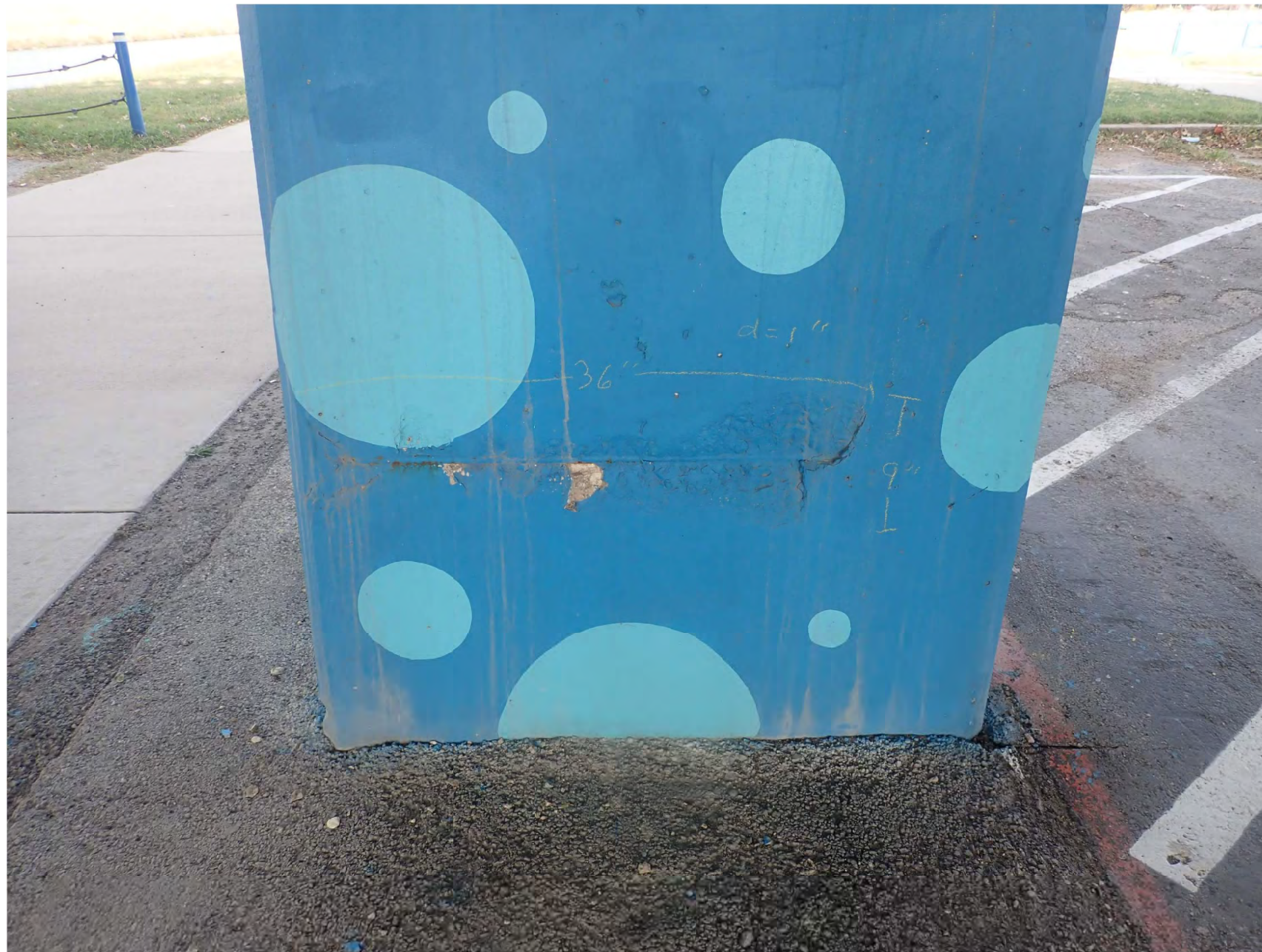
EXAMPLE OF PIER 9 SPALL DAMAGE
