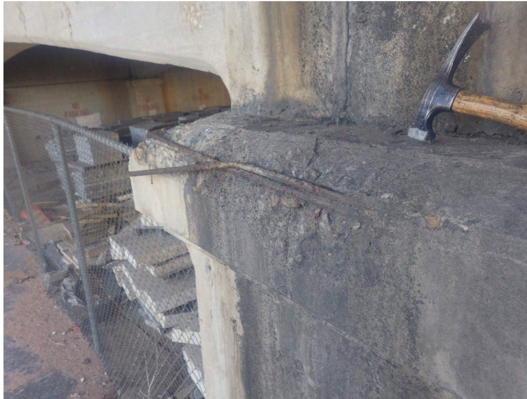
EXAMPLE OF PIER 2 SPALL DAMAGE
