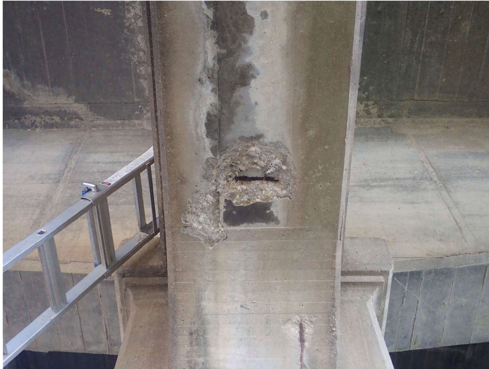
EXAMPLE OF PIER 13 SPALL DAMAGE
