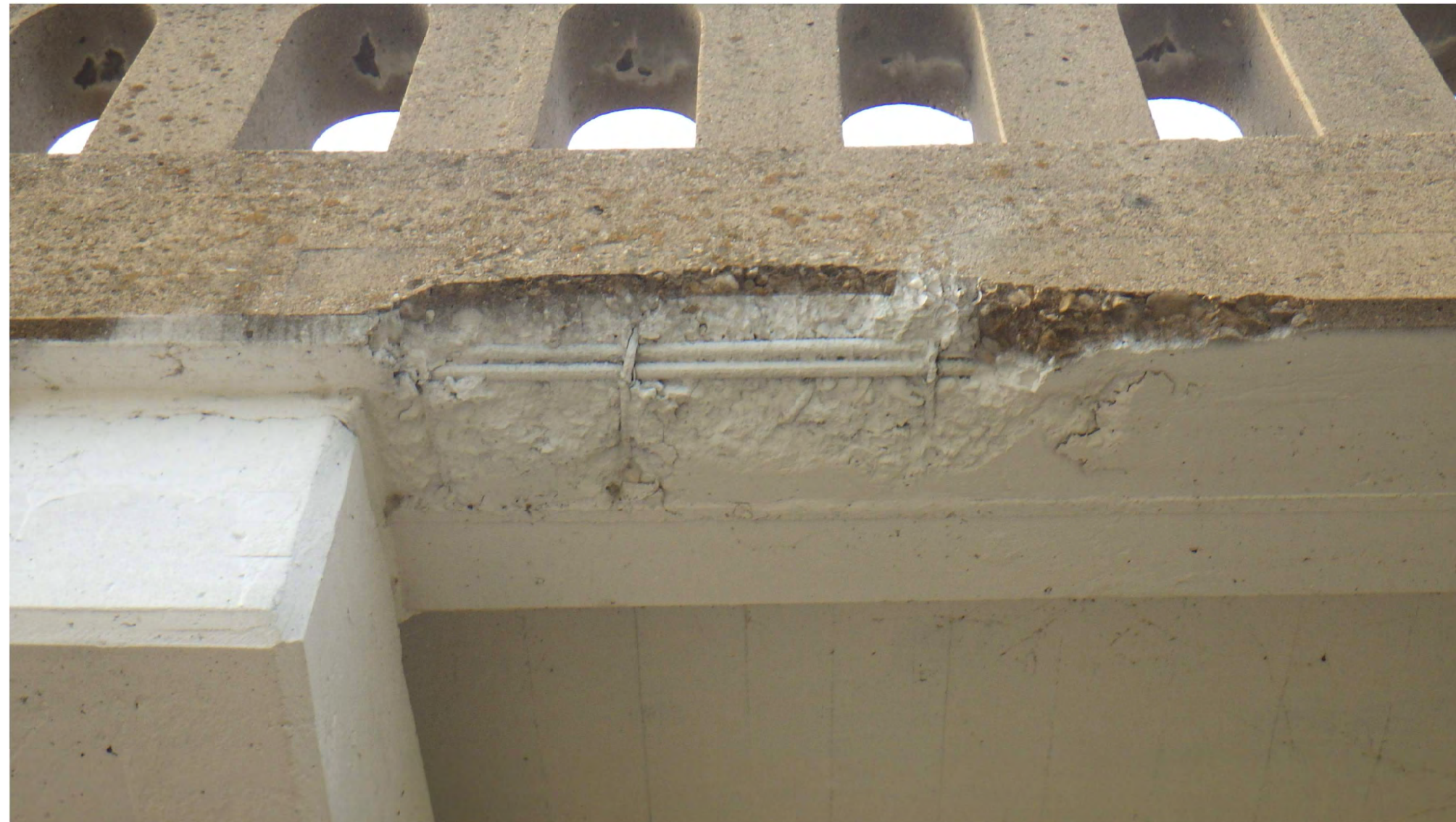
EXAMPLE OF SPAN 10 SPALL DAMAGE
