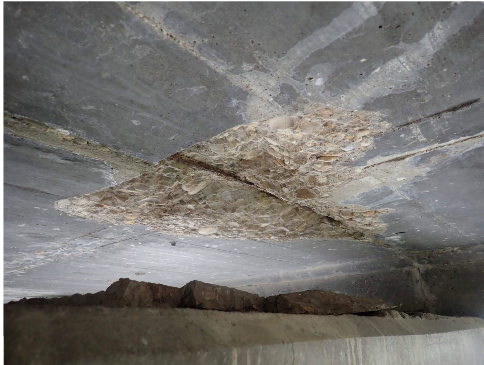
EXAMPLE OF SPAN 14 SPALL DAMAGE
