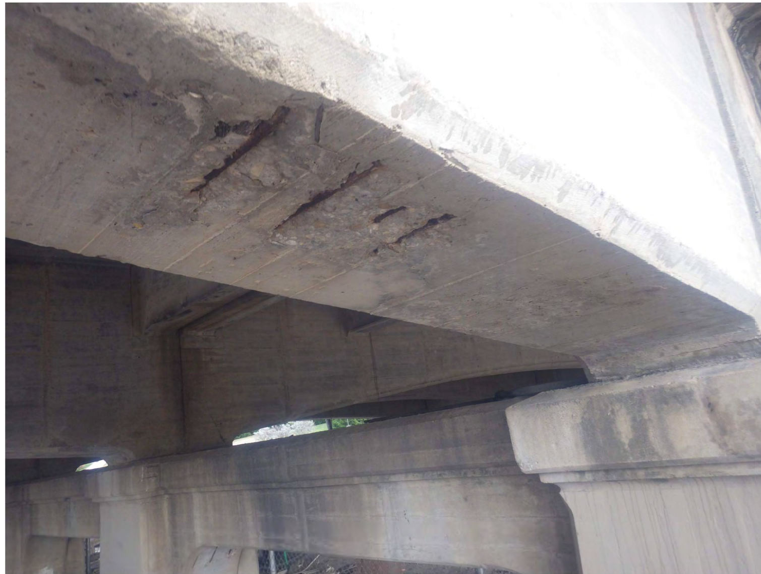
EXAMPLE OF SPAN 2 SPALL DAMAGE
