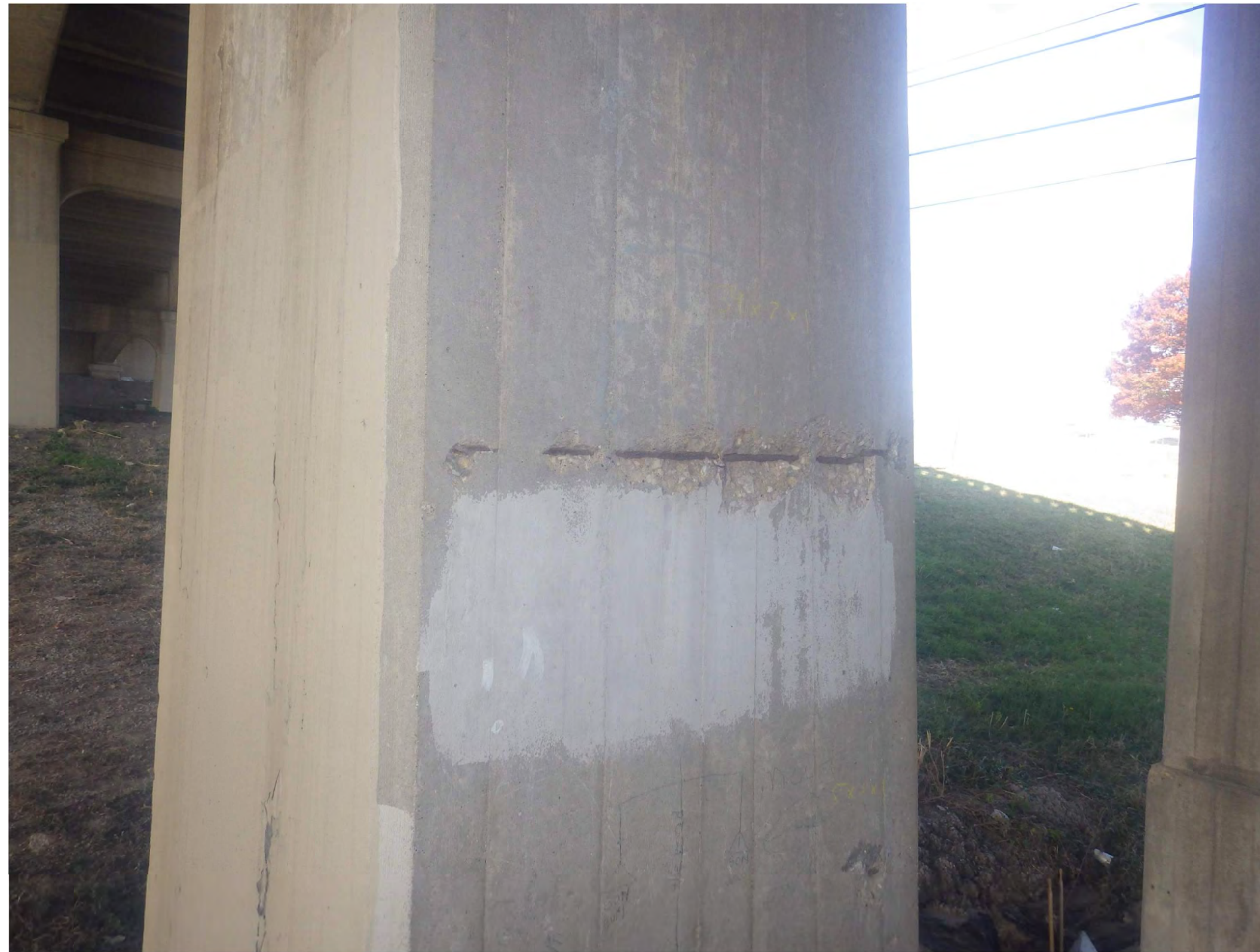
EXAMPLE OF PIER 12 SPALL DAMAGE
