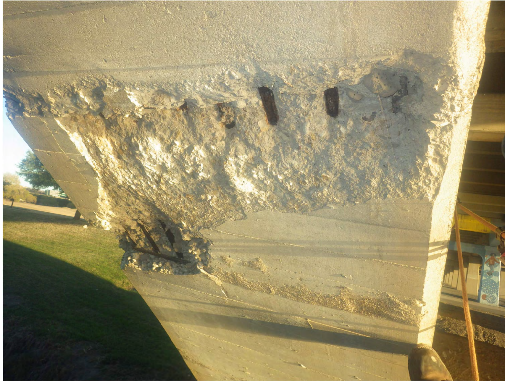
EXAMPLE OF SPAN 12 SPALL DAMAGE
