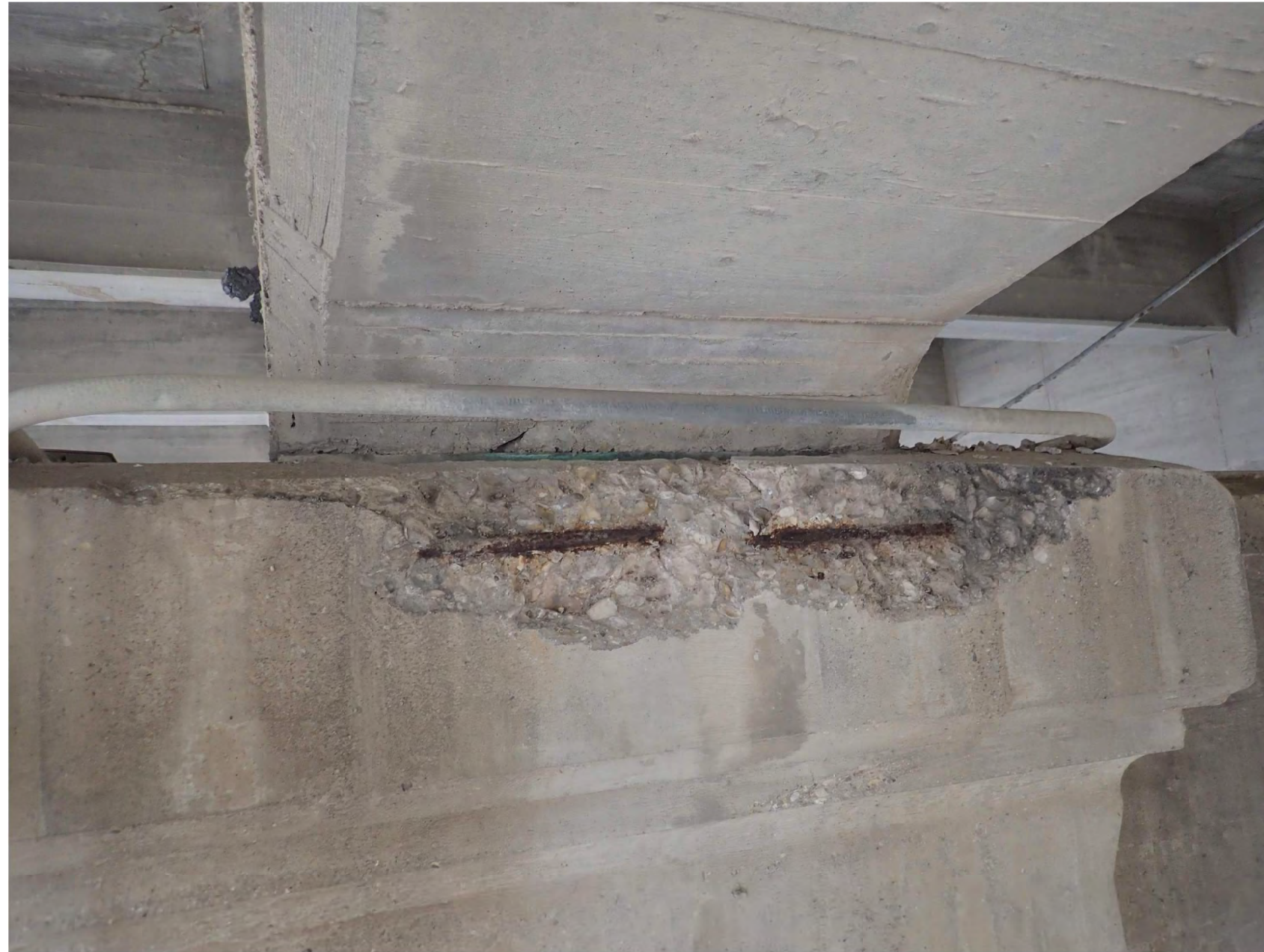
EXAMPLE OF PIER 4 SPALL DAMAGE
