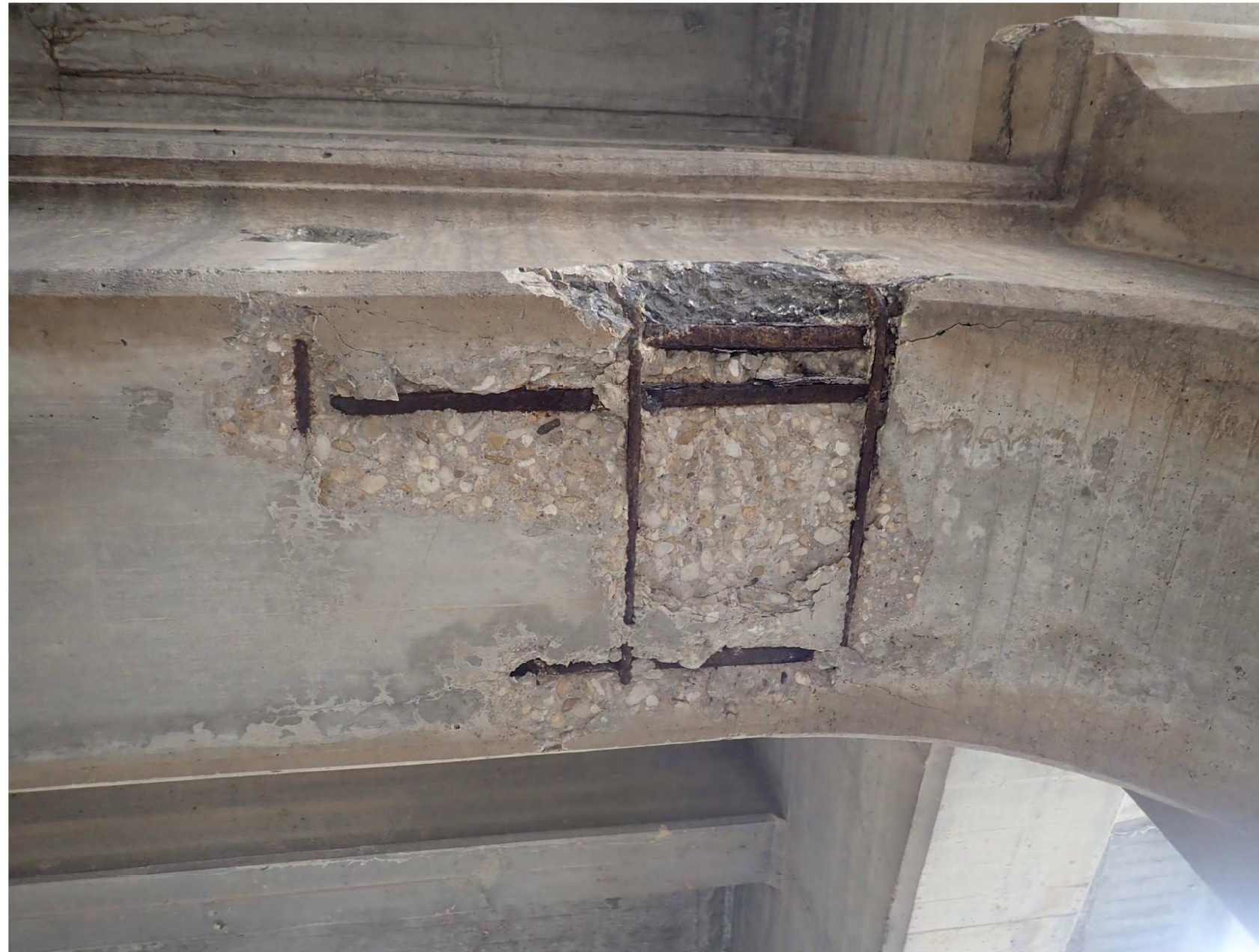
EXAMPLE OF PIER 3 SPALL DAMAGE
