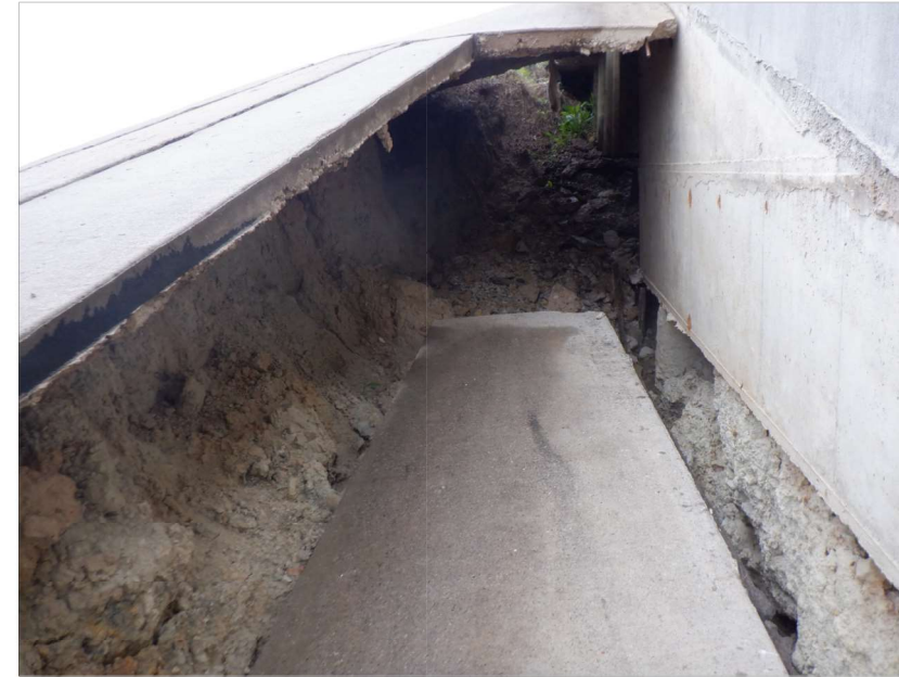
PHOTO 2 (VIEW OF FAILED RIPRAP AND ERODED AREA NEAR NORTHWEST WINGWALL, LOOKING NORTHWEST)
