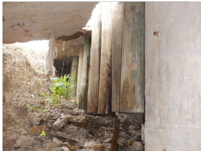
PHOTO 3 (VIEW OF EROSION UNDER CONCRETE RIPRAP, MOW STRIP AND THRIE-BEAM TRANSITION NEAR NORTHWEST WINGWALL, LOOKING NORTH)
