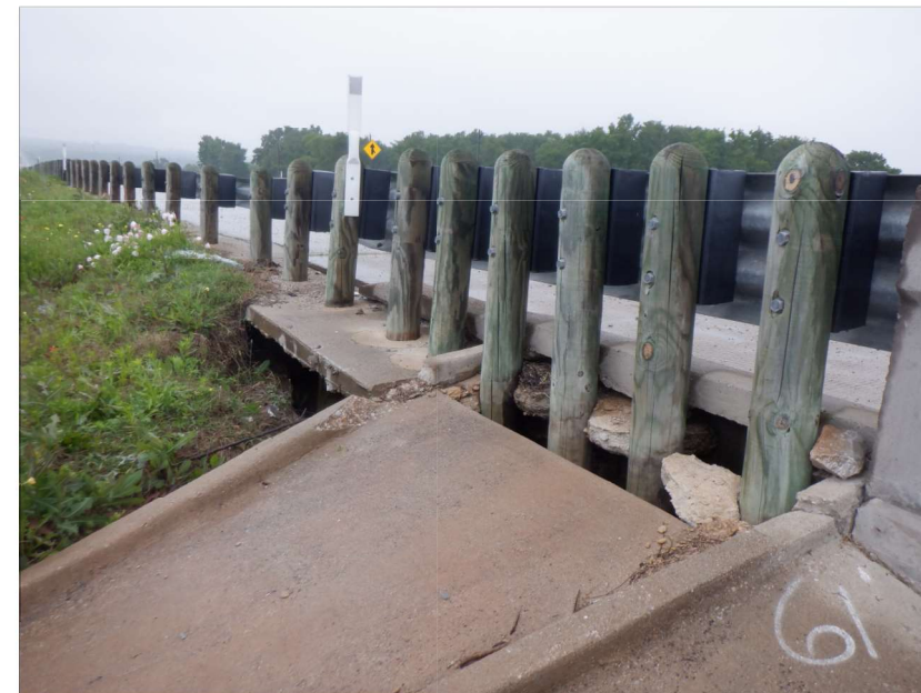
PHOTO 4 (VIEW OF CRACKED AND DAMAGED CURB AT THRIE BEAM TRANSITION, CONC FLUME AND MOW STRIP, LOOKING NORTH)
