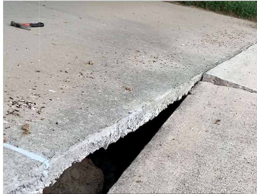
PHOTO 1 (VIEW OF EXPOSED EROSION UNDER RIPRAP AT ABUTMENT #4, LOOKING EAST)
