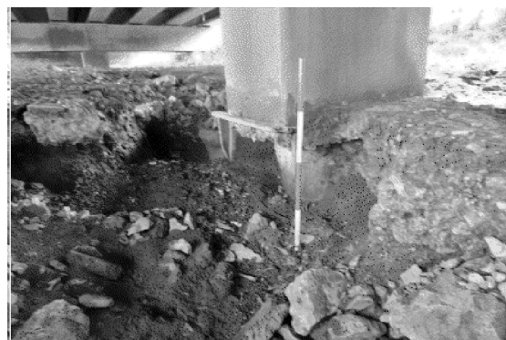
NORTHEAST BANK EROSION
