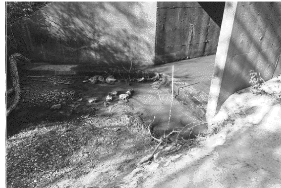
NORTHWEST WINGWALL EROSION
