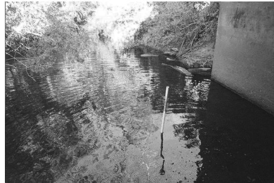
EROSION UPSTREAM END
