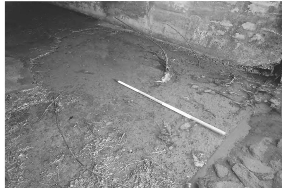
NOTE: 1. Bottom slab has widespread moderate delaminations and spalls with exposed heavily rusted rebar.
