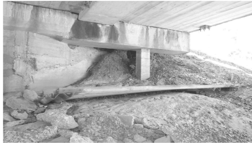
FAILED STEEL BACKWALL AT NORTHWEST END OF SOUTHWEST ABUTMENT CAP LOOKING SOUTHWEST
