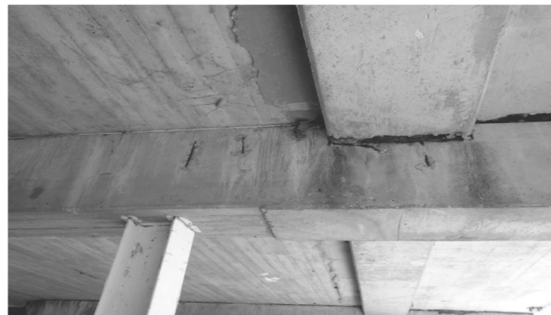
COVER SPALLS WITH EXPOSED REBAR AT INTERIOR BENT CAP LOOKING NORTHEAST
