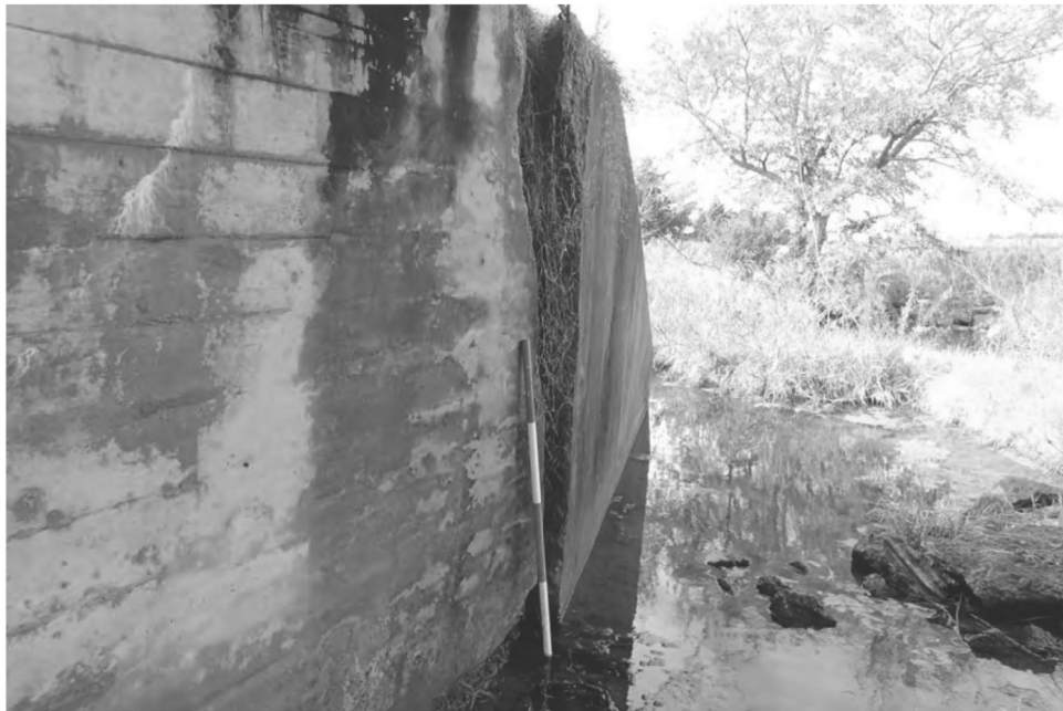
NOTE: 1. The southwest wingwall has separated from the culvert and has rotated a maximum of 7" at the top due to embankment pressure. The southwest wingwall has settled up to 2" at the end.
