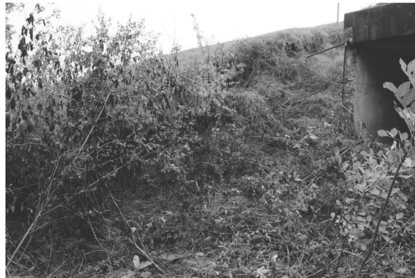
NOTE: North wingwall has failed and is laying in channel.
