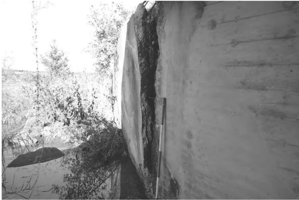
NOTE: 1. The northwest wingwall has separated from the culvert and has rotated a maximum of 7" at the top due to embankment pressure.
