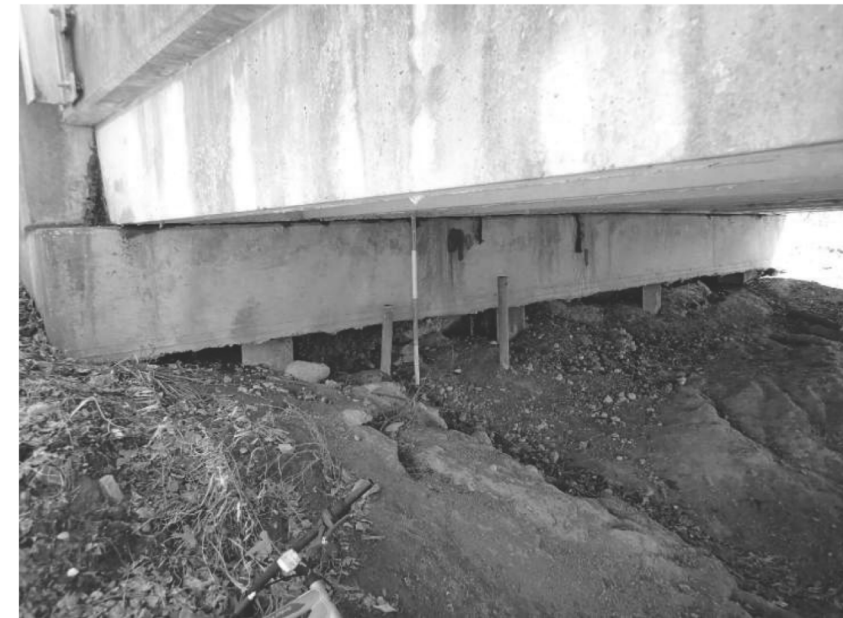
Erosion at top of banks has fully undermined both abutment caps exposing the steel piles
