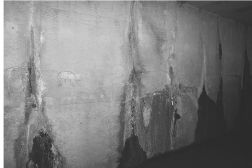
NOTE: Abutment walls have minor horizontal cracks (up to 0.040" wide) and minor to moderate vertical cracks (up to 5/16" wide) with heavy efflorescence.
