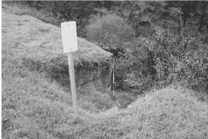
NOTE: Embankment at north corner has an area of erosion 10' x 7' x 5' deep due to wingwall failure.
