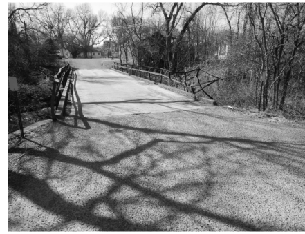
Superstructure with damaged rails
