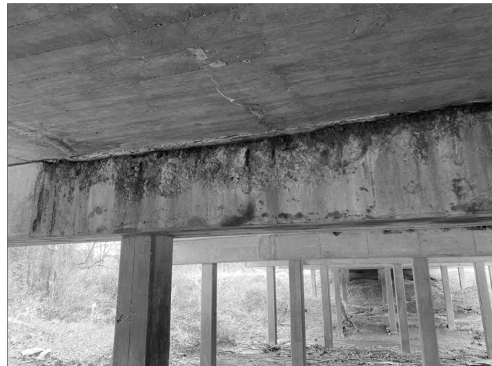
TYPICAL SPALLING AT BENTS 3, 5, 7, 9 (SB1)
