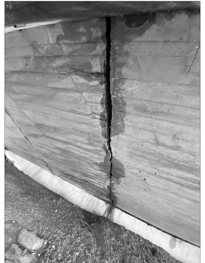
CRACK ON UNDERSIDE OF DECK AT MIDSPAN (SP1)
