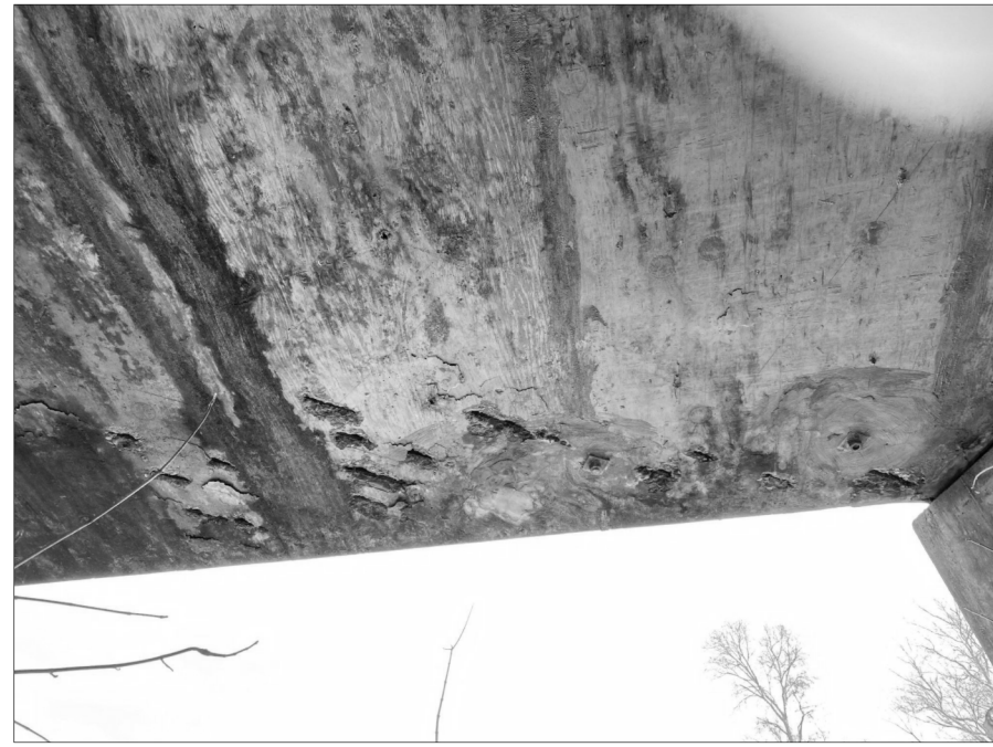
TYPICAL SPALLS AND DELAMINATIONS AT UNDERSIDE OF DECK (SP1)
