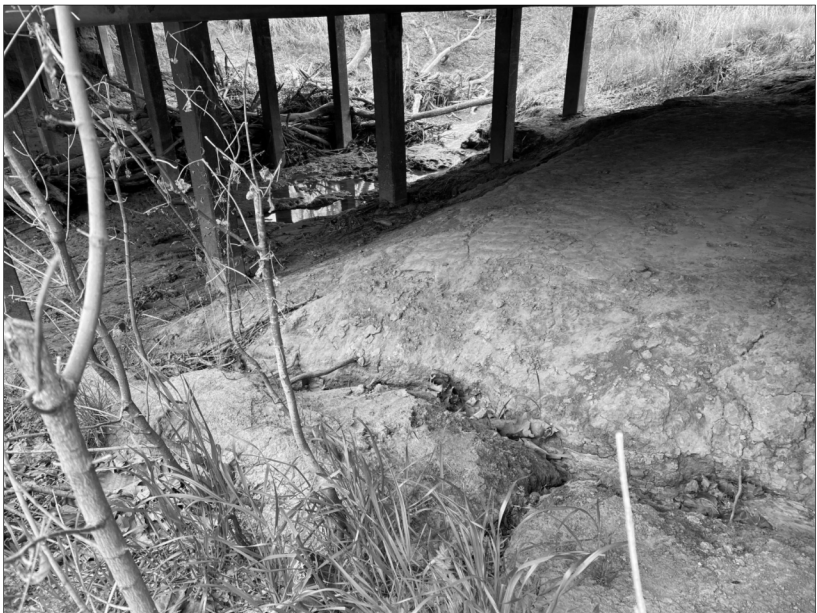
EROSION GULLY ON NE SIDE (M3)
