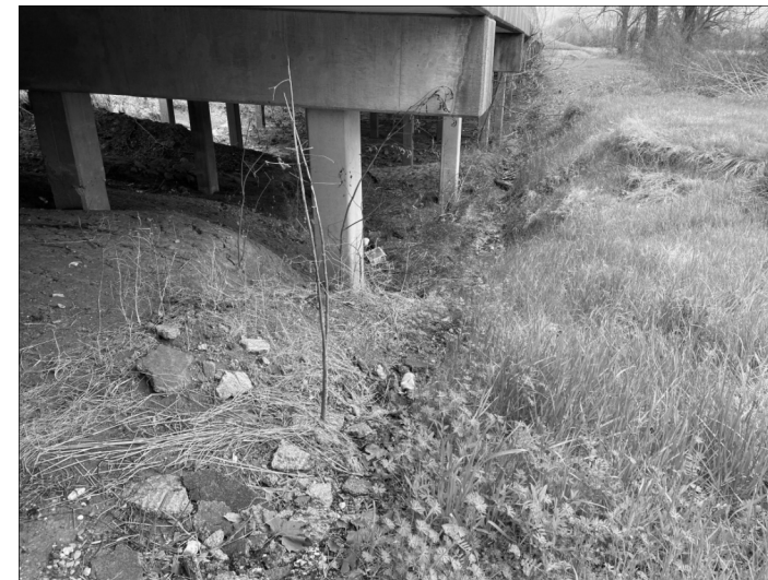
EROSION GULLY AT NW CORNER (M1)
