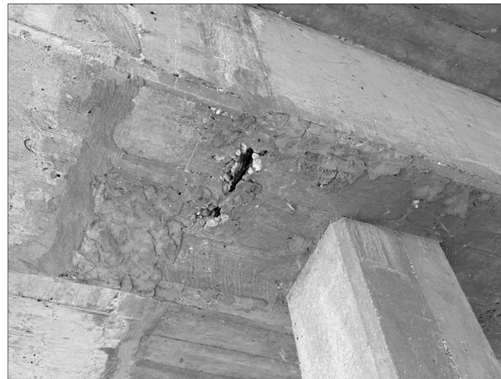
MINOR SPALL AT BENT 6 CAP (SB2)
