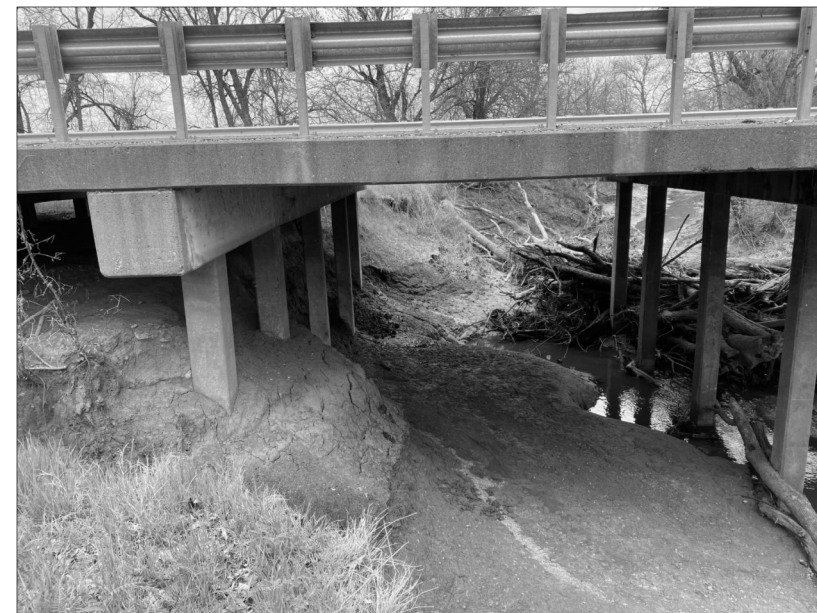
TYPICAL CHANNEL BANK EROSION (M2)
