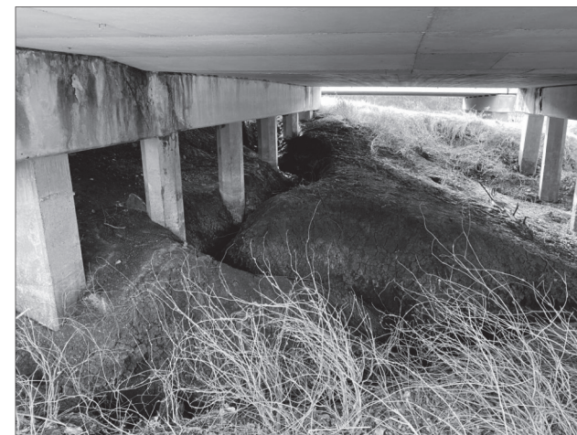
EROSION GULLY (M1)
