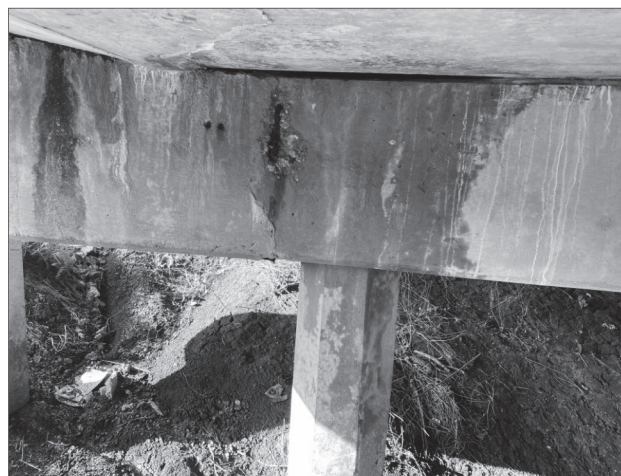
MINOR SPALL ON BENT 7 CAP (SB2)
