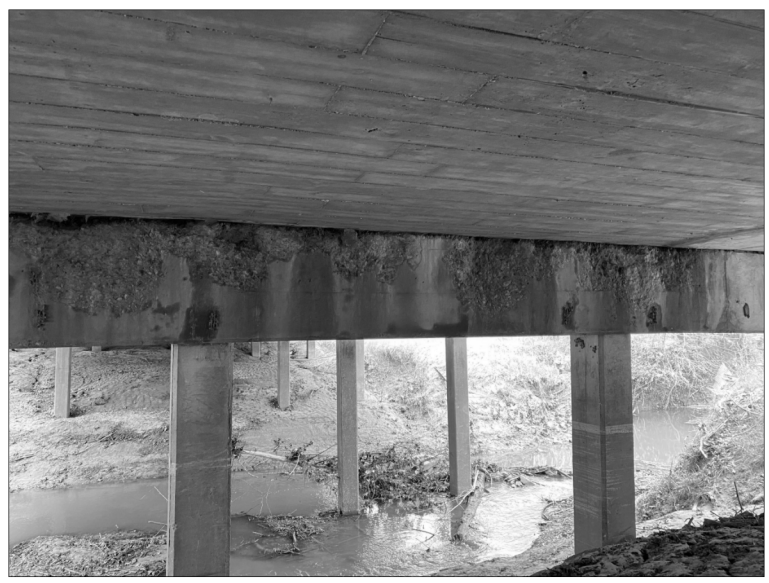
TYPICAL BENT CAP SPALL (SB1)
