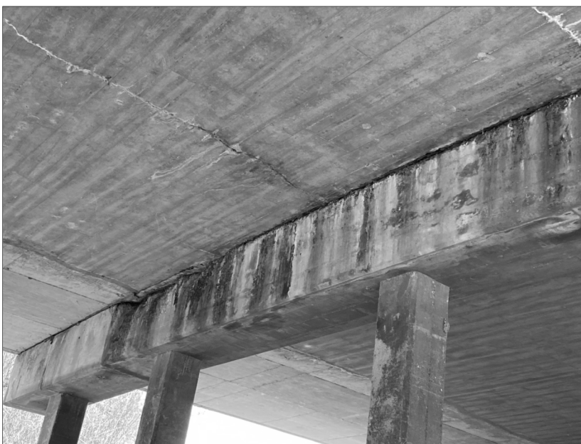
TYPICAL BENT CAP SPALLS (SB1)
