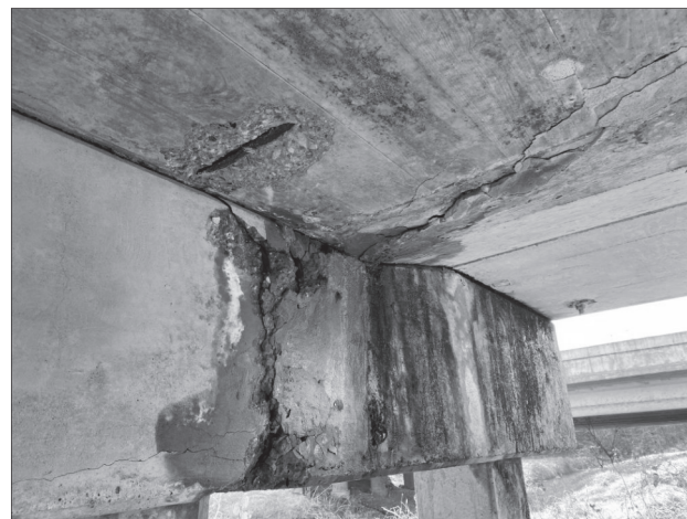
TYPICAL BENT CAP SPALL (SB1) AND MINOR SPALL AT UNDERSIDE OF DECK (SP1)
