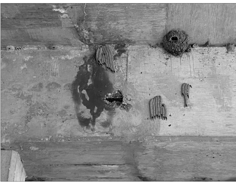
MINOR SPALL ON BENT 5 CAP (SB2)
