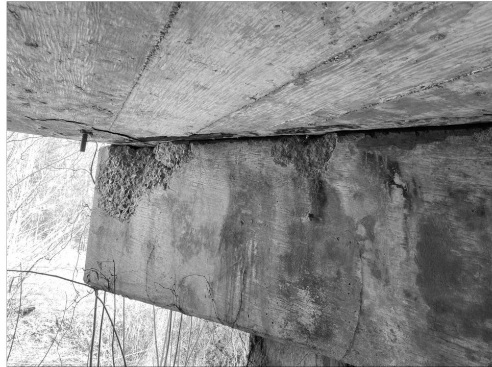
TYPICAL BENT 2 CAP SPALL
