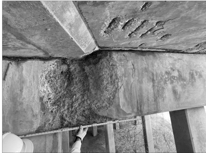
BENT 4 CAP SPALL (SB1)
