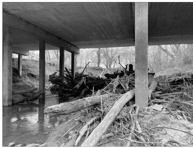
DRIFT AND DEBRIS IN SPAN 5 (M1)
