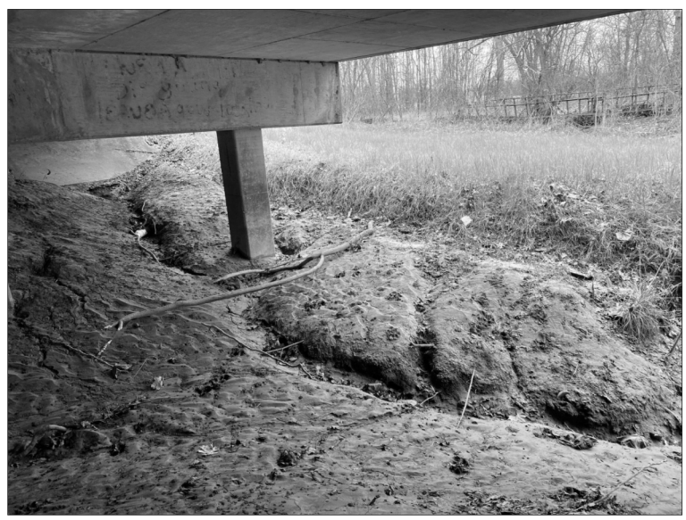
TYPICAL EROSION GULLY ON WEST END (M1)
