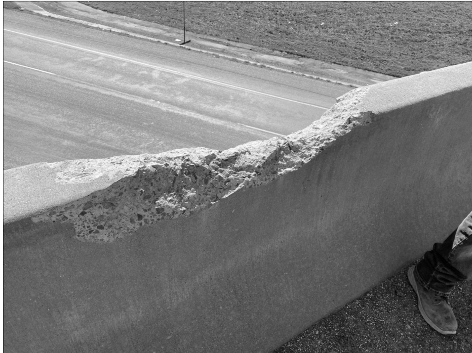
SPALL IN SOUTH BRIDGE RAIL AT SPAN 3
