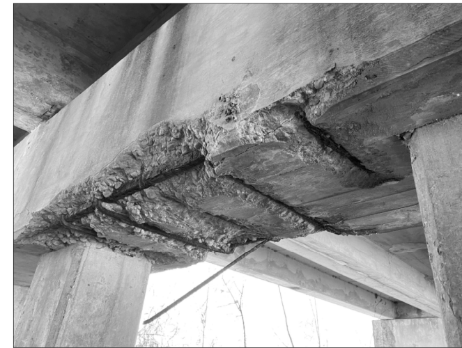
TYPICAL BENT CAP SPALL (SB2)
