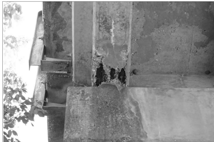
BENT 4 BEAM SPALL (SP1)
