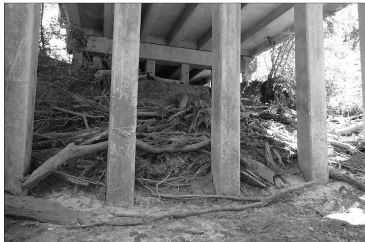
DRIFT AND CHANNEL EROSION AT SPAN 3 (M1 AND M2)
