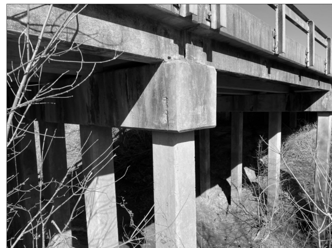
TYPICAL MINOR BENT CAP SPALL (SB1)
