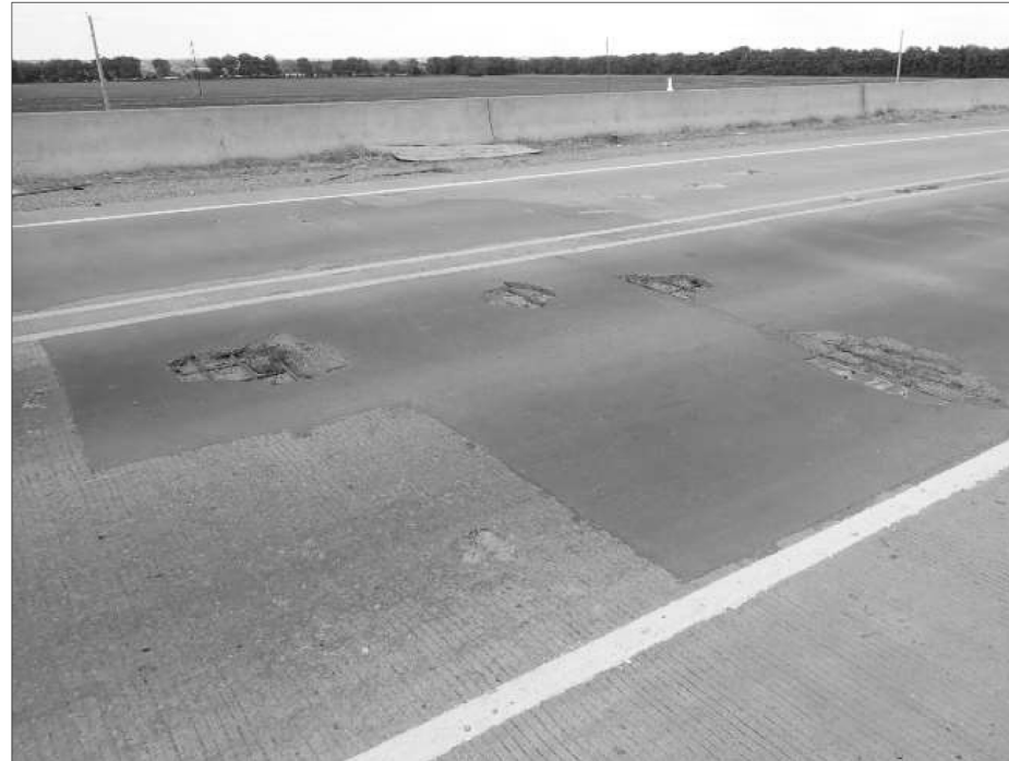
DECK SPALLS WITH EXPOSED REBAR IN SPANS 2 AND 3
