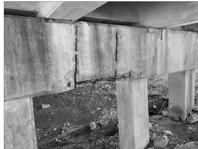
TYPICAL BENT CAP SPALL (SB2)
