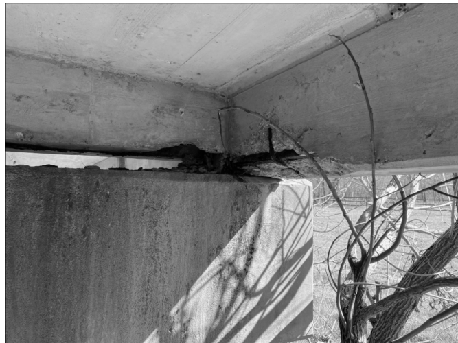
TYPICAL SPALL AT TEE BEAM (SP1)
