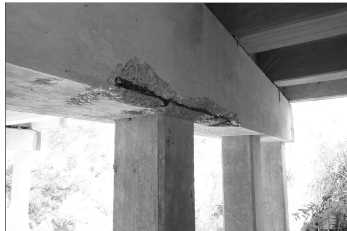
BENT 2 BENT CAP SPALL (SB1)
