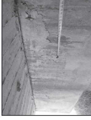
INTERIOR BENT CAP HAS DELAMINATIONS LOOKING NORTHEAST. 18-IN DIAMETER APPROX.
