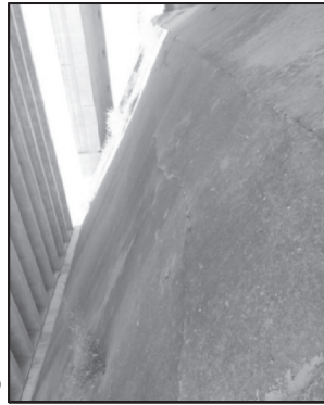
FRACTURE AND BUCKLING OF SOUTH ABUTMENT RIP RAP. 20' APPROX.
