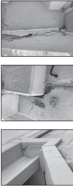
A CRACKS AND SPALLS ON ALL FOUR ABUTMENT BACKWALL AND COPING
