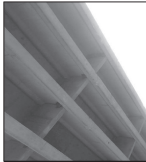
OVERHEIGHT SPALLS TO BEAMS 1-3 IN SPAN 2 LOOKING SOUTHEAST.
