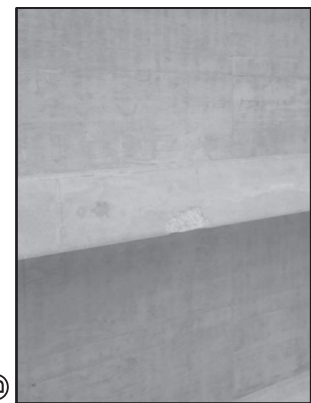
B SPALLS IN BEAMS 3-6 OF SPAN 2 LOOKING SOUTHWEST. 1 SF APPROX.
