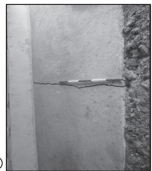
FRACTURE IN ABUTMENT RIPRAP NEAR CENTER LOOKING SOUTH. 8 LF APPROX.
