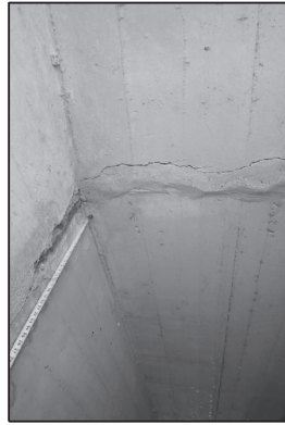
TRANSVERSE AND VERTICAL CRACKING AT WIDENED JOINTS
