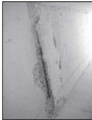
DELAMINATION AND SPALLS WITH EXPOSED REBAR ON BOTTOM OF TOP SLAB IN BARREL 2 FROM NORTH AT EAST END LOOKING NORTHEAST.
