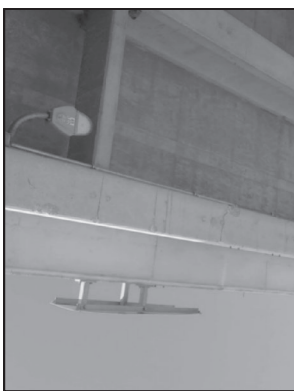
IMPACT SPALLS TO WEST EXTERIOR BEAM OF CENTER SPAN LOOKING NORTH. 1 SF APPROX.
