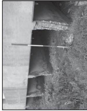
MODERATE SPALLS WITH EXPOSED STEEL AT EAST ENDS OF INTERIOR WALLS #3-5 (FROM NORTH).
