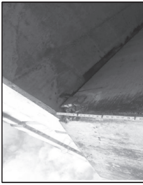
CORNER SPALL AT BENT 3 CAP LOOKING SOUTHWEST.
