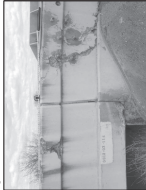
IMPACT DAMAGE TO CONCRETE/ABUTMENT INTERFACE AREA, LOOKING EAST.
