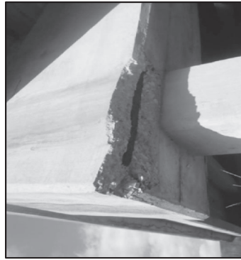
BENT 2 CORNER SPALL AT WEST END OF CAP LOOKING NORTH.
