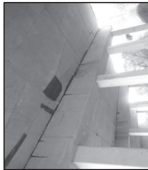
AREAS OF SPALLING AT NORTH FACE OF BENT & CAP LOOKING SOUTHWEST.
