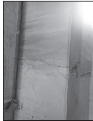
B INTERIOR BENT CAP HAS A VERTICAL CRACK AT CONSTRUCTION JOINT AND EXPOSED REINFORCING IN BENT CAP SOFFIT BETWEEN PILES 2 AND 3 LOOKING EAST.
