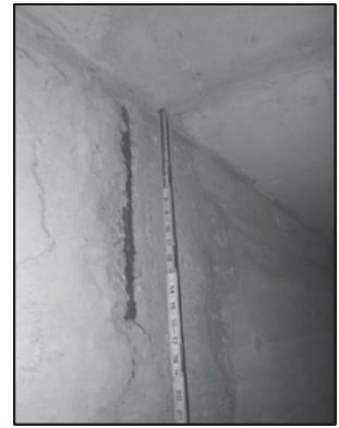
SPALLS WITH EXPOSED REINFORCING IN BOXES 1 - 3 ALONG NORTH WIDENING JOINT LOOKING SOUTH.
