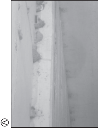
SOFFIT OF ORIGINAL SLAB HAS SPALLING WITH EXPOSED REBAR ALONG SOUTH EDGE LOOKING NORTHEAST. 6 SF APPROX.
