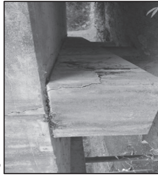
NORTH END OF CAP. 12' X 24" SPALLED AREA APPROX.
