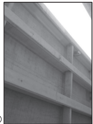
A SPALL IN BEAM 2 OF SPAN 2 LOOKING SOUTH. 1 SF APPROX.
