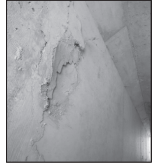
PATCHED AREA WITH DELAMINATION ON BOTTOM OF TOP SLAB IN BARREL 2 FROM WEST LOOKING NORTHEAST.
