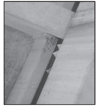
BENT 15 SPAN 14 HAS AN AREA OF DELAMINATION UP TO 2SF WITH CRACKING UP TO 1/32-IN WIDE IN DECK SOFFIT BETWEEN BEAMS 2 AND 3 LOOKING SOUTHWEST.
