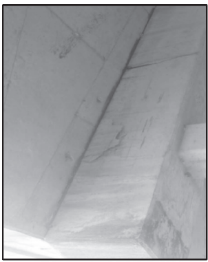
DELAMINATION AT BENT 12 LOOKING SOUTH 4.5' X 4.5' APPROX.
