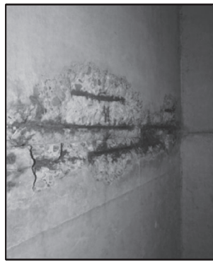
(A) MODERATE SPALL WITH EXPOSED AND CORRODED REBAR IN SOFFIT OF TOP SLAB AT BARREL #5 (FROM NORTH).
