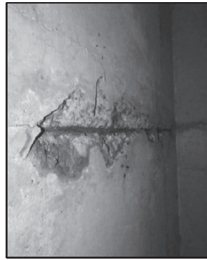
(B) MODERATE SPALL WITH EXPOSED AND CORRODED REBAR IN SOFFIT OF TOP SLAB AT BARREL #1 (FROM NORTH).
