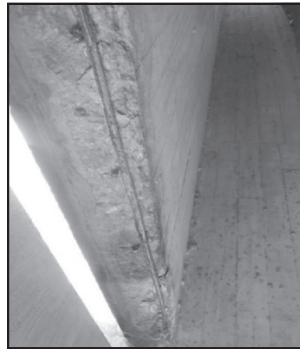
SPALLS WITH EXPOSED REBAR ON BOTTOM OF SLAB UNDER DRAINAGE INLET IN BARREL 5 FROM SW NEAR SE END LOOKING NORTHWEST.
