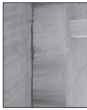
BENT 11 CAP SPALL LOOKING SOUTH: 1.5 SF X 2.5' D APPROX.
