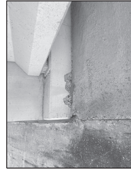
SPALLING ON SOUTH ABUTMENT 0038-01-082
