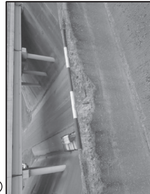
EAST BRIDGE RAIL DAMAGE NEAR BENT 2 SPAN 2 LOOKING EAST.
