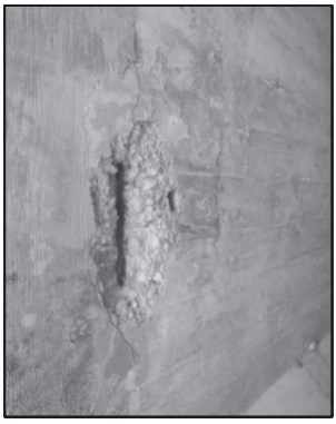
SPALL WITH EXPOSED REBAR AND DELAMINATION ON BOTTOM OF TOP SLAB IN NORTH END OF WEST BARREL LOOKING SOUTH. (1'-3" X 1'-5")
