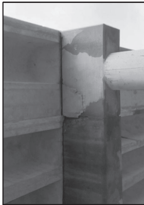
SPALL WITH EXPOSED STEEL NEAR WEST END OF CAP AT BENT 19 (FROM SOUTH) 2' DIAMETER APPROX. 4 SF.
