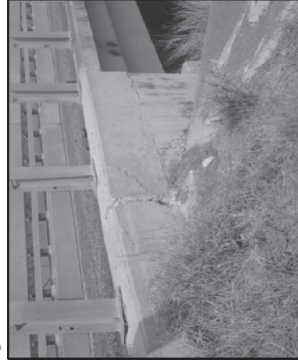
IMPACT DAMAGE TO SOUTHWEST CORNER WINGWALL EXTENSION LOOKING NORTHEAST.
