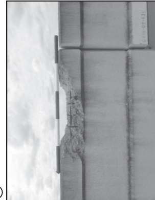
SOUTHEAST APPROACH RAIL DAMAGE LOOKING WEST.
