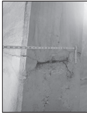
A INTERIOR BENT CAP HAS A VERTICAL CRACK AT CONSTRUCTION JOINT AND A SPILL WITH EXPOSED REINFORCING IN BENT CAP SOFFIT BETWEEN PILES 2 AND 3 LOOKING EAST.
