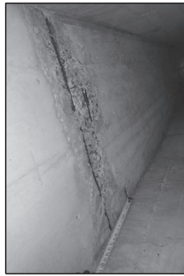
SPALLS WITH EXPOSED CORRODED REINFORCING IN TOP SLAB SHOWN MOST SEVERE ON BARREL 3 FROM SW. CLEAN AND PATCH SPALL.
