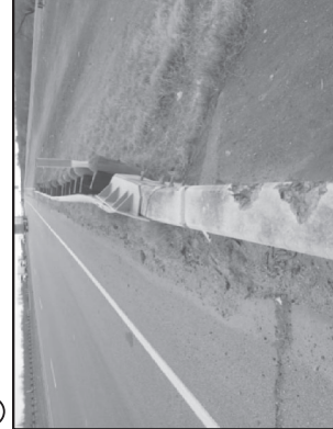
IMPACT DAMAGE TO CONCRETE/ABUTMENT INTERFACE AREA.
