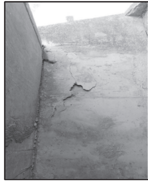
DELMINATION AT NORTH END OF WEST ABUTMENT CAP LOOKING NORTHWEST. 20\"/>
