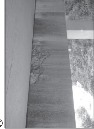
Ⓐ BENT 3 CAP HAS A SPALL OVER PILE 2 LOOKING NORTH. 32"W X 16"H X 2'D APPROX.
