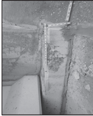
SPALL AT EAST END OF NORTH ABUTMENT CAP LOOKING NORTH.
