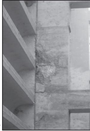
SPALL WITH EXPOSED REBAR ON BENT CAP 4 WEST FACE LOOKING EAST. 4 SF APPROX.
