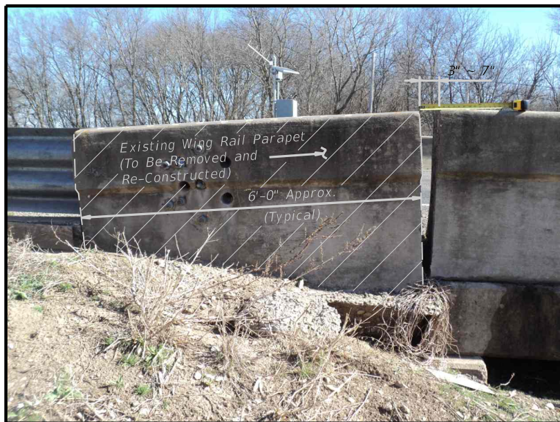
ELEVATION OF EXISTING SETTLED RAIL PARAPET (SHOWING SW CORNER - STR #028 ASH CREEK) OTHER LOCATIONS ~ SIMILAR
