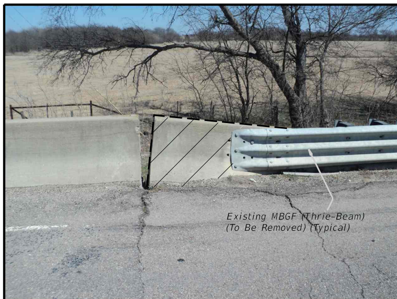
ELEVATION OF EXISTING SETTLED RAIL PARAPET (SHOWING THRIE-BEAM CONNECTION) TYPICAL FOR ALL LOCATIONS
