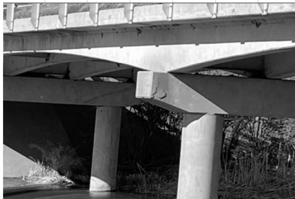
BENT 3 COLUMN 2 CONC STR REPR 10 SF
