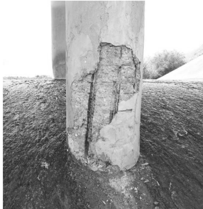
Bent 4 Column 2 CONC STR REPR 80 SF
