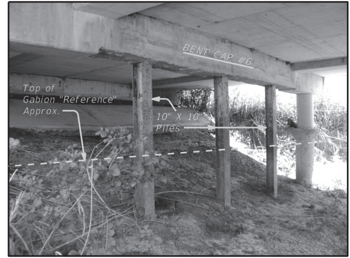
EROSION REPAIR AT INTERIOR BENT #6 (SHOWING APPROX. LIMITS OF GABION WALL) (LOOKING NE)
