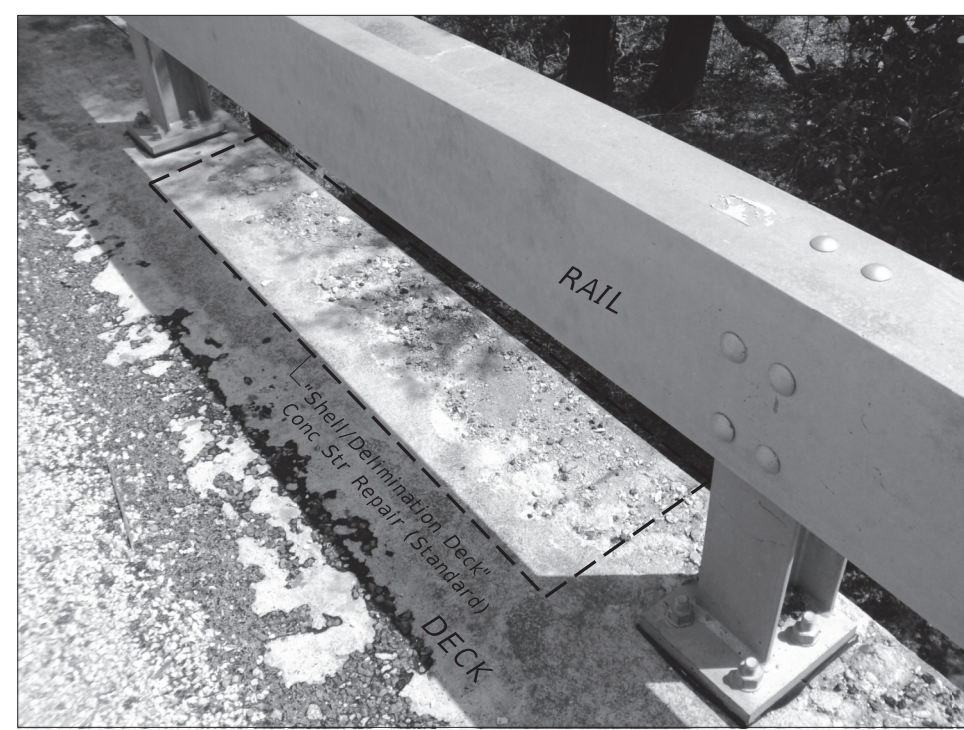
SCALING CONCRETE DECK REPAIR DETAILS SHOWING LIMITS OF SCALING REPAIR AT DECK EDGE
