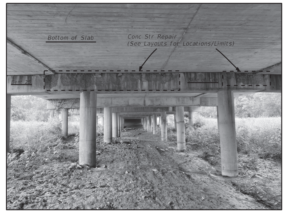
CONCRETE STRUCTURE REPAIR △ SHOWING SPALLS AT SIDE OF CAP
