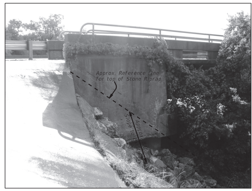
RIPRAP REPAIR AT ABUTMENT #5 WINGWALL (SHOWING LIMITS OF STONE PROTECTION) (LOOKING EAST)
