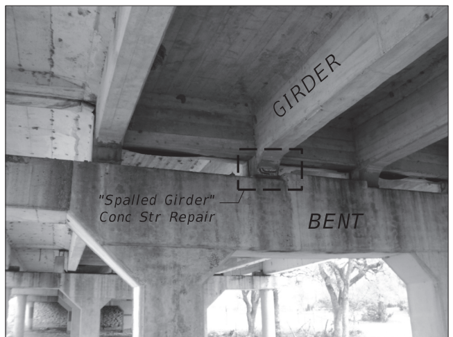
① SPALL REPAIR AT GIRDER (SEE LAYOUT FOR SPALL LOCATION)
