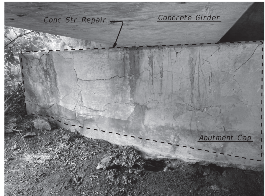
CONCRETE STRUCTURE REPAIR △ SHOWING SPALL ALONG ABUTMENT CAP
