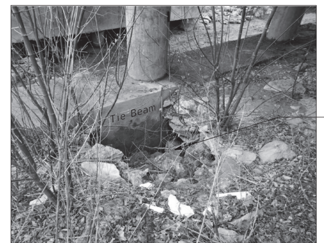
① REPAIR AT EXISTING TIE BEAM SHOWING LIMITS OF REPAIR AREA BENT #4 SOUTH SIDE DETAIL 1
