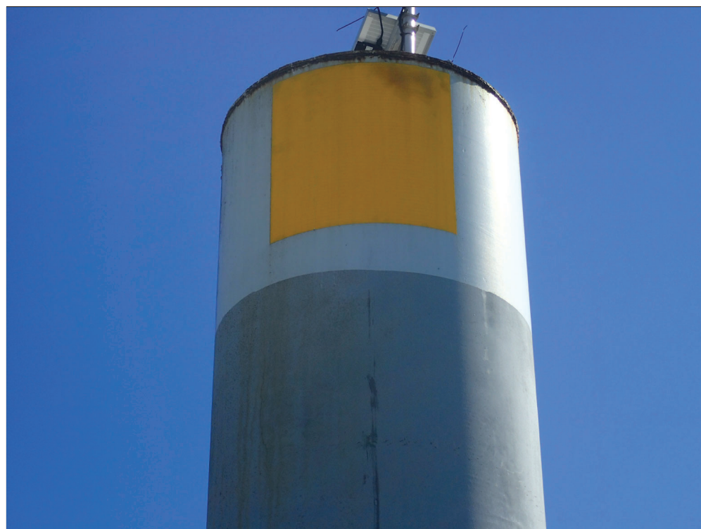
RETRO-REFLECTIVE ADHESIVE SIGN ON INTERMEDIATE DOLPHIN (SQUARE)
