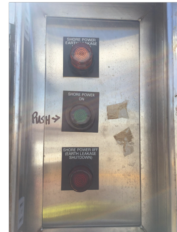
SHORE POWER CABINET CONTROLS FRONT EXTERIOR VIEW
