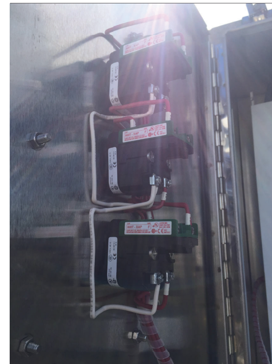
SHORE POWER CABINET CONTROLS FRONT INTERIOR VIEW
