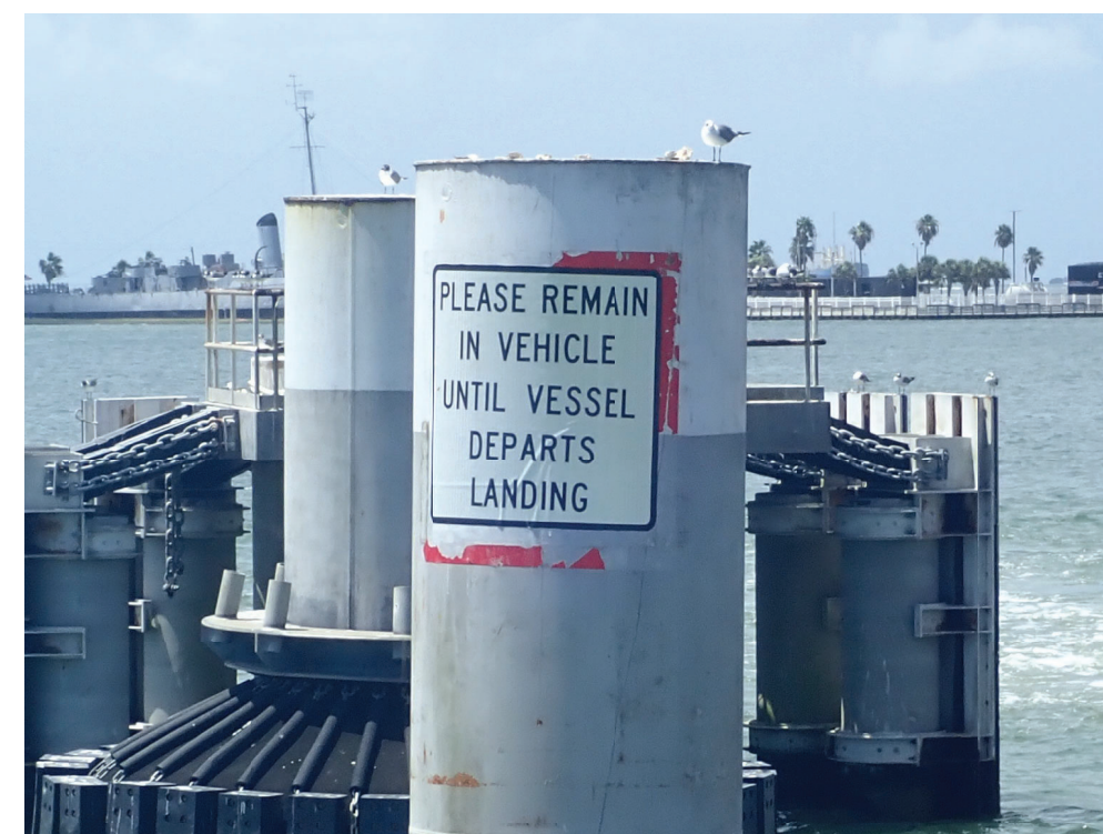
NOTICE TO MOTORISTS ADHESIVE SIGN ON MONOPILE DOLPHIN
