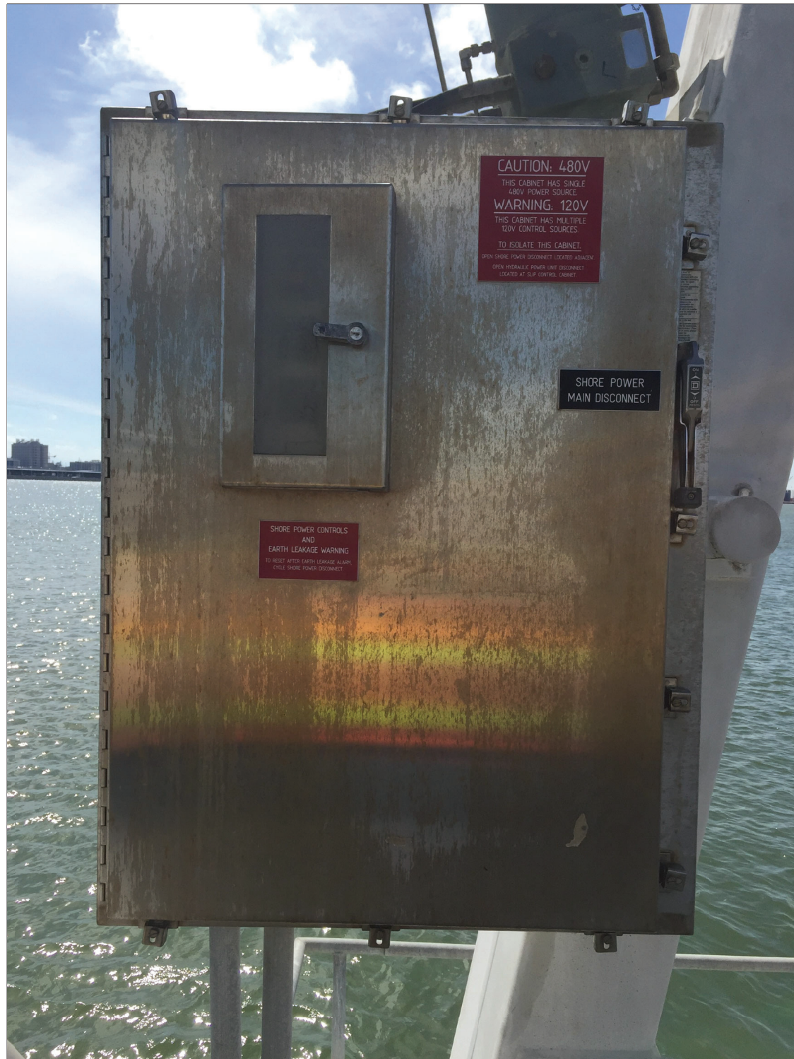
SHORE POWER CABINET FRONT EXTERIOR VIEW
