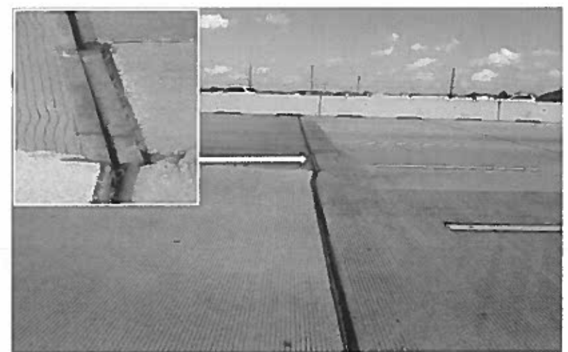
③ REPLACE DAMAGED BRIDGE JOINT (SEJ) EASTBOUND MAINLANES BETWEEN MANAGED LANES AND WIDENING SECTION.
