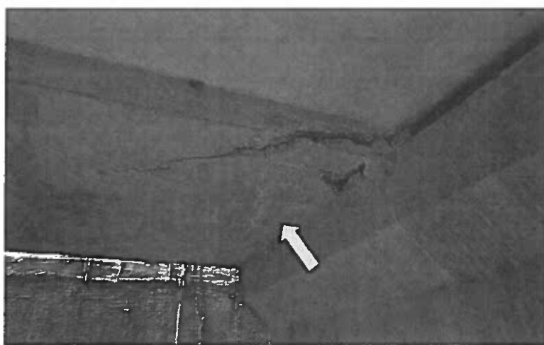
④ DELAMINATION IN THE DECK SOFFIT LEFT OF BEAM 3.
