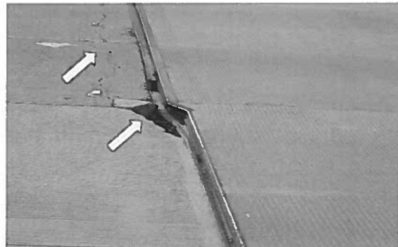
③ REPLACE DAMAGED BRIDGE JOINT (SEJ) WESTBOUND MAINLANES BETWEEN MANAGED LANES AND WIDENING SECTION.
