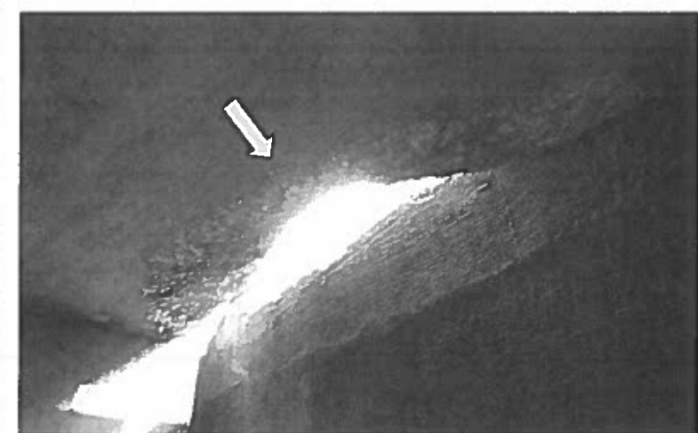
⑤ DEEP SPALL WITH EXPOSED REBAR IN DECK SOFFIT ALONG BEAM 1.
