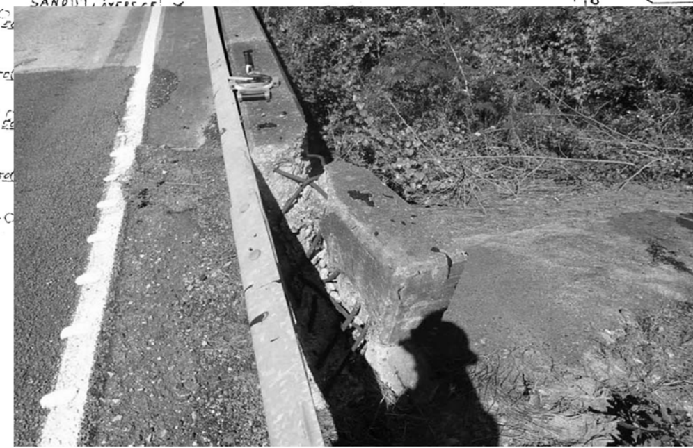
IMPACT DAMAGE TO RAIL AT SOUTH CORNER
