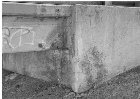
B Typical Abutment Cracks
