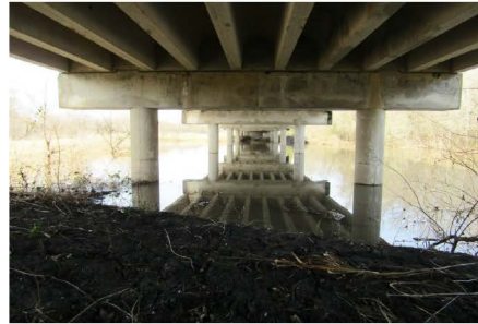
CONTRACTION SCOUR BETWEEN BENTS 7-11. HIGH WATER LEVEL HIDES EXPOSED DRILLED SHAFTS LOOKING NORTHEAST
