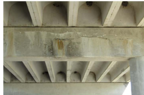
SOUTHWEST FACE OF CENTER BENT HAS DELAMINATION & CRACKING LOOKING NORTH
