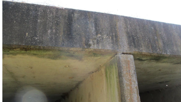
7 - Crack in concrete on west side at top of wall
