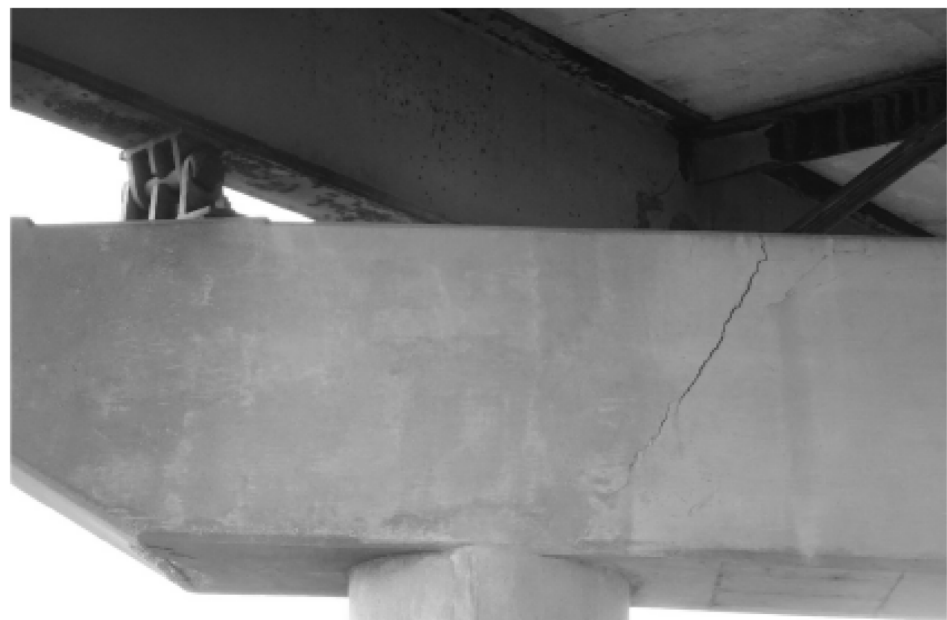
NOTE: 1. The North interior bent cap has a wide diagonal shear crack (approx. 1/4") over the inside face of the East column.
