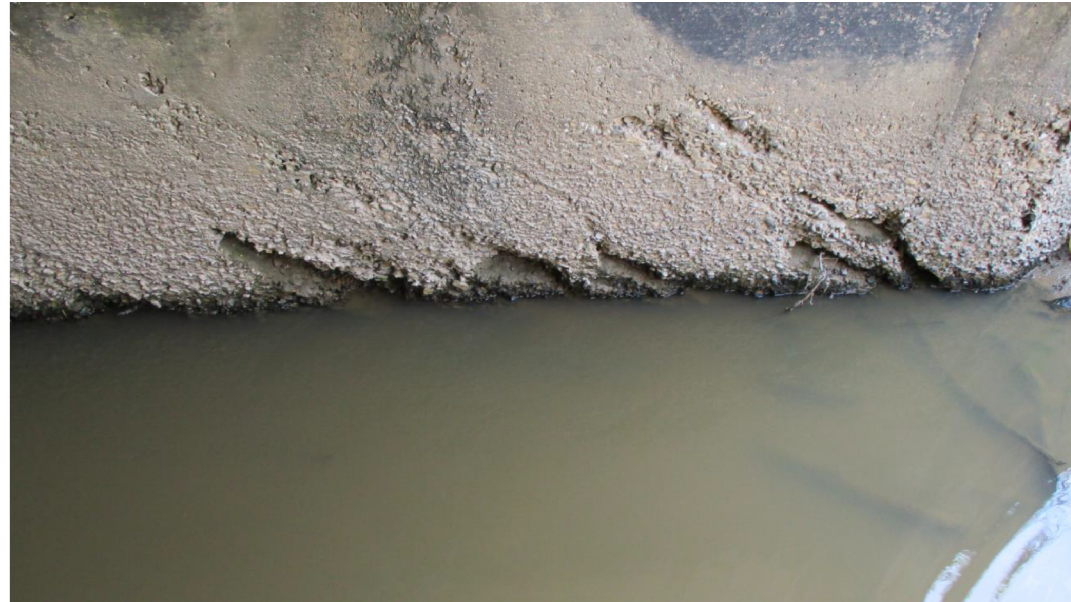
11 - Voids and deterioration in bottom of walls
