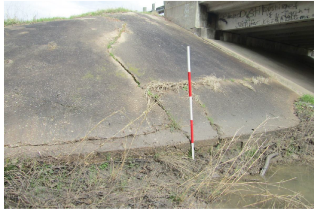
NORTHWEST CORNER OF RIPRAP AT UPSTREAM SIDE HAS MODERATE SCOUR LOOKING NORTHEAST
