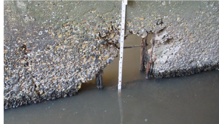
9 - Voids at lower section of interior culvert walls
