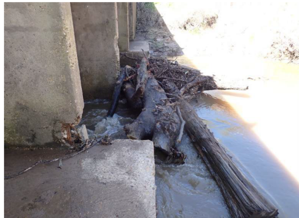
Moderate drift accumulation at upstream and downstream end of culvert
