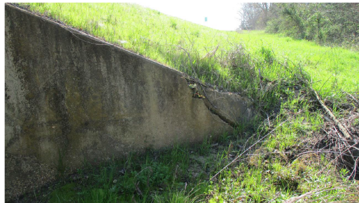
8 - Cracked/Spalled concrete in wingwall
