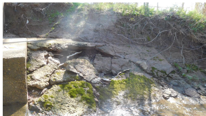
8 - Partial collapse of riprap
