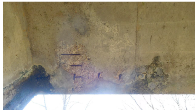
9 - Spalling concrete in top of barrels, exposed rebar
