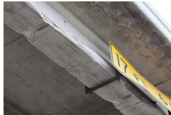
SEVERAL IMPACT SPALLS WITH STRANDS EXPOSED ALONG EAST BEAM AT SPAN 5 LOOKING NORTHWEST
