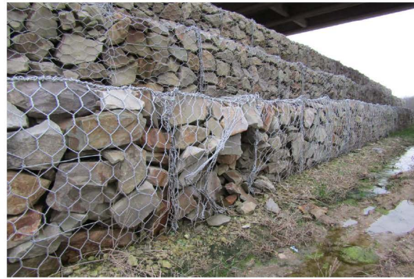
IMPACT DAMAGE TO SOUTH ABUTMENT GABIONS LOOKING SOUTHWEST
