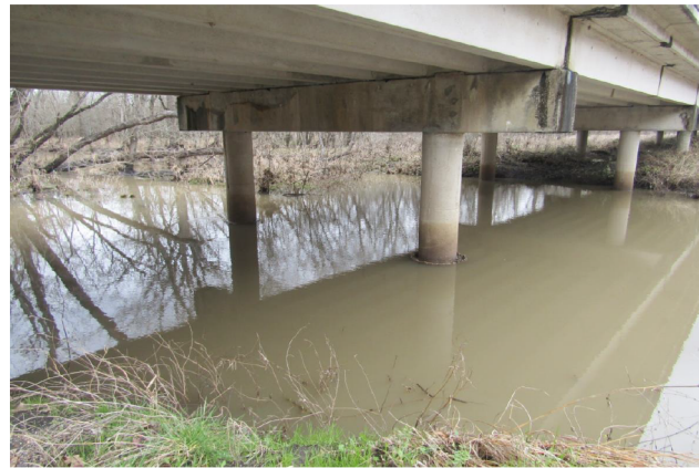
MODERATE CONTRACTION SCOUR AT BENTS 12 & 13 HAVE EXPOSED DRILLED SHAFTS LOOKING NORTHWEST
