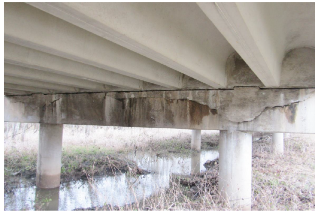
MODERATE DELAMINATION AND SPALLING ALONG SOUTH FACE OF CAP 9 LOOKING NORTHWEST
