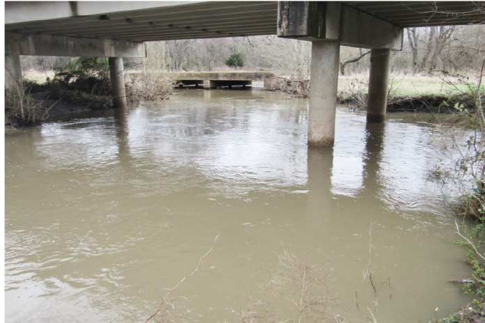
EXPOSED DRILLED SHAFTS AT BENT 8 ARE BELOW WATER LOOKING NORTHEAST
