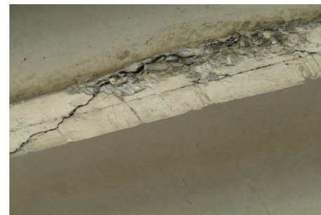
DELAMINATING OF STEM 4 FROM SOUTHEAST ALONG SPAN 3 LOOKING EAST
