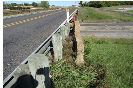
WEST WINGWALL IS LEANING AWAY FROM BRIDGE LOOKING NORTH
