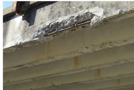
SOUTHEAST EXTERIOR GIRDER STEM OF SPAN 3 HAS SEVERE IMPACT DAMAGE WITH EXPOSED REBAR LOOKING WEST
