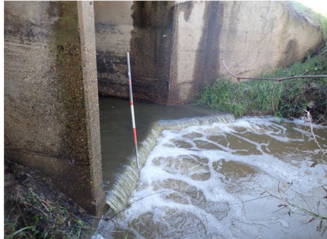
Channel scour has exposed culvert toewall at Southeast Barrel (~1' high) at upstream end and (~3.5' high) with slight undermining (< 1' deep) at downstream end
