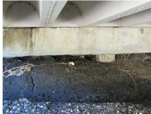
UNDERMINING OF SOUTHEAST ABUTMENT AND EXPOSED PILES LOOKING SOUTHEAST
