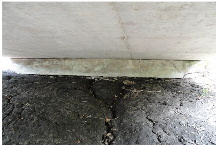
UNDERMINING OF EAST ABUMENT CAP AND EXPOSED PILES LOOKING EAST
