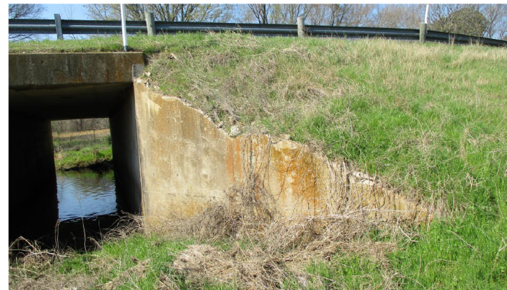
10 - Cracked/Spalled concrete in wingwall
