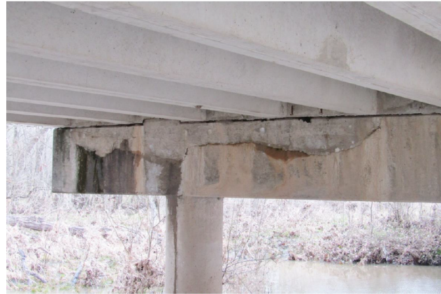
MODERATE DELAMINATION AND SPALLING ALONG SOUTH FACE OF CAP 13 AT WEST END LOOKING NORTHWEST
