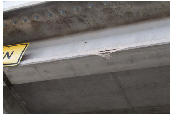
MINOR IMPACT SPALL WITH TWO STRANDS EXPOSED ON WEST BEAM AT SPAN 5 LOOKING NORTHEAST
