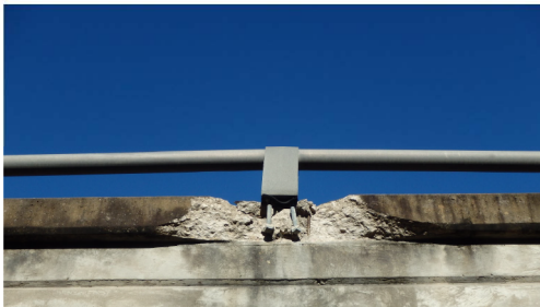
SPALL WITH EXPOSED ANCHOR BOLTS AT SOUTHEAST BRIDGE RAIL (TYP) LOOKING NORTHWEST
