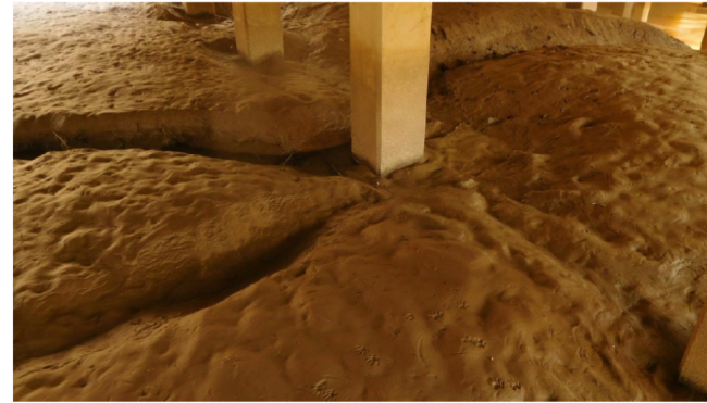
9 - Undermining of piles
