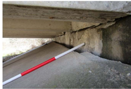
NORTHWEST RIRAP HAS MOVED (4") FROM THE ABUTMENT CAP LOOKING SOUTHEAST
