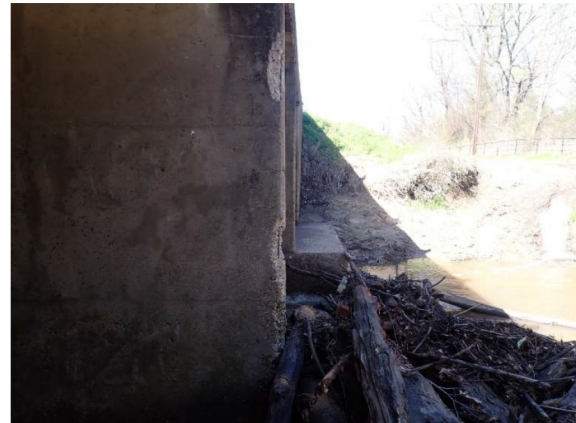
Upstream end of culvert walls in center barrels have significant spalling (~5'H x 2'D)
