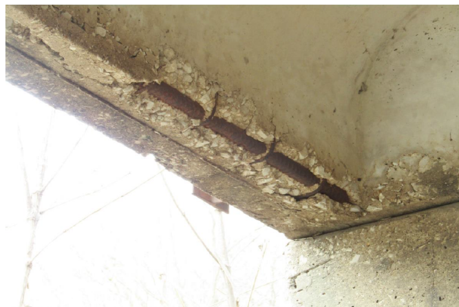
MODERATE DELAMINATION AND SPALLING WITH EXPOSED REBAR OF WEST EXTERIOR BEAM OVER BENT 2 LOOKING NORTHWEST
