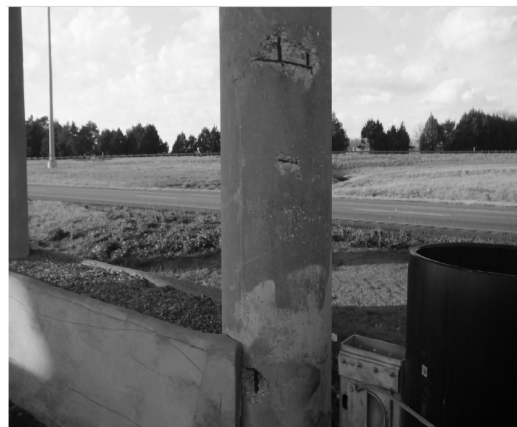
NOTE: 1. The East exterior column at the center bent has approximately 12 sq. ft. of delaminations and approximately 3 sq. ft. of spalls that are 2" deep with exposed rebar.
