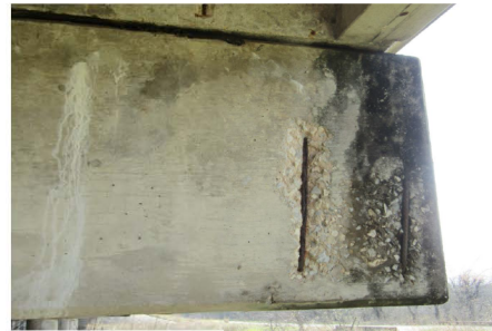
UPSTREAM END OF BENT CAP 5 HAS MODERATE SPALLS WITH EXPOSED REBAR LOOKING WEST
