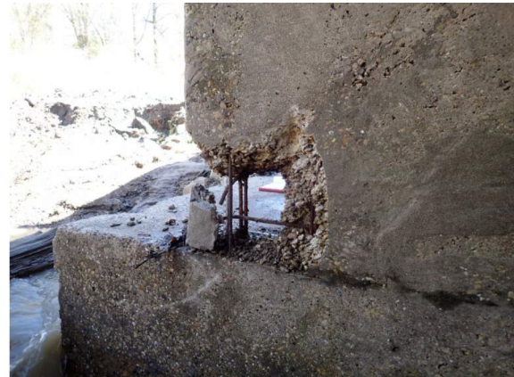
Upstream end of culvert walls in center barrels have significant voids (up to 2 SF x full width)
