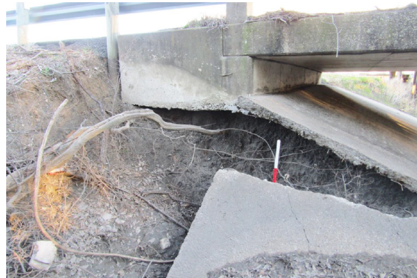
RIPRAP SLAB, ABUTMENT CAP AND WINGWALL ARE UNDERMINED AS MUCH AS 4' BACK DUE TO RIPRAP FAILURE LOOKING SOUTHEAST
