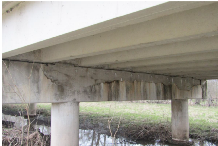
MOST ALL OF NORTH SIDE OF CAP 3 HAS MODERATE DELAMINATIONS & SPALLING LOOKING SOUTHWEST
