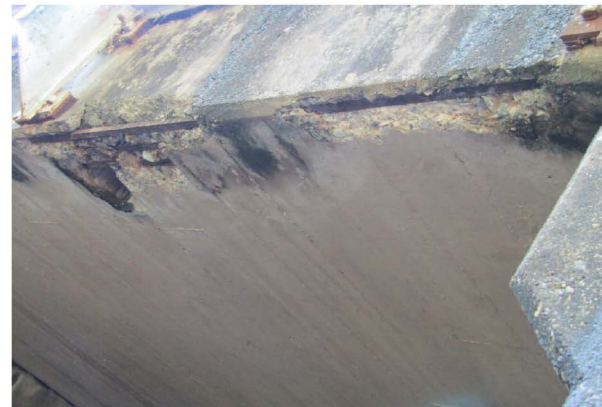
SPALLING WITH EXPOSED REBAR AT SPAN 2 FROM SOUTHWEST ALONG SOUTHEAST SIDE LOOKING WEST
