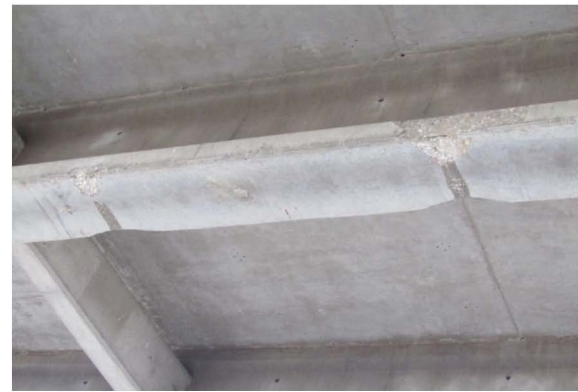
IMPACT SPALLING WITH STRANDS EXPOSED ALONG BEAM 3 FROM WEST IN SPAN 5 FROM THE NORTH LOOKING NORTHEAST
