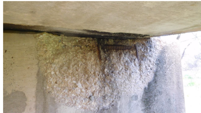
8 - Spalling concrete with exposed rebar on bent cap
