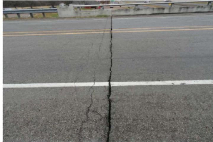
THE NORTH ABUTMENT JOINT HAS CRACKS LOOKING EAST
