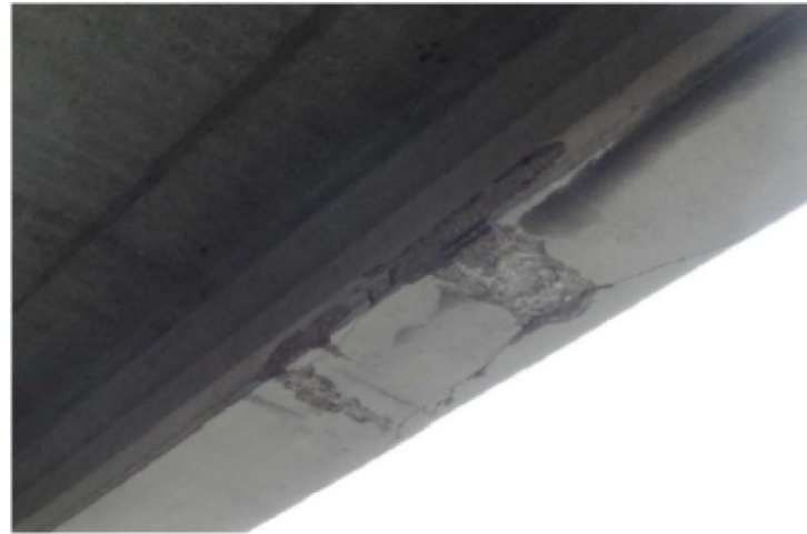
MODERATE SPALL WITH EXPOSED REBAR ALONG WEST EXTERIOR BEAM AT SPAN 3 LOOKING SOUTHWEST
