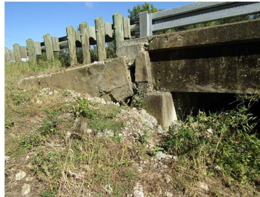
BROKEN AND SEPARATED WEST WINGWALL LOOKING NORTH
