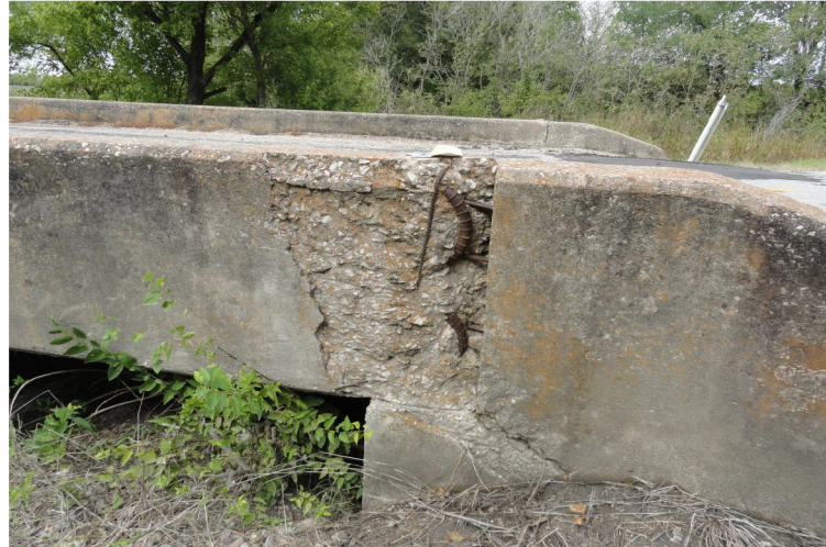
SPALLS AT EAST END OF SOUTH PARAPET LOOKING NORTH
