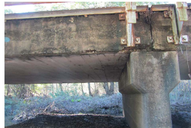
MINOR SPALLING WITH EXPOSED REBAR AT SPAN 3 SOUTHEAST SIDE LOOKING NORTHWEST
