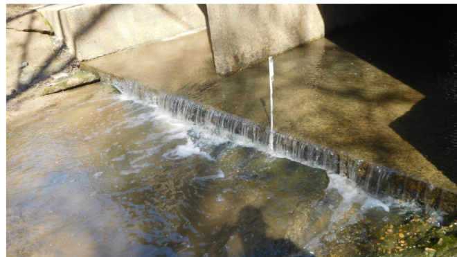
7 - 2 ft scour at downstream toe
