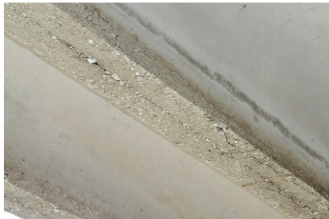
2ND BEAM FROM WEST AT CENTER SPAN HAS HORIZONTAL CRACKING LOOKING NORTHWEST
