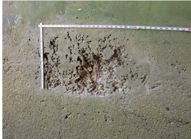
Moderate abrasion, scaling and pitting along bottom of culvert walls with a few minor to moderate voids (up to 2 SF x 2" D) with exposed and corroded rebar.
