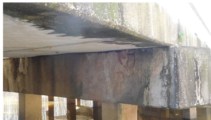
8 - Spalling concrete with exposed rebar on bent caps
