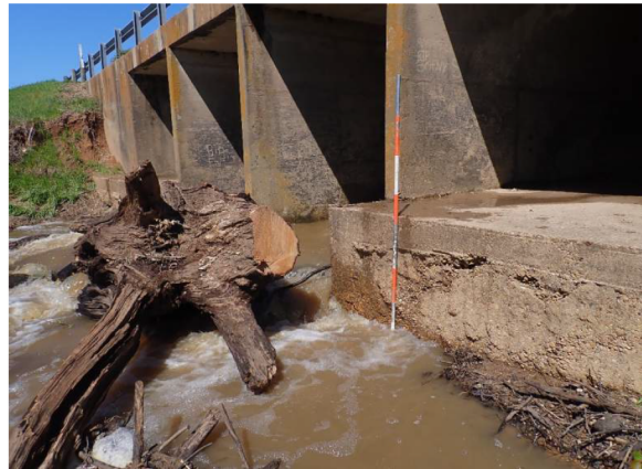
Rock riprap has been placed in upstream and downstream channels and has mostly washed away at downstream end of exterior barrels, leaving exposed toewalls (up to 4.5'H)
