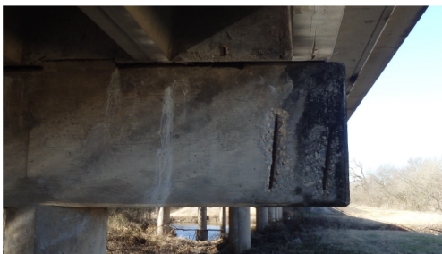
SPALLS WITH EXPOSED REBAR ON BENT CAP 5 (TYP AT OTHER BENT CAPS) LOOKING SOUTHWEST
