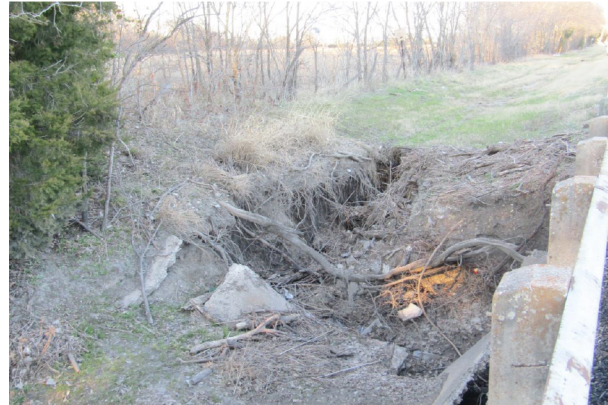
MODERATE EROSION AT THE NORTH DITCH HAS UNDERMINED THE RIPRAP, ABUTMENT CAP AND WINGWALL LOOKING NORTH
