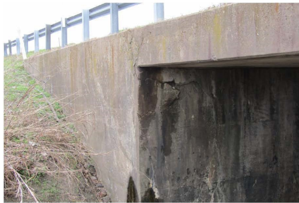
CRACK AND SPALL AT NORTHEAST END OF SOUTHEAST ABUTMENT AND EAST WINGWALL AND HEADWALL INTERFACE. LOOKING SOUTH
