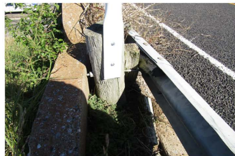
BROKEN BLOCK OUT AT WEST CORNER TRANSITION LOOKING EAST
