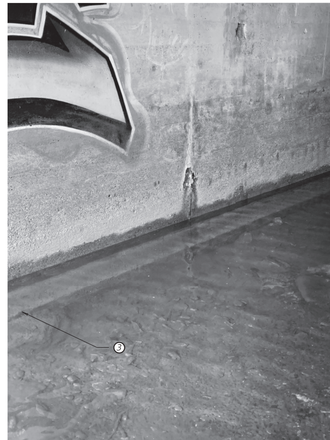
Exposed AB footing, South wall, near East bridge end
