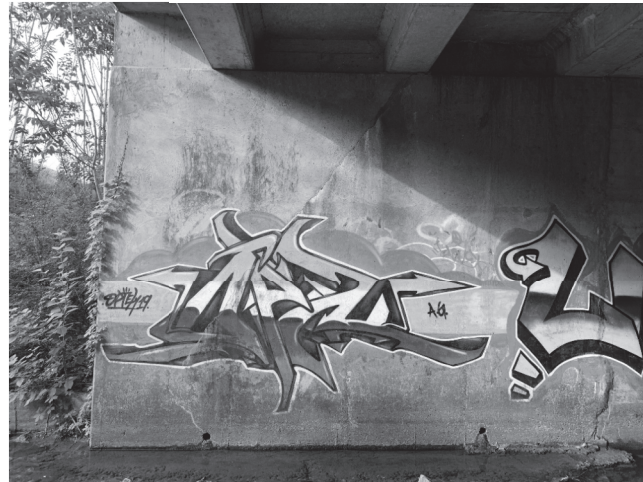
SB1 - Diagonal crack on S AB Wall
