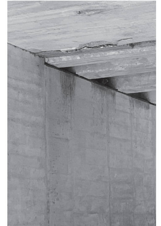
SP3 - Spall/delamination at W widening jt
