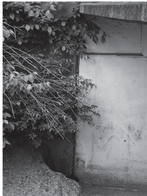
M1 - Gap between NW Retaining Wall and AB wall
