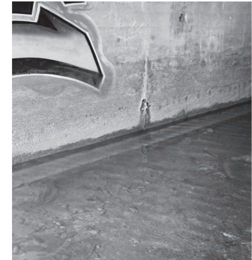
SB3 - Vertical crack at weep hole
