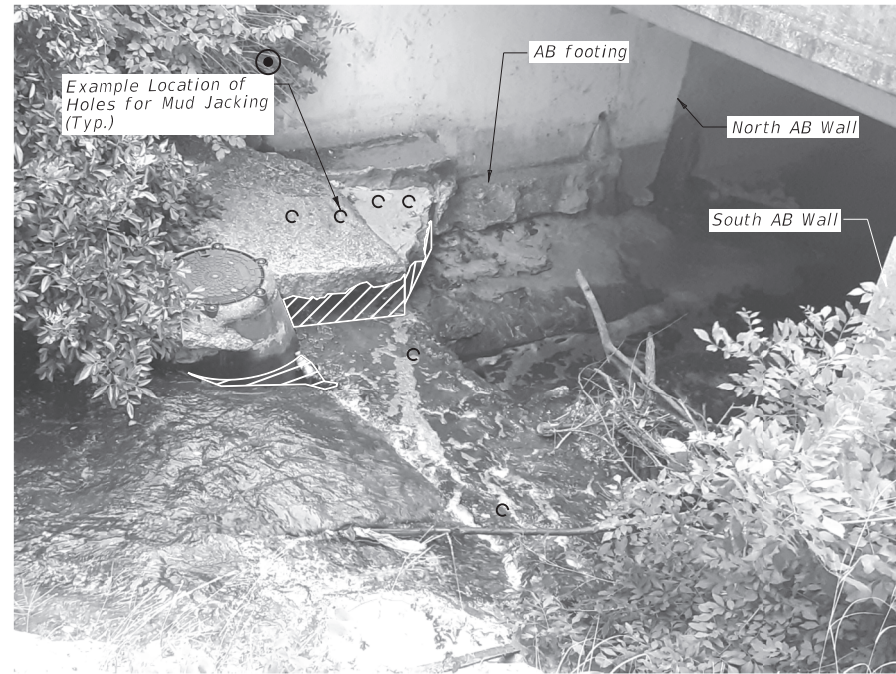
Channel Erosion, facing North, looking downstream
