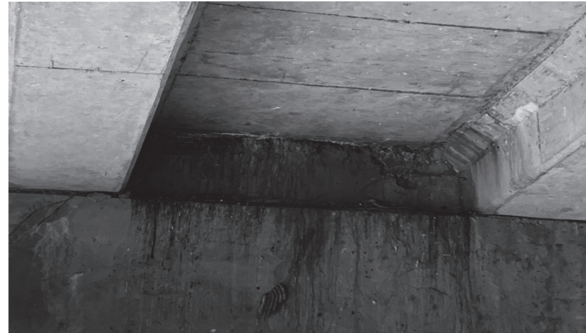
SP1 - Spall on diaphragm at S AB wall
