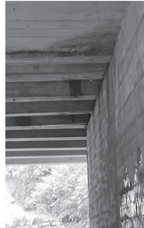
SP1, SP3 - Spall on E face of T-beam, delamination at W widening jt.
