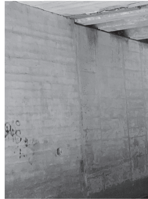
SB2 - Vertical crack at W widening jt, S AB Wall
