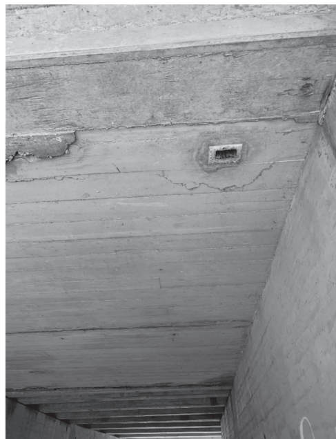
SP3 - Spall/delamination at E widening jt
