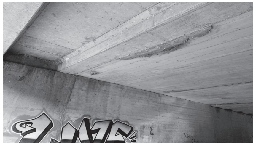
SP3 - Spall/delamination at E widening jt
