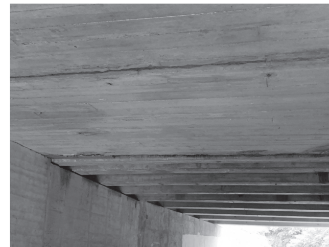
SP4 - Cracking at center widening jt
