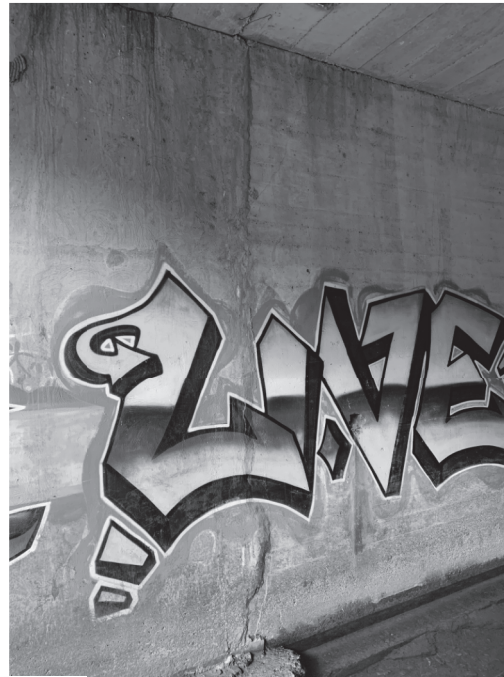
SB2 - Vertical Crack at E widening jt, S AB Wall
