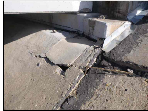
TYPICAL RIPRAP DAMAGE AT ABUTMENT (Showing Abutment 1 SE face from IH 40 WB Overpass at IH 40H FR Conn)
