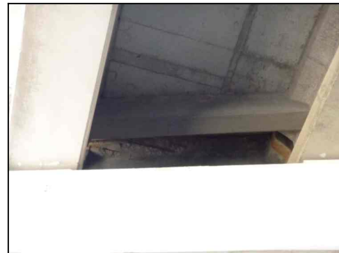
TYPICAL DAMAGE IN DECK SOFFIT AT ARMOR JOINTS AT INTERIOR BENTS
