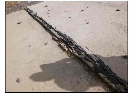
TYPICAL RIPRAP CURB DAMAGE (Showing riprap curb at Abutment 1 from IH 40 WB Overpass at FM 295)
