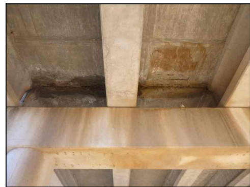
TYPICAL DAMAGE IN DECK SOFFIT AT JOINTS AT INTERIOR BENTS (Showing Joint 2 from IH 40 WB Overpass at BI 40F)
