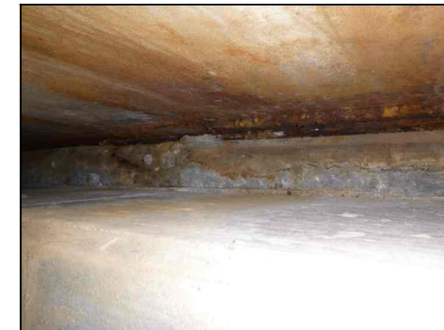
TYPICAL DAMAGE IN DECK SOFFIT AT ARMOR JOINTS AT ABUTMENTS
