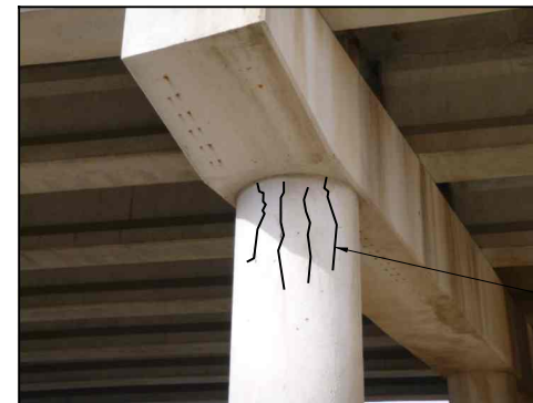
TYPICAL COLUMN SPLIT CRACKING (Showing Bent 3 Column 3 from IH 40 WB Overpass at FM 295)
