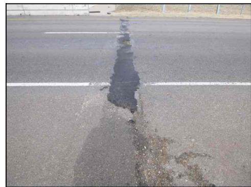
TYPICAL DAMAGE IN ASPHALT PAVEMENT ABOVE RELIEF JOINTS AT APPROACH SLABS
