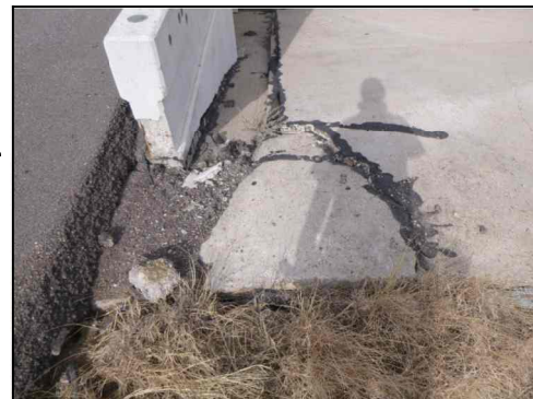
TYPICAL RIPRAP DAMAGE AT WINGWALL (Showing Abutment 4 NE face from IH 40 EB Overpass at IH 40F FR Conn)
