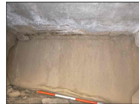
TYPICAL DAMAGE IN DECK SOFFIT AT JOINTS AT ABUTMENTS (Showing Joint 1 from IH 40 WB Overpass at FM 295)
