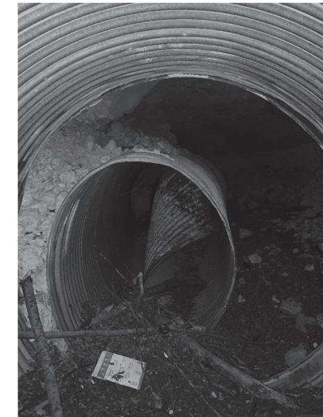
PHOTO OF COLLAPSED CMP IN VOID AREA
