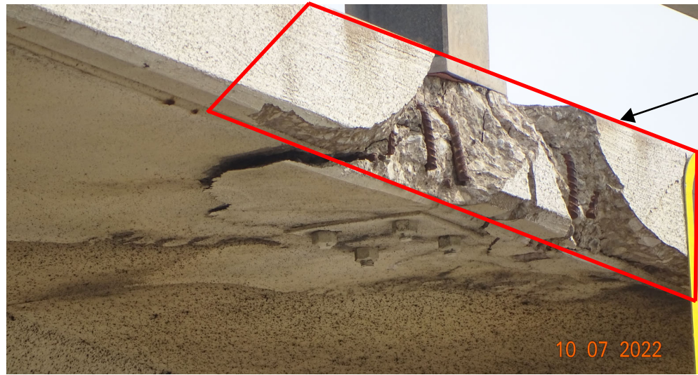
PHOTO 1 (Showing impact damage to overhang soffit in span #3 on the south overhang.)
