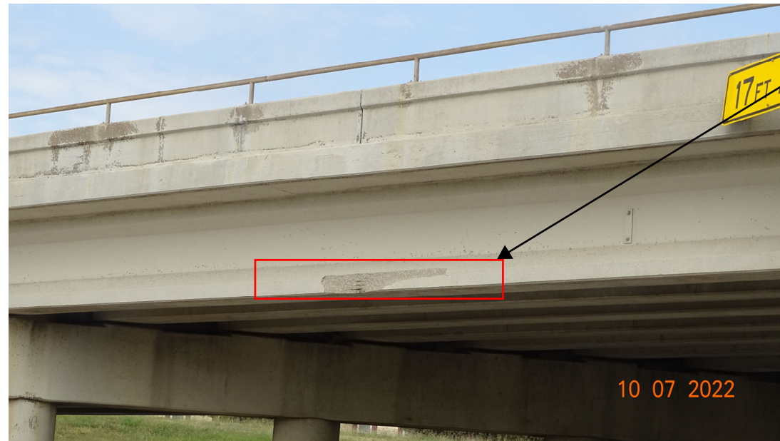
PHOTO 1-A (Showing beam damage at span 3)
