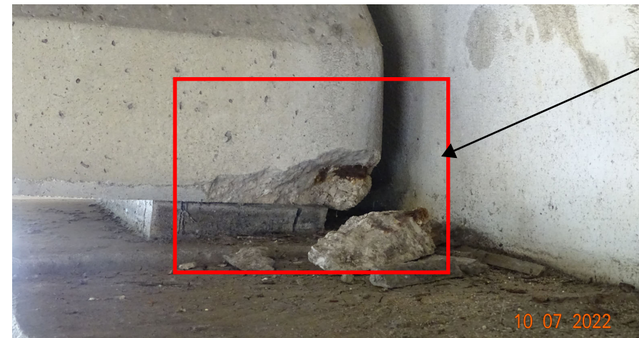
PHOTO 4 (Showing spalling of beam #5 with exposed strand.)
