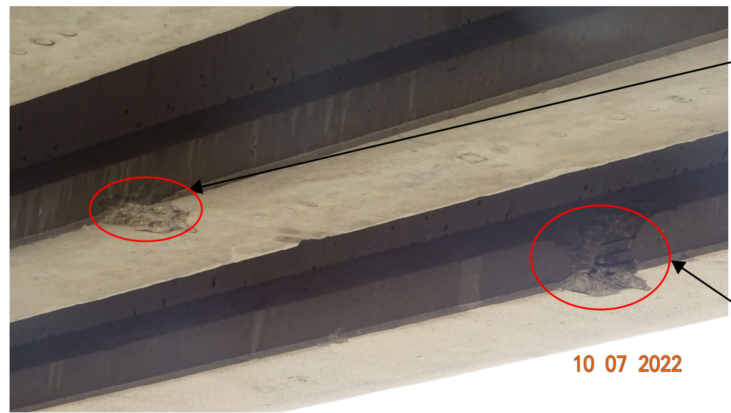
PHOTO 2-A (Showing beam damage at span 2)
