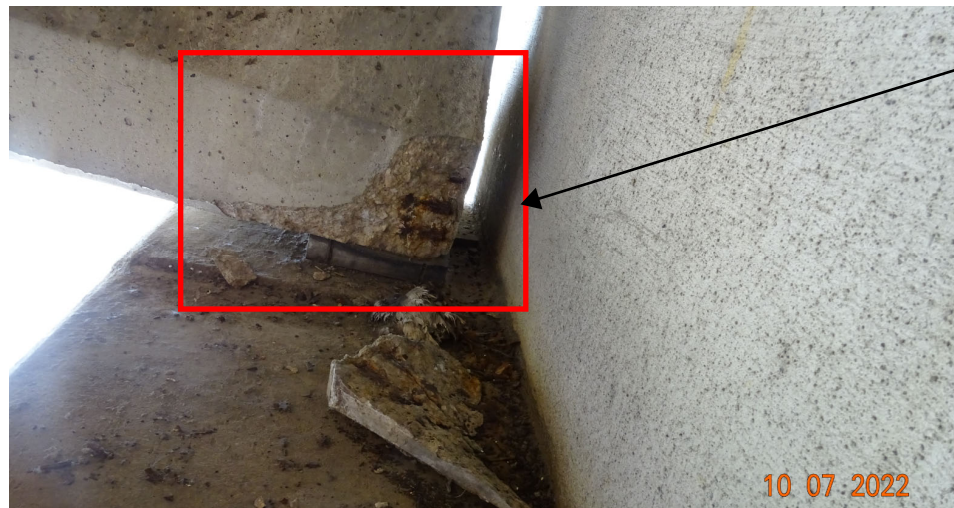
Photo 3 (Showing spalling of beam #6 with exposed strand.)
