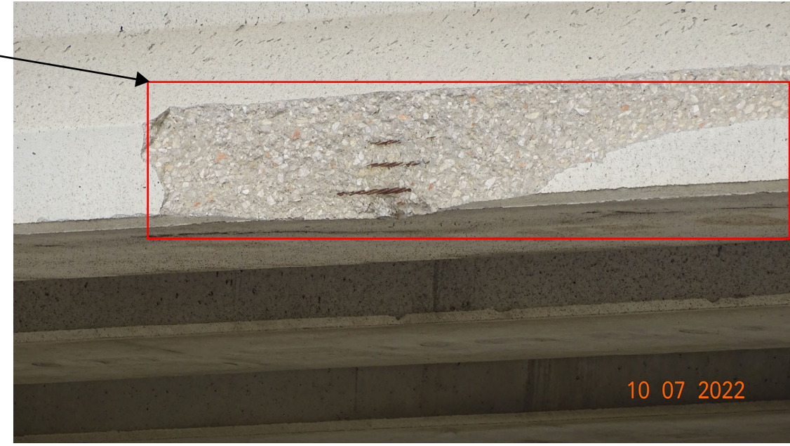
PHOTO 1-B (Showing beam damage at span 3)
