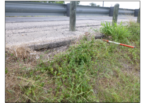
④ UNDERMINING AT SOUTH CORNER MOWSTRIP
