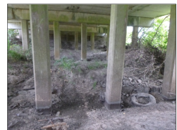
⑤ EROSION CHANNEL AT BENT 3
