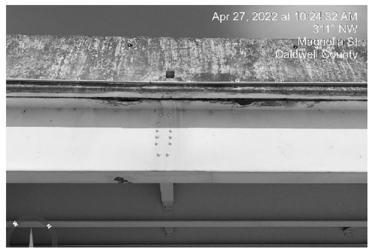
EXISTING DRAIN HOLE
