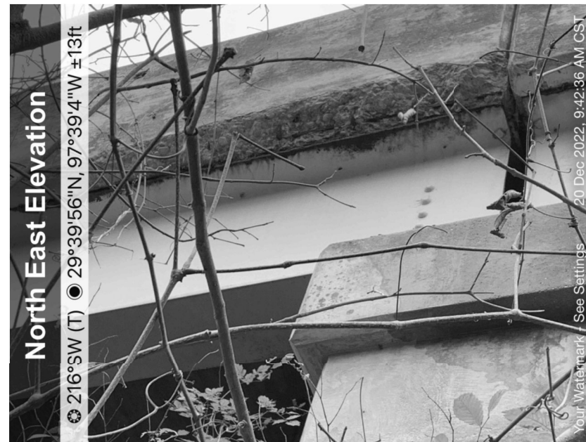
Deck Edge Spall (Typical)
