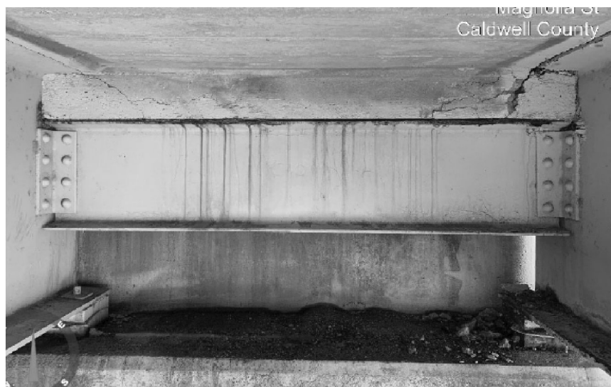
Corrosion on Diaphragm (Typical)
