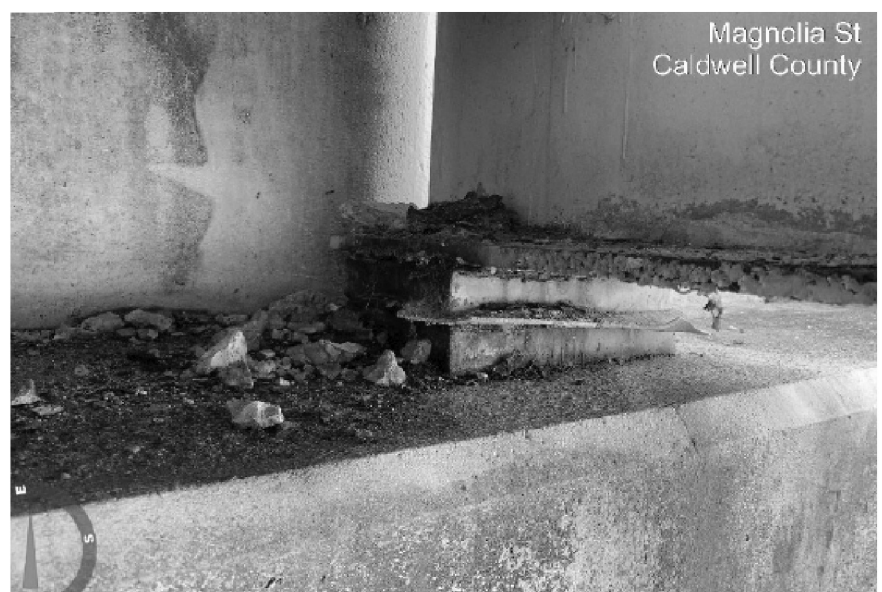
Corrosion on Bearings (Typical)
