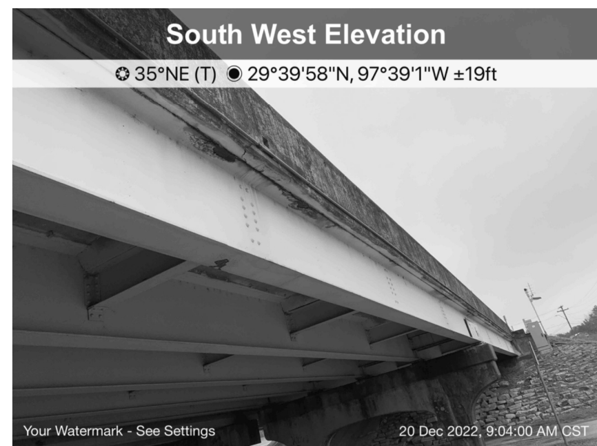
Corrosion on Exterior Beams (Typical)
