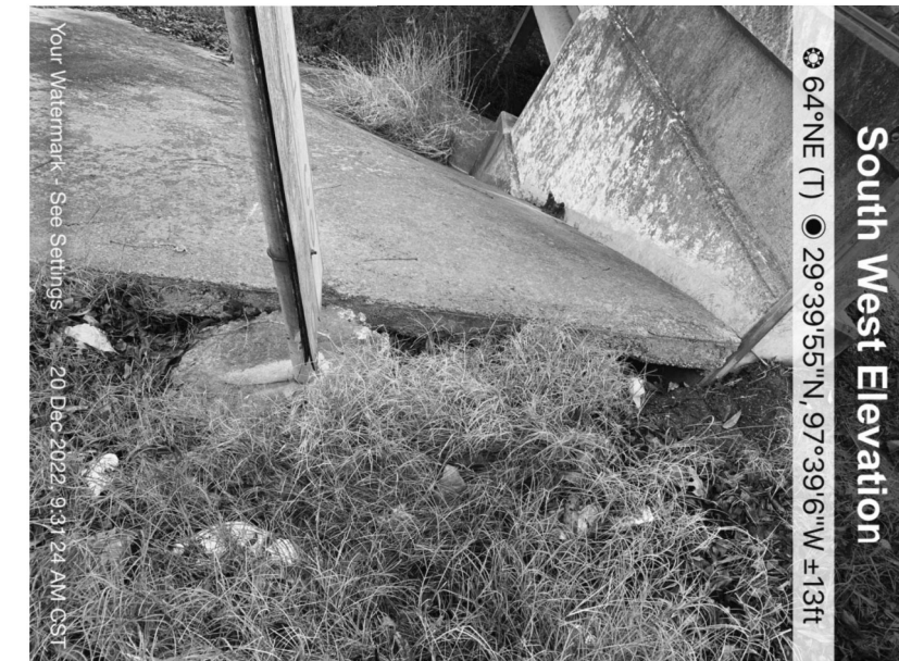
Undermining at SW Riprap
