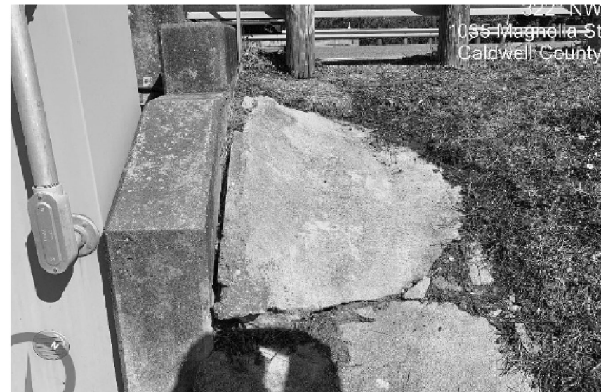
Broken Shoulder Drain
