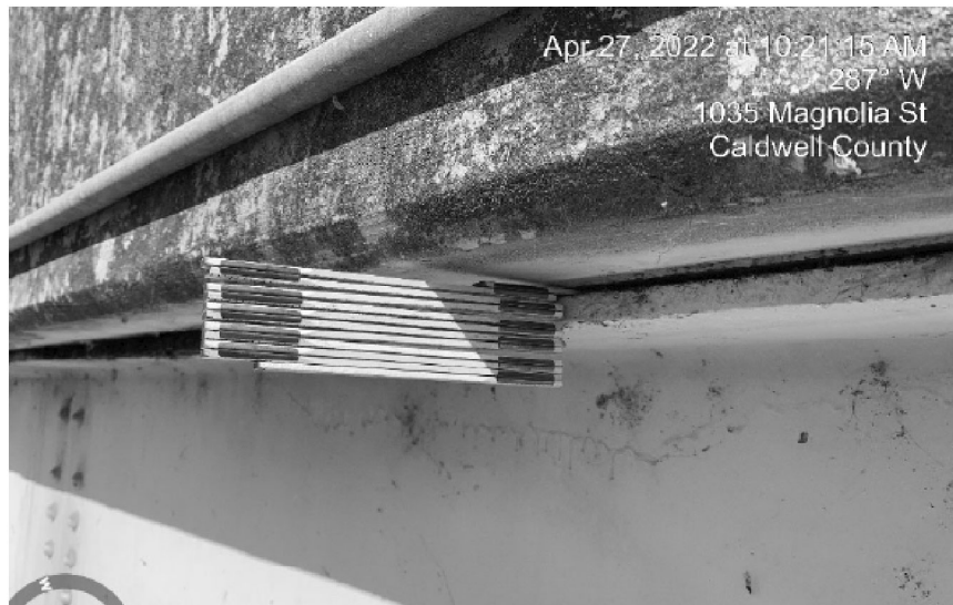
Top Flange separated from Deck
