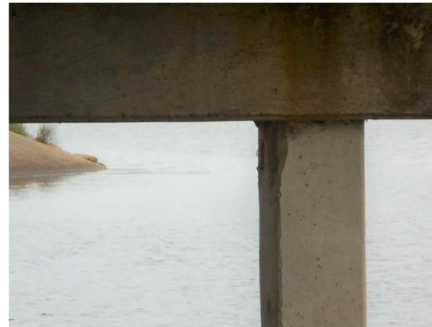
Spall on West pile of Bent 2 from North SB1 1 SF
