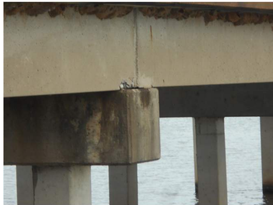
Typical Superstructure spall at both ends of Bents 2 and 3 from North SP1 1 SF Each at 4 locations
