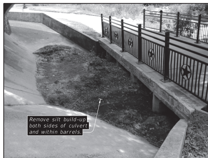
SILT REMOVAL AT CULVERT (Showing limits of silt removal at West end.)
