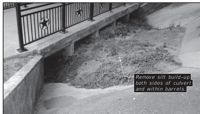
SILT REMOVAL AT CULVERT (Showing limits of silt removal at East end.)
