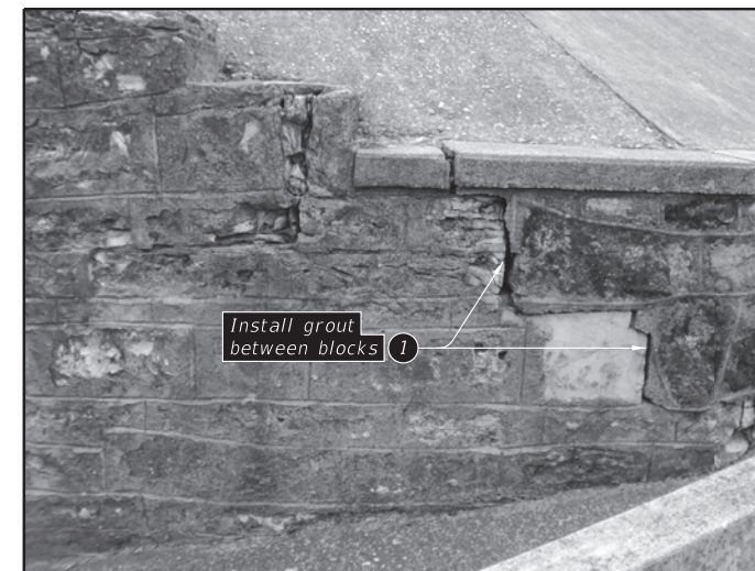
12 REPAIR LOCATION "B" (Showing limits of grout repair.) ① Furnish pre-packaged grout conforming to DMS-4675. All materials and labor for installing grout will be subsidiary to Item 432, "Riprap."
