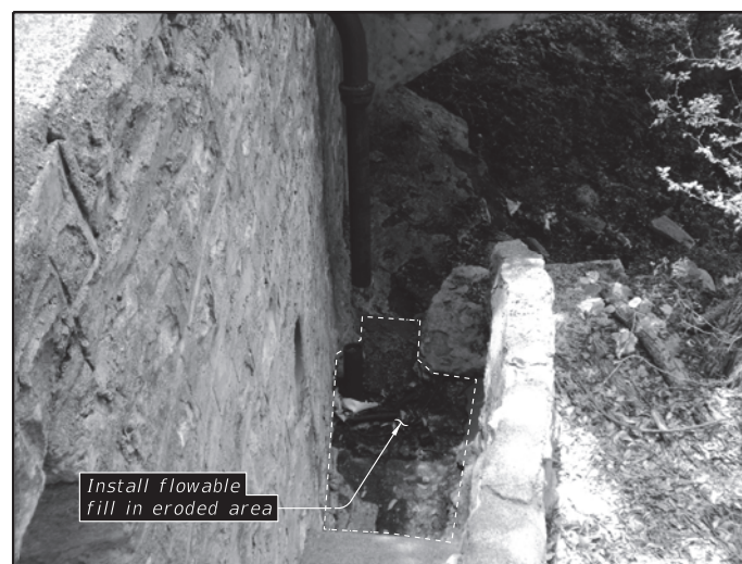
13 REPAIR LOCATION "C" (Showing limits of erosion at retaining wall.)
