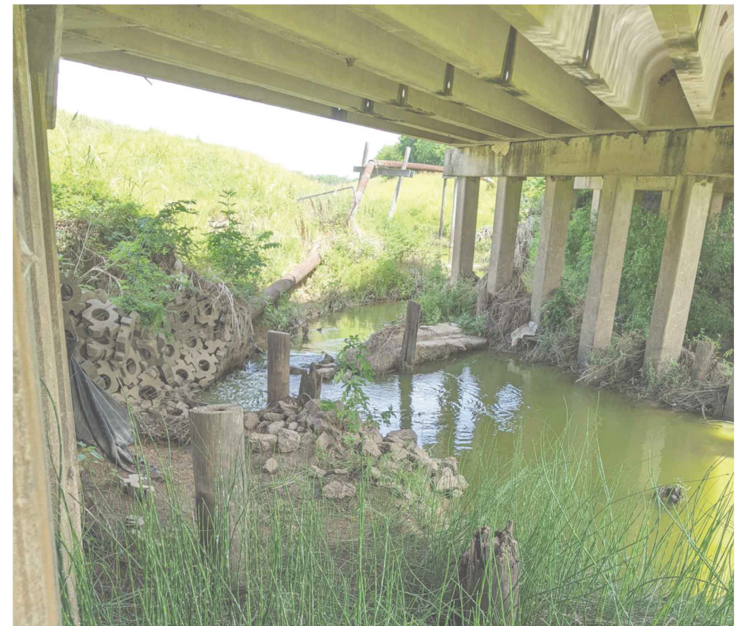
EXISTING DEBRIS IN NORTH DRAINAGE DITCH TO BE REMOVED UNDER ITEM 100
